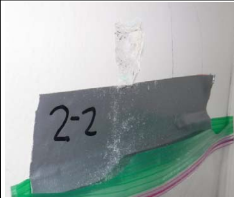
Sample 2-2, Plaster/Skim Coat, Bedroom 2
