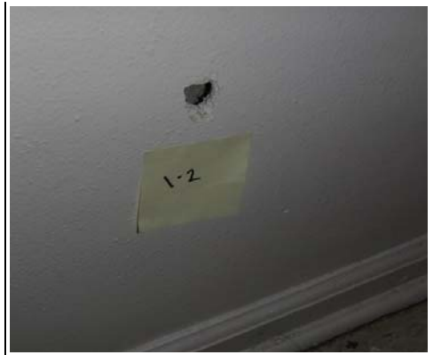
Sample 1-2, Plaster/Skim Coat, Bedroom 1
