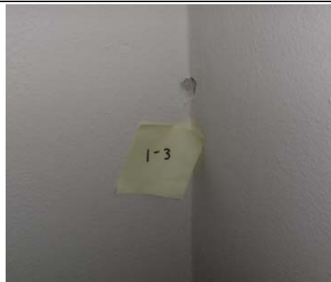
Sample 1-3, Plaster/Skim Coat, Bedroom 2
