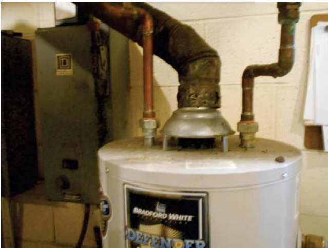
35. Leasing office mechanical, hot water heater
