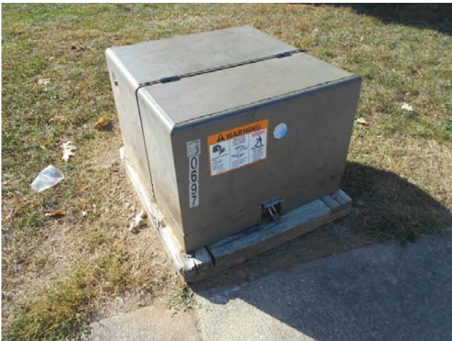
135. Pad mounted electric transformer
