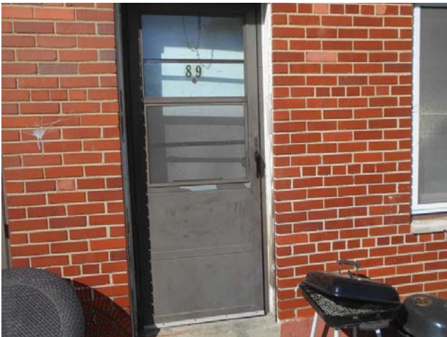
143. 86-96 Benning Place, front facade, aging doors
