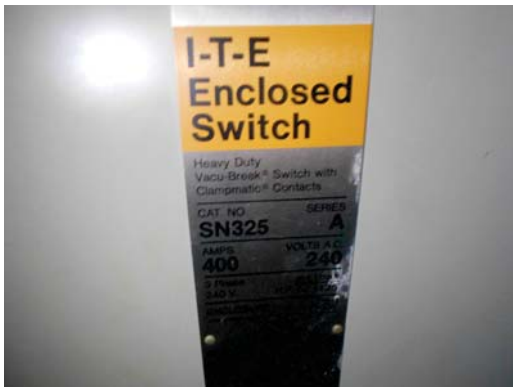
Typical Basement electrical equipment
