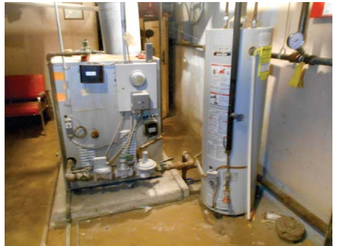
60. 900-914 Wilberforce Place, Task Force HQ, Mechanical Basement, water heater and boiler
