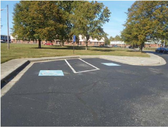
157. Handicap parking in Benning Place, no curb cut, missing 1 vertical sign
