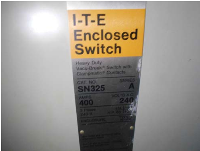
113. Typical Basement electrical equipment
