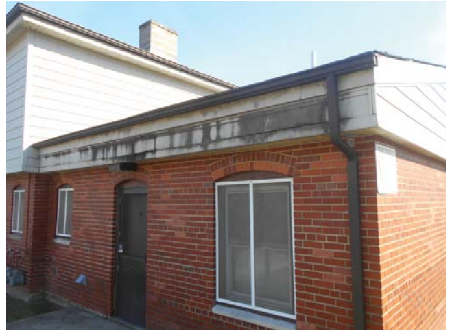
138. 86-96 Benning Place, dirt buildup on soffit
