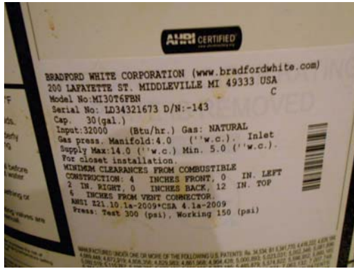
Leasing office mechanical, hot water heater
