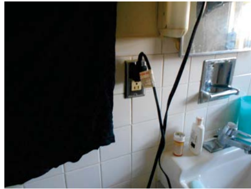
814 Oldfield Avenue, 1bed/1bath, ground floor unit - Bathroom GFCI
