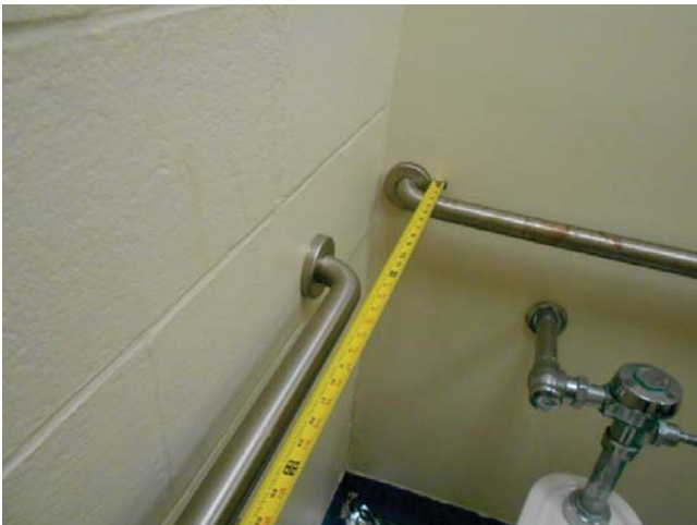
11. Leasing office public restroom, side grab bar
