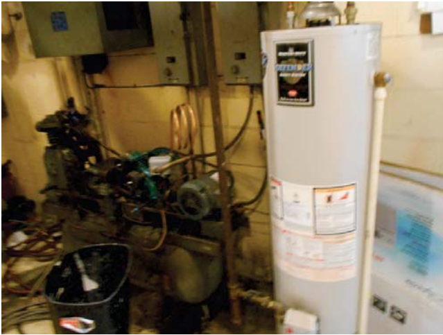
33. Leasing office mechanical, hot water heater
