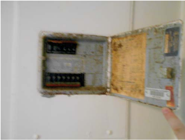
61. 82 Bragg Place, 2bed/1bath, Townhouse unit - Stab-Lok electrical panel
