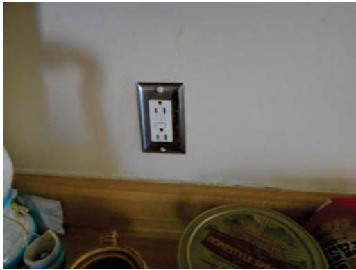
814 Oldfield Avenue, 1bed/1bath, ground floor unit - Kitchen GFCI
