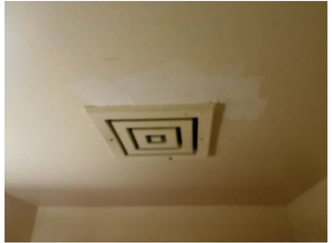
54. 1619 West Stewart Street, 2bed/1bath, Townhouse unit - Bathroom exhaust
