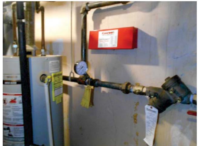
62. 900-914 Wilberforce Place, Task Force HQ, Mechanical Basement sprinkler main
