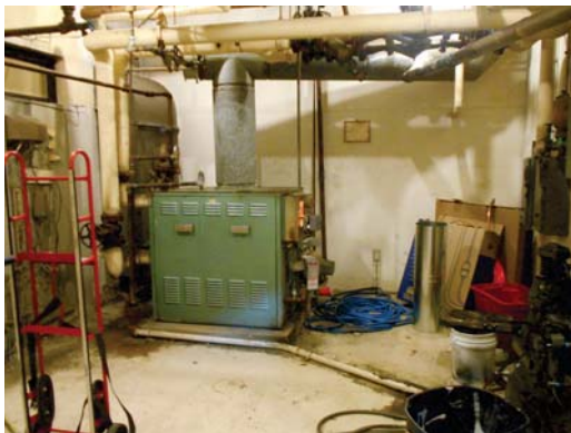
Leasing office mechanical
