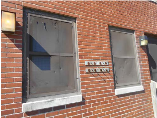
101. Typical aluminum windows with screen, typical screen in poor condition
