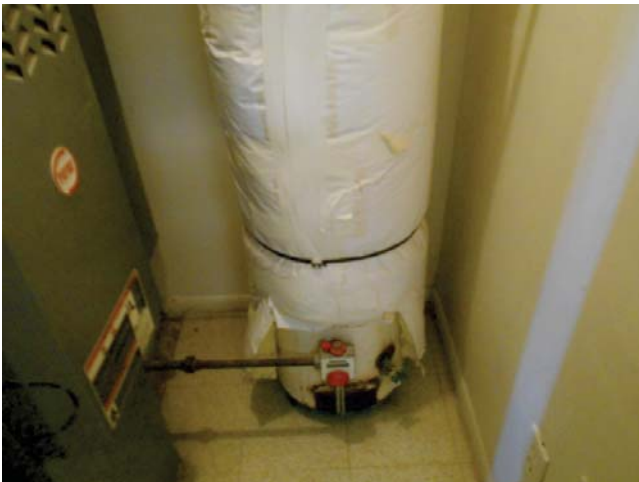
67. 82 Bragg Place, 2bed/1bath, Townhouse unit - Furnace and water heater
