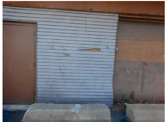
72. Garage building, damaged siding
