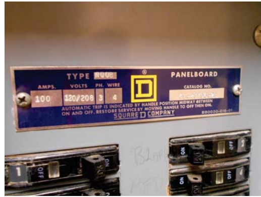
Leasing office electrical panel
