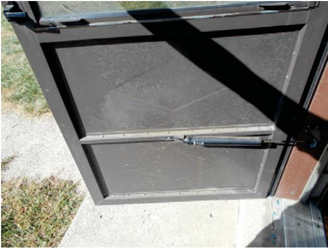
57. 1619 West Stewart Street, 2bed/1bath, Townhouse unit - Damaged door
