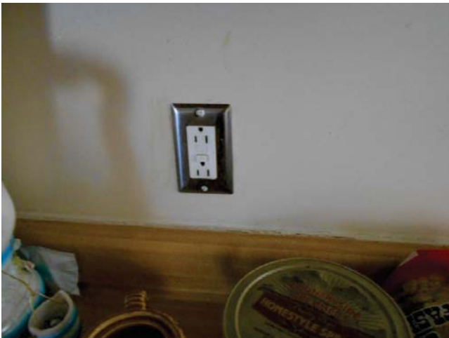
27. 814 Oldfield Avenue, 1bed/1bath, ground floor unit - Kitchen GFCI
