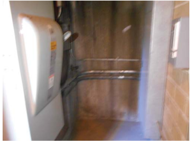
110. Typical Basement electrical equipment
