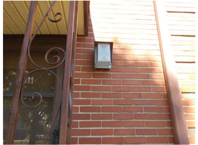
102. Typical exterior building lighting
