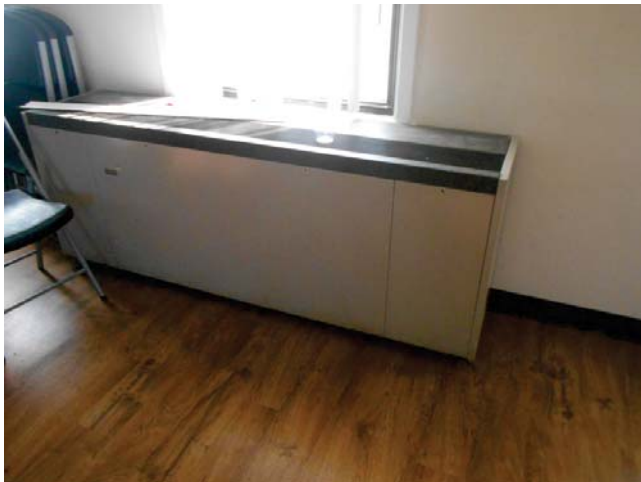
71. 900-914 Wilberforce Place, Task Force HQ, Radiator
