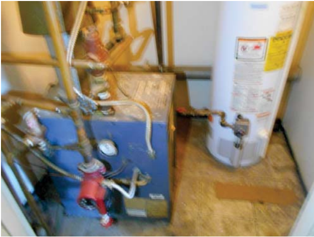
41. 1049 Carver Avenue, 2bed/1bath, Townhouse unit - Steam boiler and Water heater
