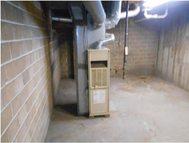
117. Typical Basement air handler
