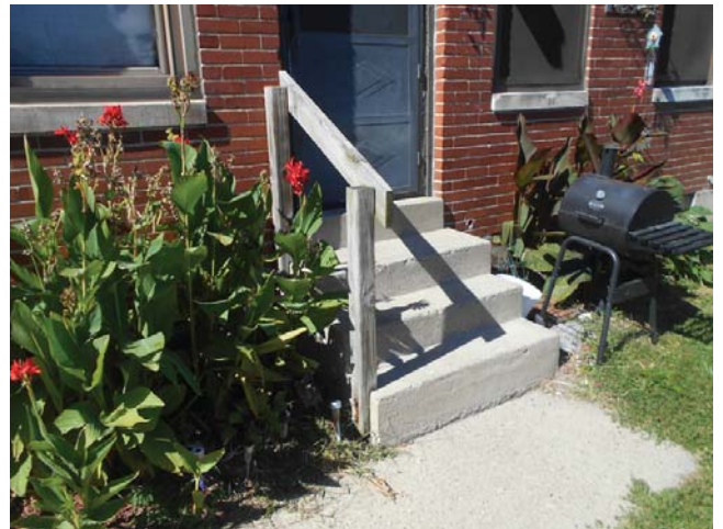
108. Typical unit entrance, wood railing, not code compliant
