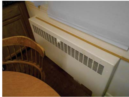
1619 West Stewart Street, 2bed/1bath, Townhouse unit - Radiator
