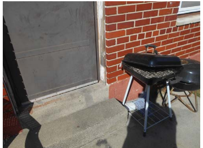
144. 86-96 Benning Place, front facade, aging door frame
