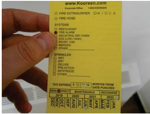
900-914 Wilberforce Place, Task Force HQ, Fire panel, Inspected June 2022
