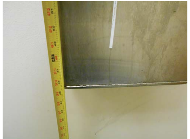
20. Leasing office public restroom, paper towel dispenser height, 48"
