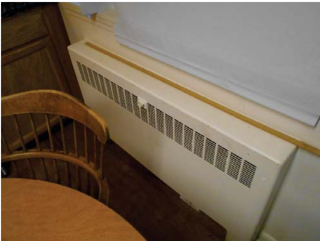
51. 1619 West Stewart Street, 2bed/1bath, Townhouse unit - Radiator
