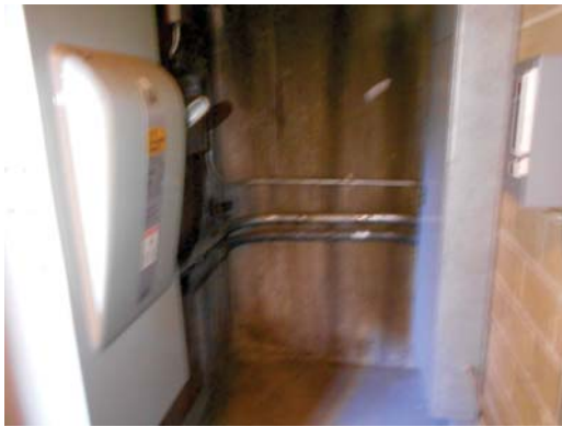
Typical Basement electrical equipment
