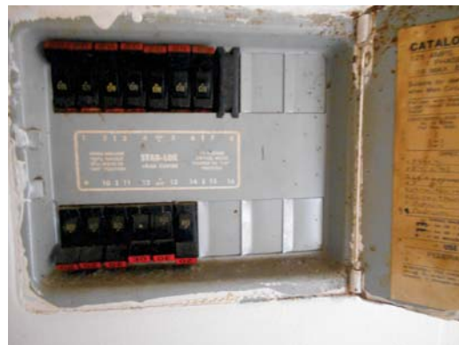
928 Custer Place, 2bed/1bath, Townhouse unit - Stab-Lok electrical panels
