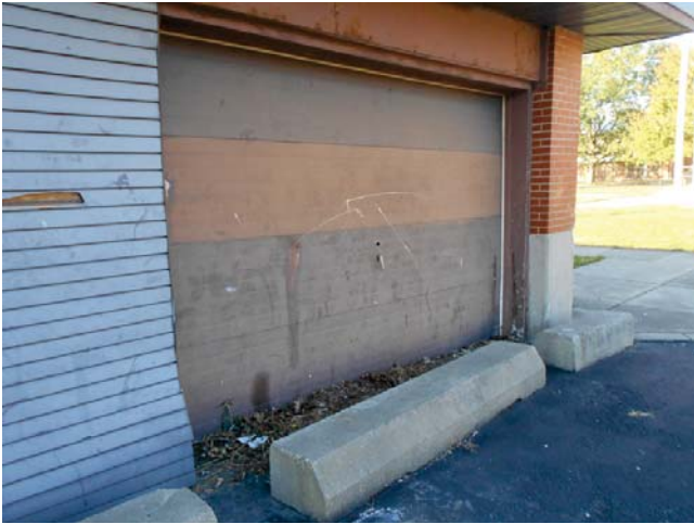
73. Garage building, damaged siding
