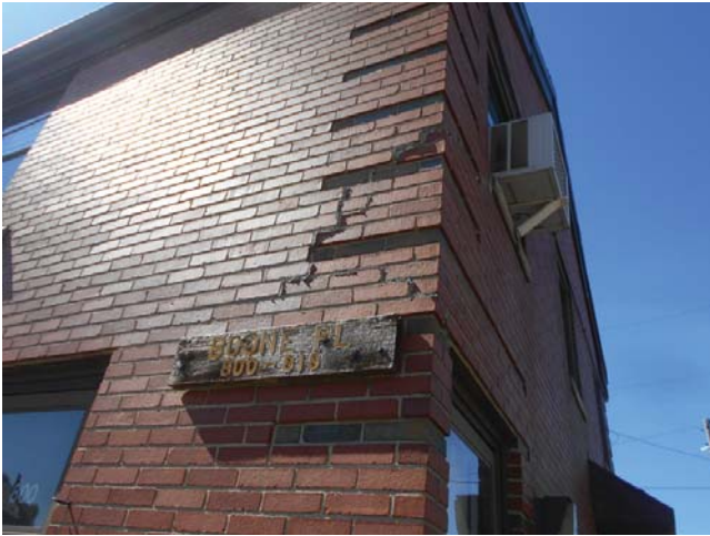
109. Boone Place, damaged facade
