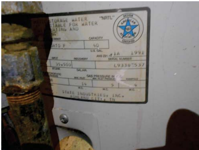
61. 900-914 Wilberforce Place, Task Force HQ, Mechanical Basement water heater
