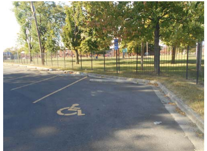
120. Handicap parking by Hughes Place, no access aisle or path to sidewalk
