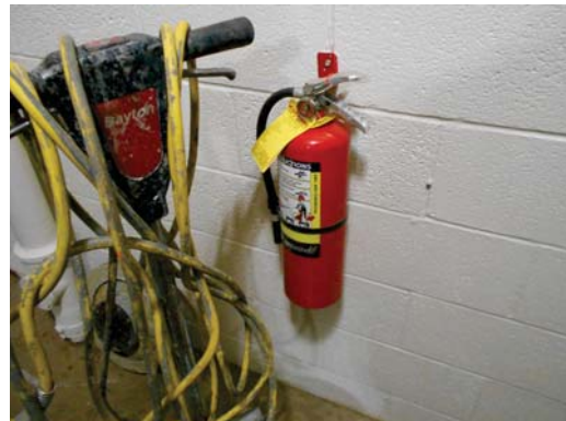
Leasing office fire extinguisher
