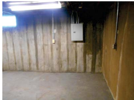
Typical Basement Electrical panel
