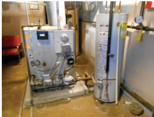
900-914 Wilberforce Place, Task Force HQ, Mechanical Basement, water heater and boiler
