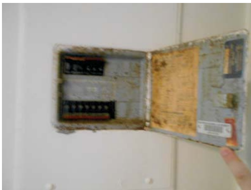
82 Bragg Place, 2bed/1bath, Townhouse unit - Stab-Lok electrical panel
