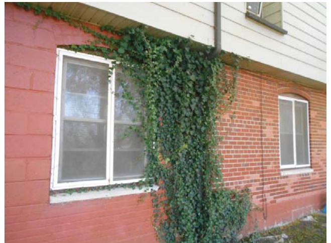
152. Foliage growing along 15-25 Benning Place, rear facade
