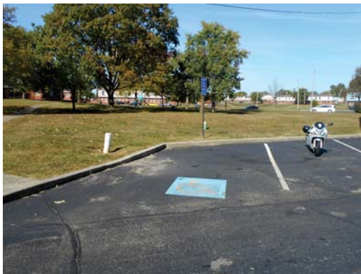
Handicap parking by Custer place, no access aisle or path to curb cut
