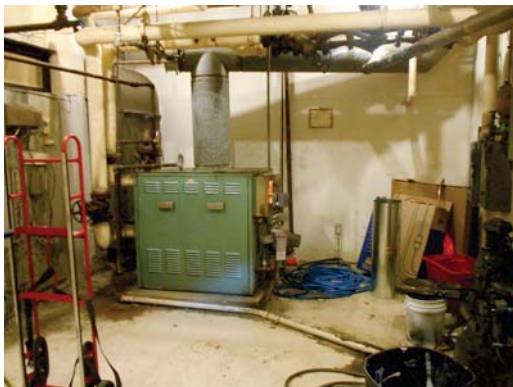
Leasing office mechanical
