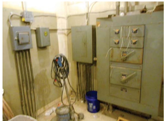
40. Leasing office mechanical, electrical equipment
