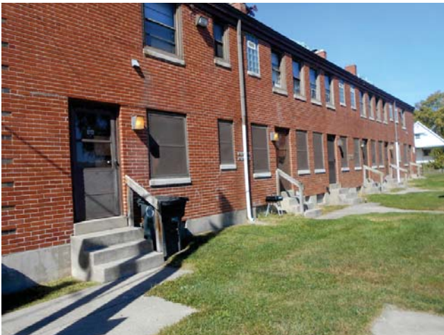
99. Typical Section 505 building, exterior steps are not code compliant, treads are not long enough and railings are not compliant
