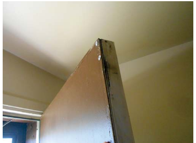
56. 1619 West Stewart Street, 2bed/1bath, Townhouse unit - Damaged door
