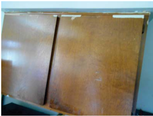
1007 Danner Avenue, 2bed/1bath, Townhouse unit - Kitchen, old cabinets
