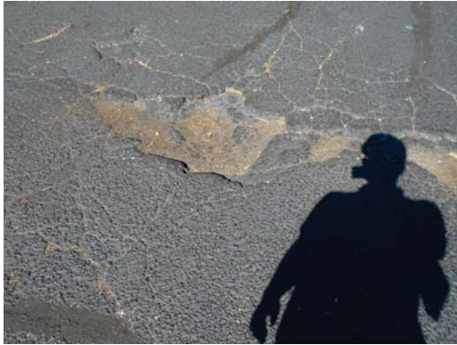
Leasing office asphalt parking lot, damaged
