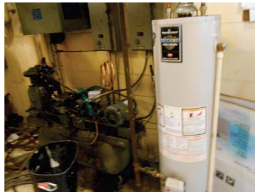
Leasing office mechanical, hot water heater
