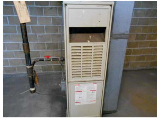
Typical Basement air handler
