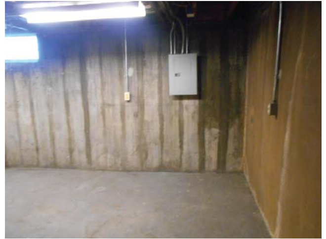
118. Typical Basement Electrical panel
