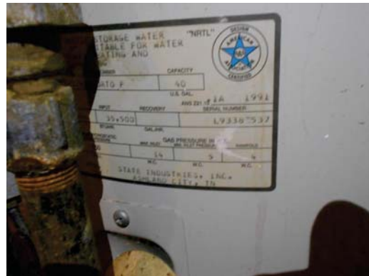
900-914 Wilberforce Place, Task Force HQ, Mechanical Basement water heater
