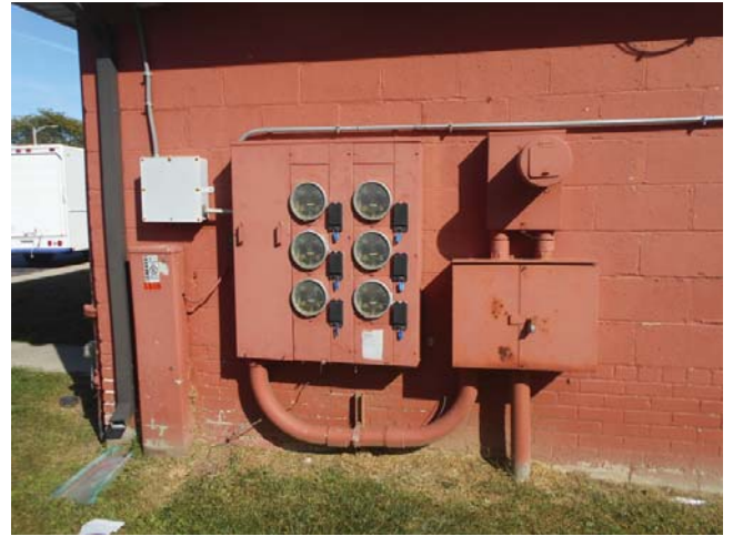
146. 921-935 Custer Place, electrical meter
