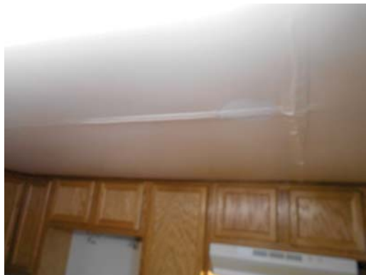
1619 West Stewart Street, 2bed/1bath, Townhouse unit - Kitchen ceiling, leak from above bathroom
