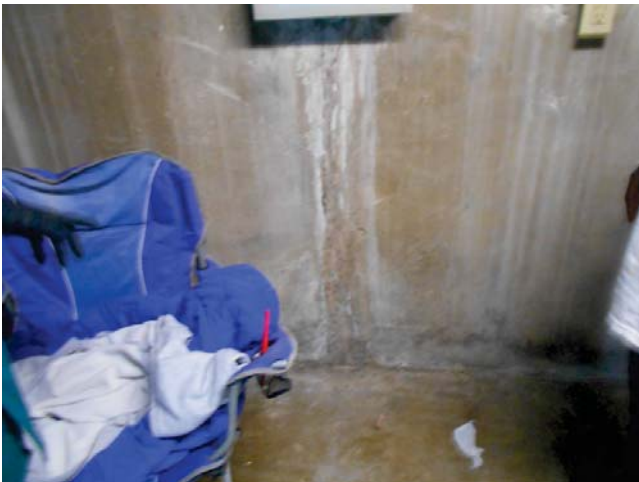
79. 1806 Germantown Street, 2bed/1bath, Townhouse unit - Basement, water damage by electrical panel
