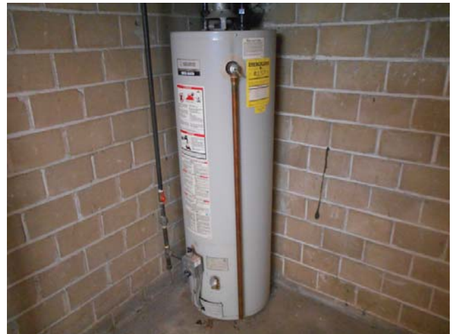
114. Typical Basement water heater
