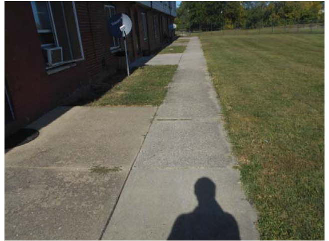
150. Typical sidewalk condition
