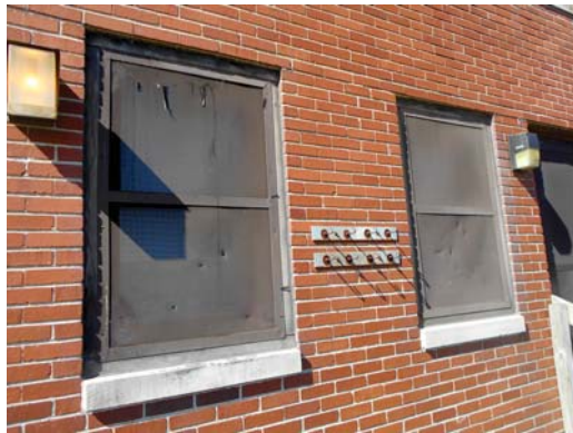
Typical aluminum windows with screen, typical screen in poor condition
