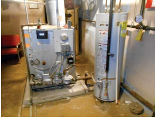
900-914 Wilberforce Place, Task Force HQ, Mechanical Basement, water heater and boiler
