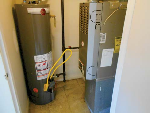
77. 928 Custer Place, 2bed/1bath, Townhouse unit - Furnace and water heater, newer
