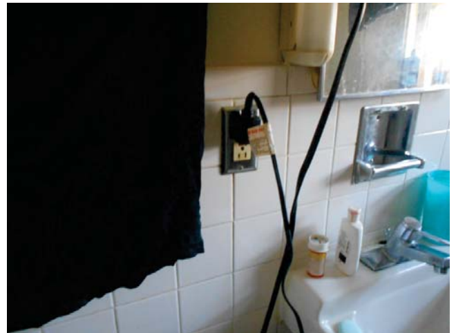
28. 814 Oldfield Avenue, 1bed/1bath, ground floor unit - Bathroom GFCI
