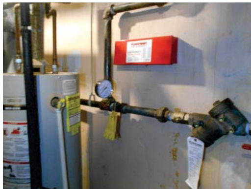
900-914 Wilberforce Place, Task Force HQ, Mechanical Basement sprinkler main
