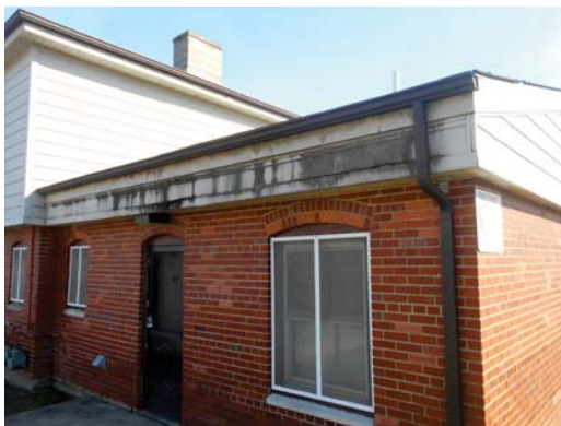
86-96 Benning Place, dirt buildup on soffit
