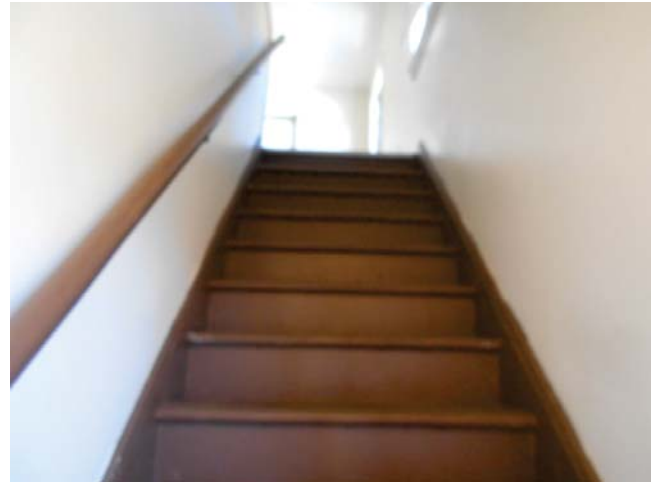
2. 818 Oldfield Avenue, 1bed/1bath, upstairs unit, vacant - Stairs
