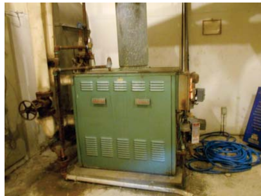
Leasing office mechanical, boiler
