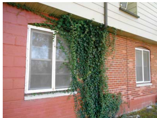
Foliage growing along 15-25 Benning Place, rear facade
