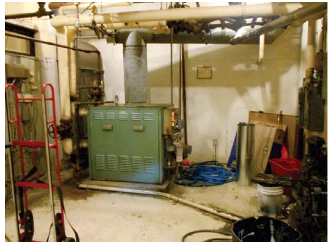
32. Leasing office mechanical
