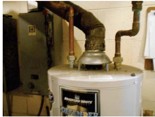
Leasing office mechanical, hot water heater
