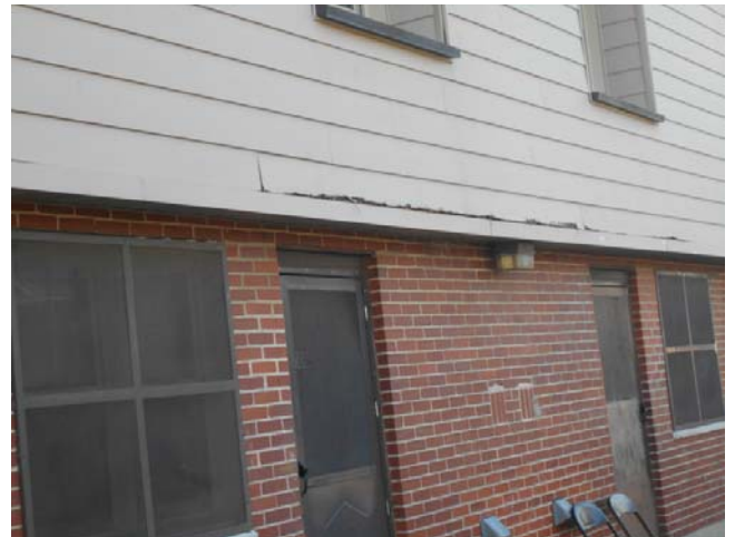
128. Typical section 502 building, aging/damaged siding
