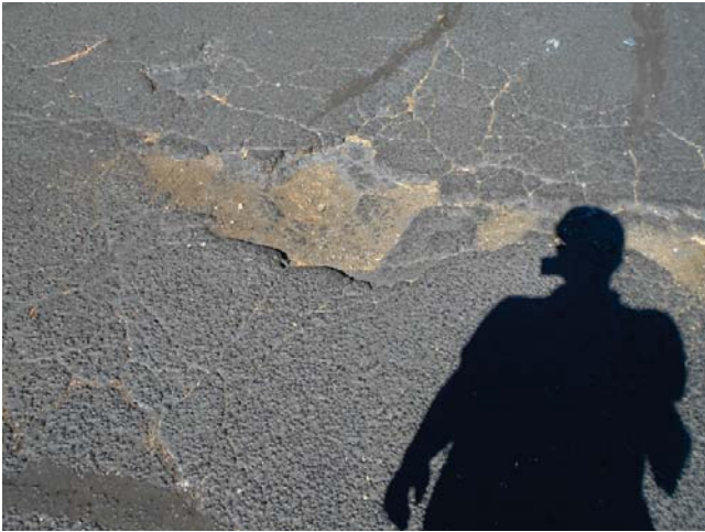
77. Leasing office asphalt parking lot, damaged
