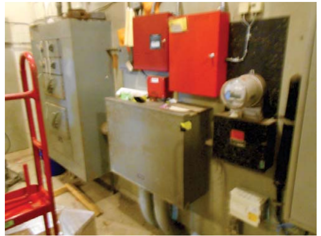
38. Leasing office mechanical, boiler electrical and fire panel
