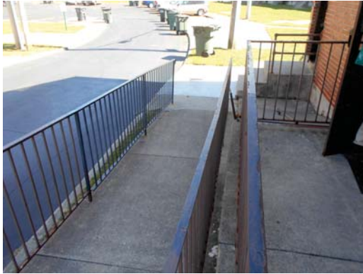
814 Oldfield Avenue, 1bed/1bath, ground floor unit, vacant - Concrete ramp to unit entrance
