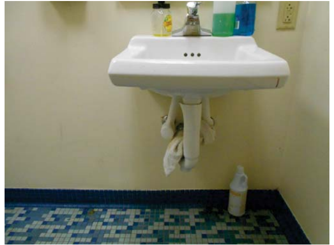
18. Leasing office public restroom, sink scald abrasion protection
