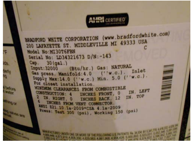
34. Leasing office mechanical, hot water heater
