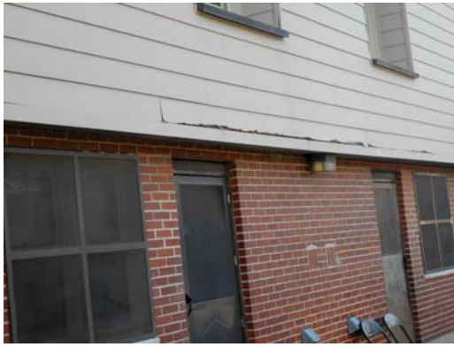
Typical section 502 building, aging/damaged siding
