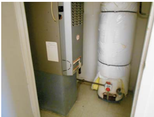
82 Bragg Place, 2bed/1bath, Townhouse unit - Furnace and water heater
