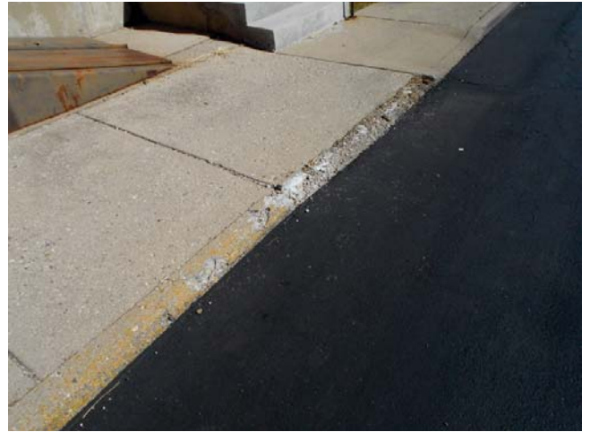
98. Concrete curb by building C-1 damaged
