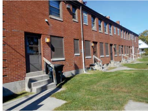
Typical Section 505 building, exterior steps are not code compliant, treads are not long enough and railings are not compliant
