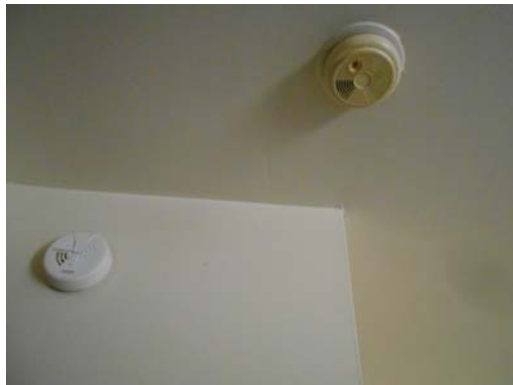
818 Oldfield Avenue, 1bed/1bath, upstairs unit, vacant - Living area smoke detector and CO2 detector
