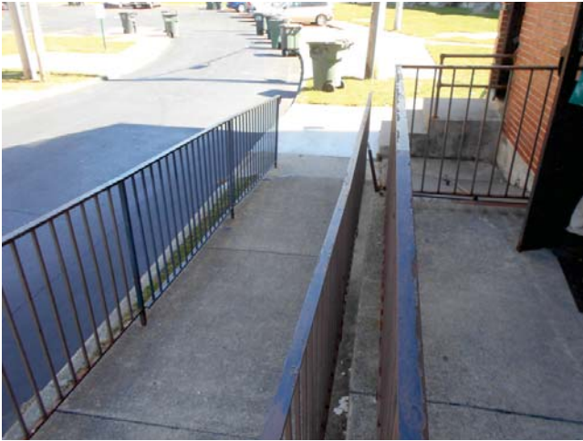
17. 814 Oldfield Avenue, 1bed/1bath, ground floor unit, vacant - Concrete ramp to unit entrance
