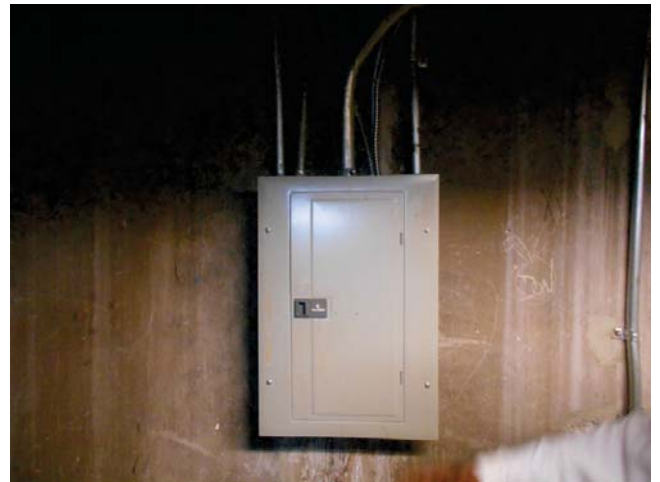
80. 1806 Germantown Street, 2bed/1bath, Townhouse unit - Basement, water damage by electrical panel
