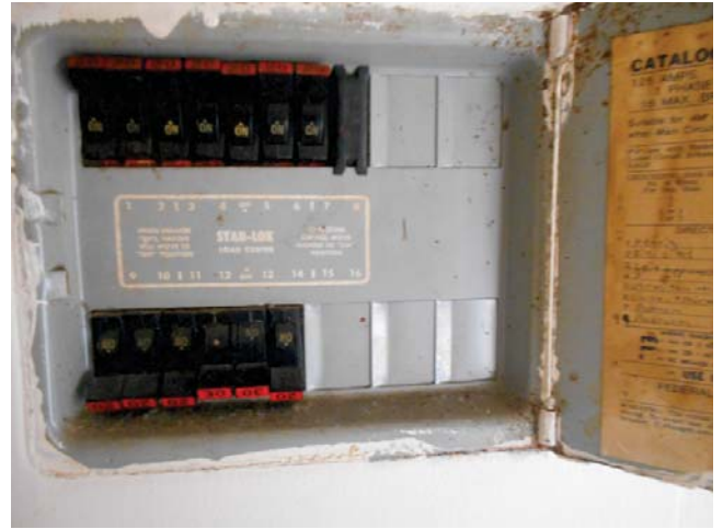
70. 928 Custer Place, 2bed/1bath, Townhouse unit - Stab-Lok electrical panels
