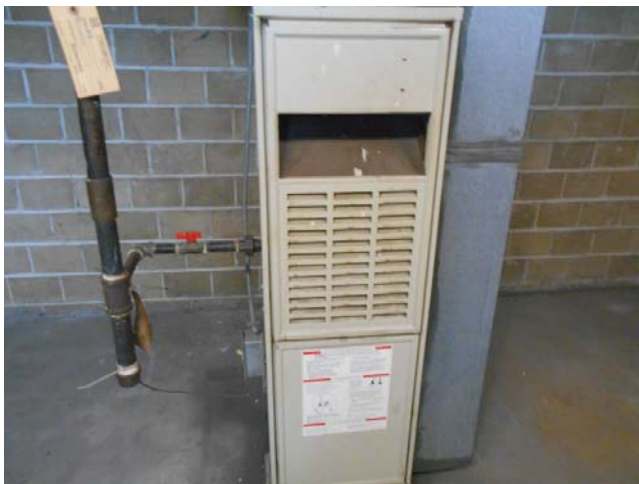
115. Typical Basement air handler
