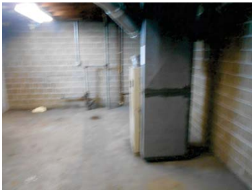
Typical Basement electrical equipment
