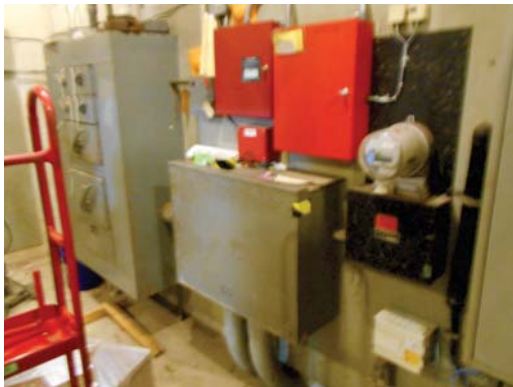
Leasing office mechanical, boiler electrical and fire panel
