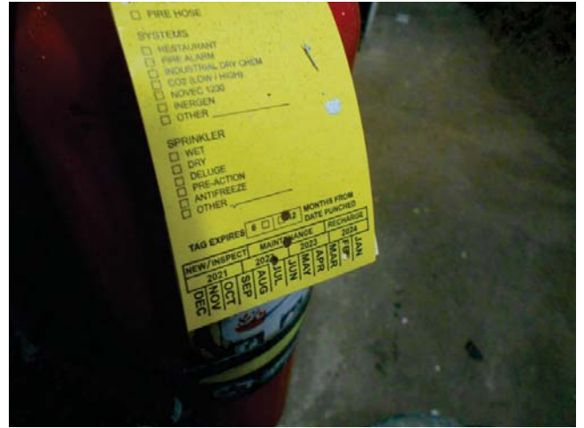
30. Leasing office fire extinguisher, inspected February 2022
