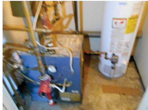
1049 Carver Avenue, 2bed/1bath, Townhouse unit - Steam boiler and Water heater
