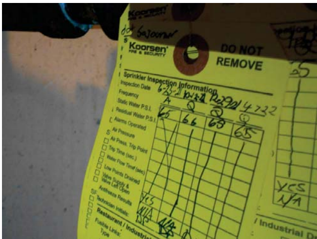
63. 900-914 Wilberforce Place Task Force HQ, Mechanical Basement sprinkler main, inspected 4/7/2022
