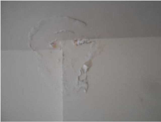
37. 1007 Danner Avenue, 2bed/1bath, Townhouse unit - Bathroom, damaged drywall
