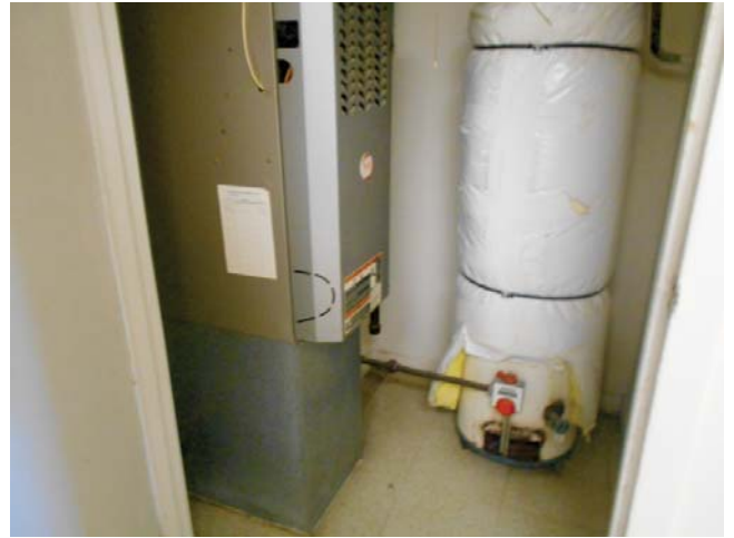
66. 82 Bragg Place, 2bed/1bath, Townhouse unit - Furnace and water heater
