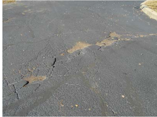
Leasing office asphalt parking lot, damaged
