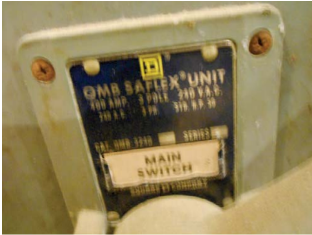
41. Leasing office mechanical, electrical equipment
