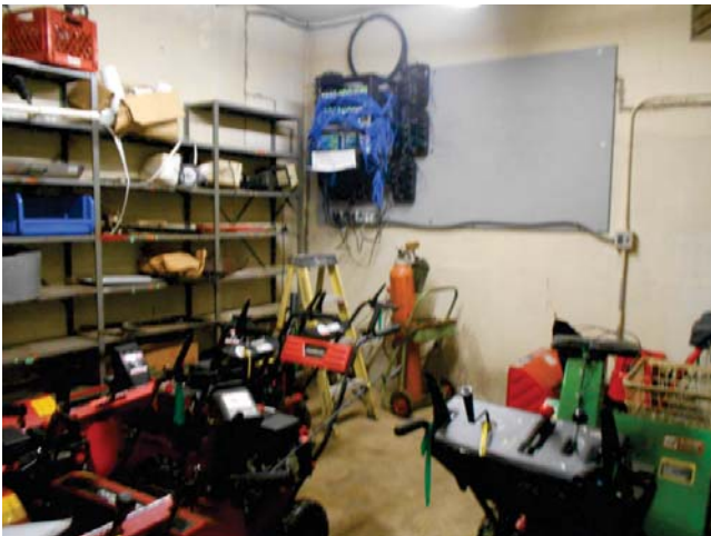
31. Leasing office mechanical
