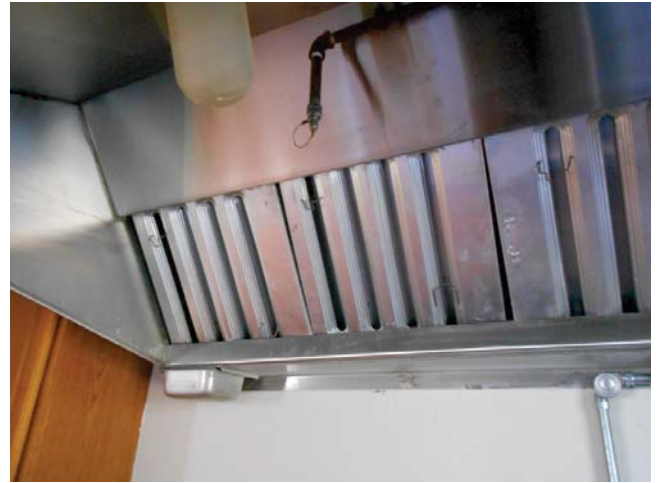
70. 900-914 Wilberforce Place, Task Force HQ, 2nd floor Main room kitchen stove fire suppression system
