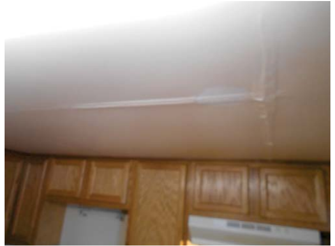
50. 1619 West Stewart Street, 2bed/1bath, Townhouse unit - Kitchen ceiling, leak from above bathroom
