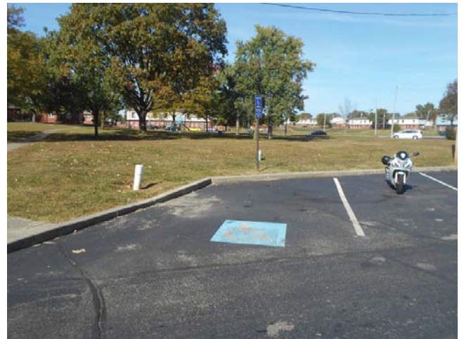
148. Handicap parking by Custer place, no access aisle or path to curb cut
