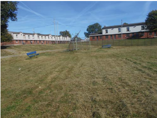
155. Damaged chain-link fencing in Gillespie Park
