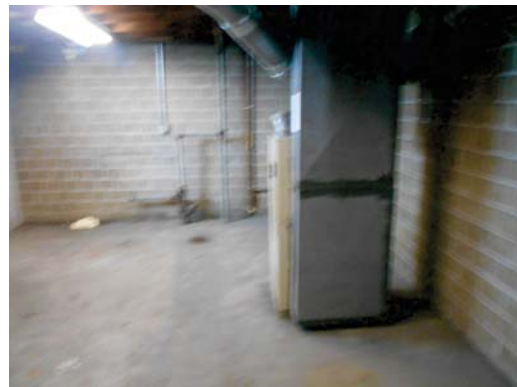
Typical Basement electrical equipment
