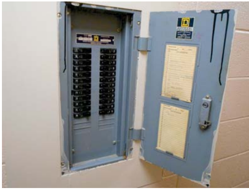
Leasing office electrical panel
