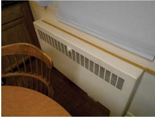
1619 West Stewart Street, 2bed/1bath, Townhouse unit - Radiator
