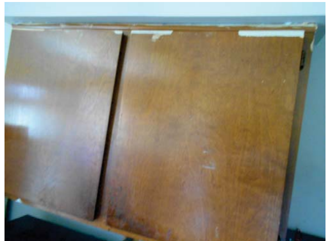
32. 1007 Danner Avenue, 2bed/1bath, Townhouse unit - Kitchen, old cabinets
