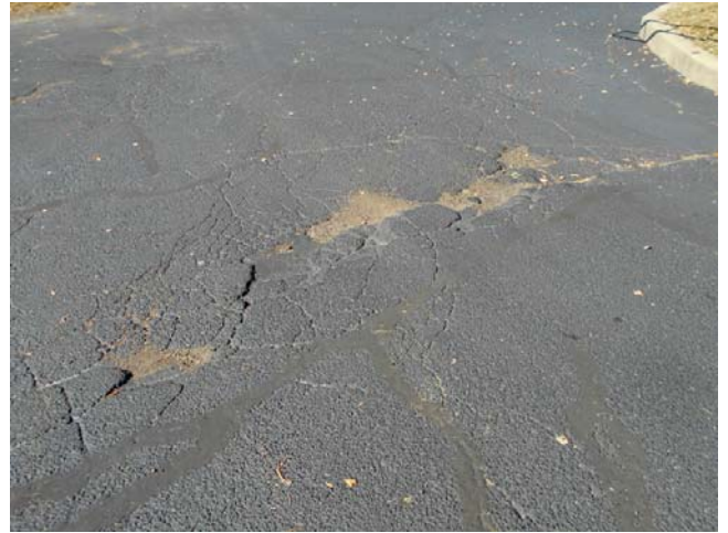
78. Leasing office asphalt parking lot, damaged
