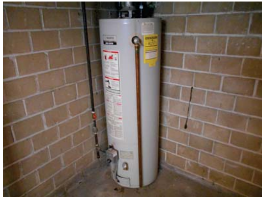
Typical Basement water heater
