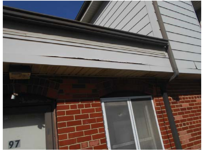
142. 86-96 Benning Place, front facade, aging siding
