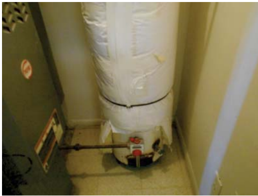
82 Bragg Place, 2bed/1bath, Townhouse unit - Furnace and water heater
