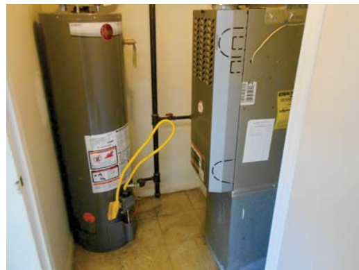
928 Custer Place, 2bed/1bath, Townhouse unit - Furnace and water heater, newer
