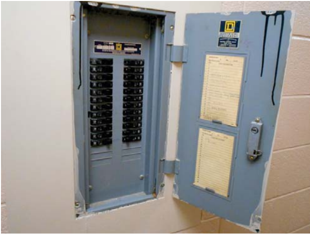
21. Leasing office electrical panel
