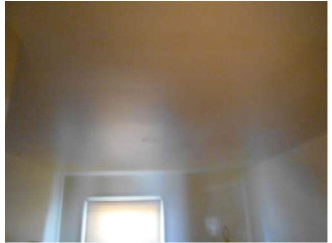
26. 814 Oldfield Avenue, 1bed/1bath, ground floor unit - Bedroom ceiling, no smoke detector
