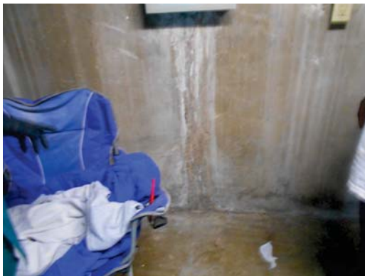
1806 Germantown Street, 2bed/1bath, Townhouse unit - Basement, water damage by electrical panel
