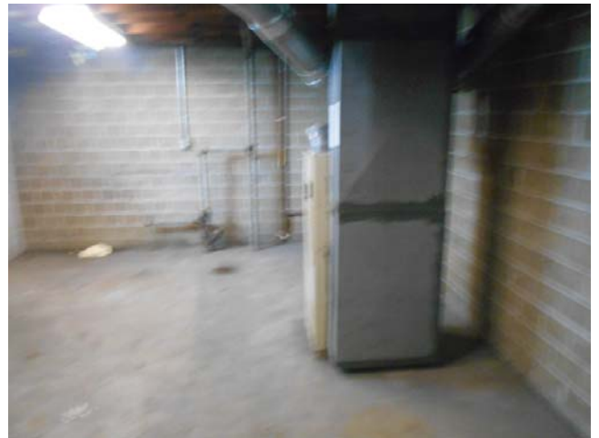
112. Typical Basement electrical equipment
