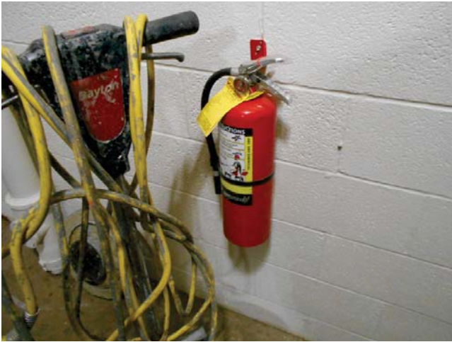
29. Leasing office fire extinguisher
