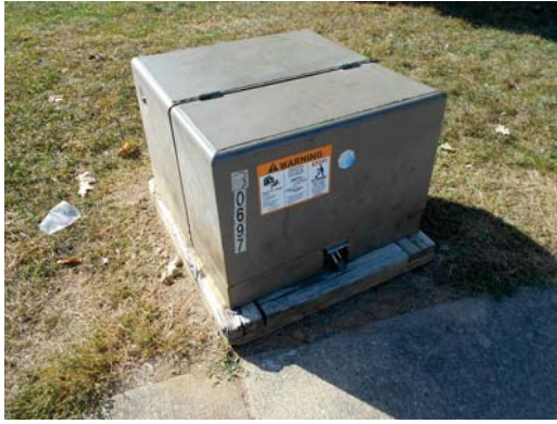
Pad mounted electric transformer
