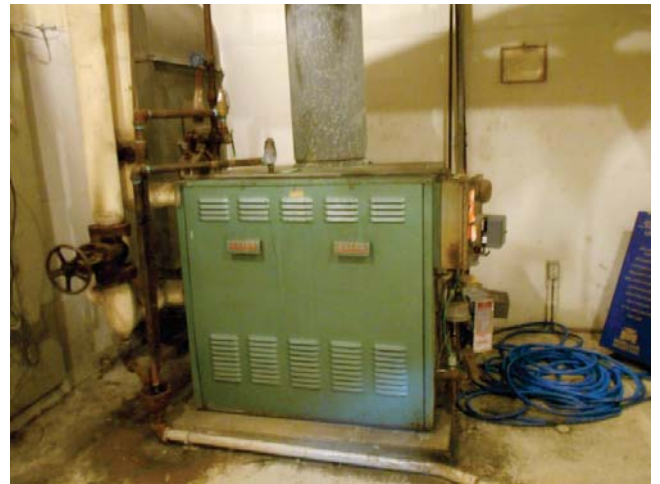
36. Leasing office mechanical, boiler
