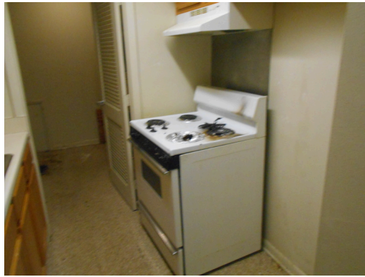
Unit E - 1bed/1bath, vacant - Kitchen stove and overhead, no wall shield
