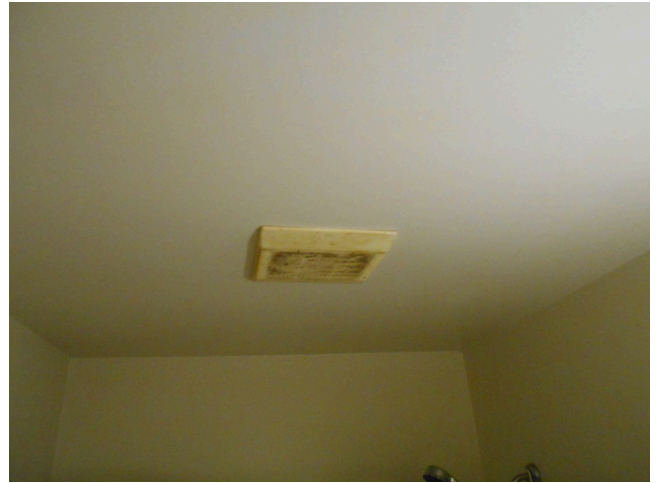
58. Unit F - 1bed/1bath - Bathroom ceiling
