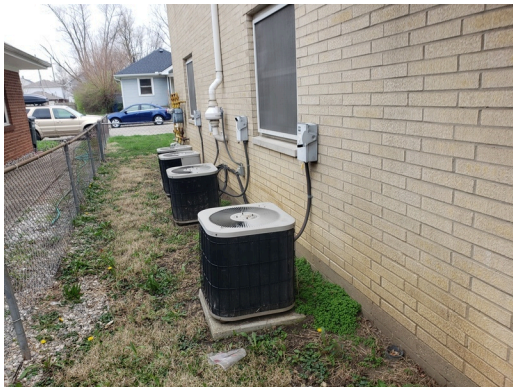
A/C condenser units
