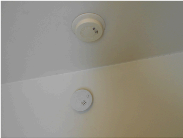
9. Stairwell smoke detector
