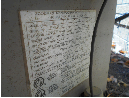
A/C condenser units
