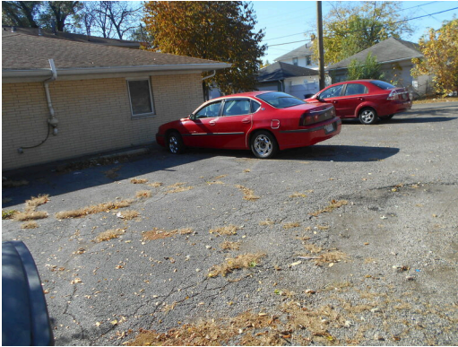
Asphalt parking lot, cracked and faded lines
