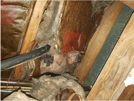
Update-Unit A - 1bed/1bath, vacant -Laundry Room- Water damage ceiling
