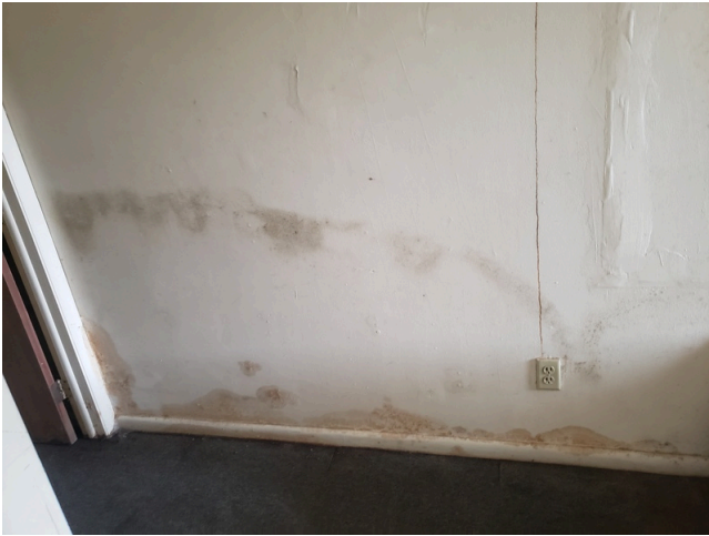
45. Update- Unit A - 1bed/1bath, vacant - Living Room- Mold/ water damage
