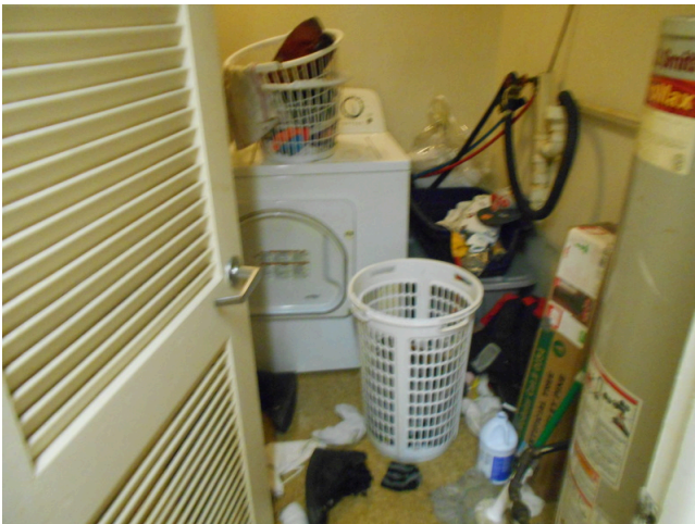
43. Unit F - 1bed/1bath - Mechanical closet
