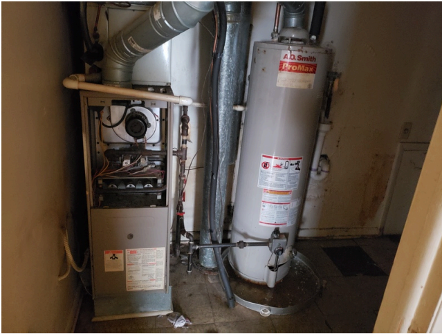
53. Update- Unit B - 1bed/1bath, vacant - 2nd Floor- Furnace and Water Heater
