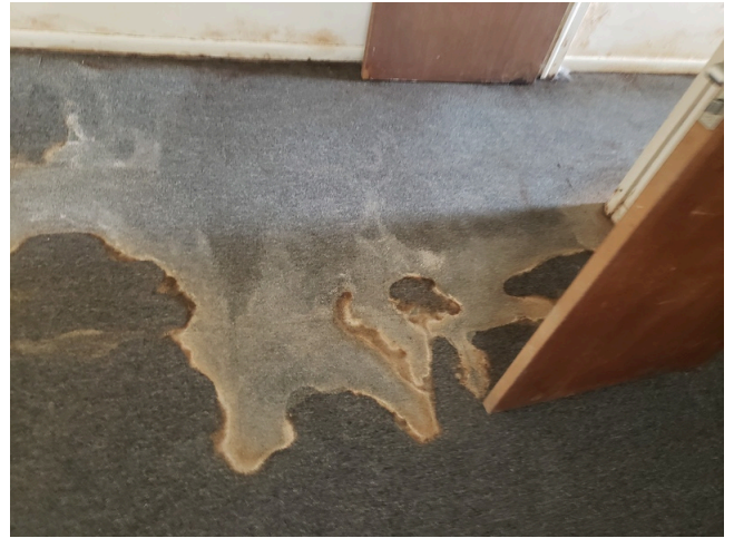
18. Update- Unit A - 1bed/1bath, vacant -Bedroom- Replace water damaged carpet
