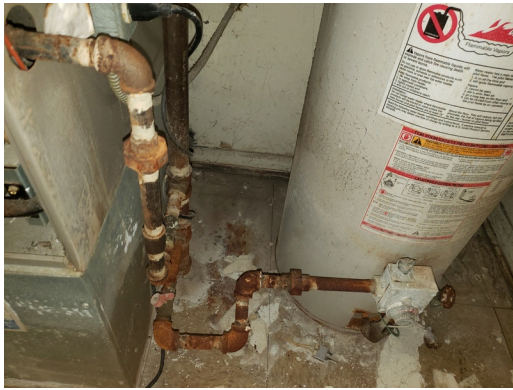
Update-Unit A - 1bed/1bath, vacant -Laundry Room- Furnace- Rusty Pipes
