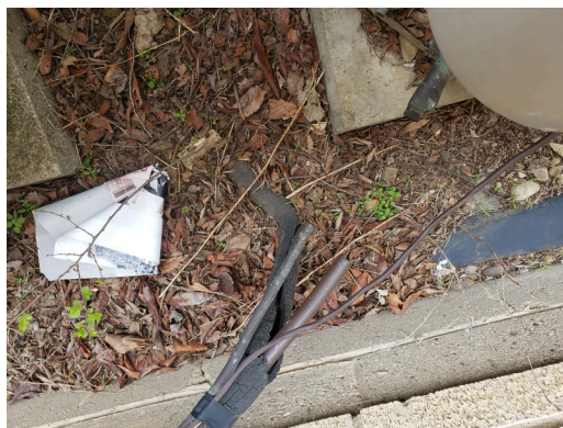
A/C units, damaged A/C condenser line set
