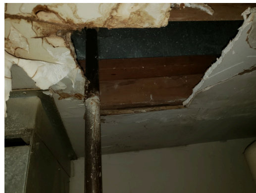
Update-Unit A - 1bed/1bath, vacant -Laundry Room- Hot water heater piping
