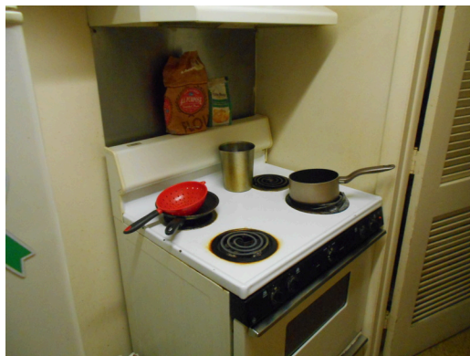
Unit F - 1bed/1bath - Kitchen range, no wall shield
