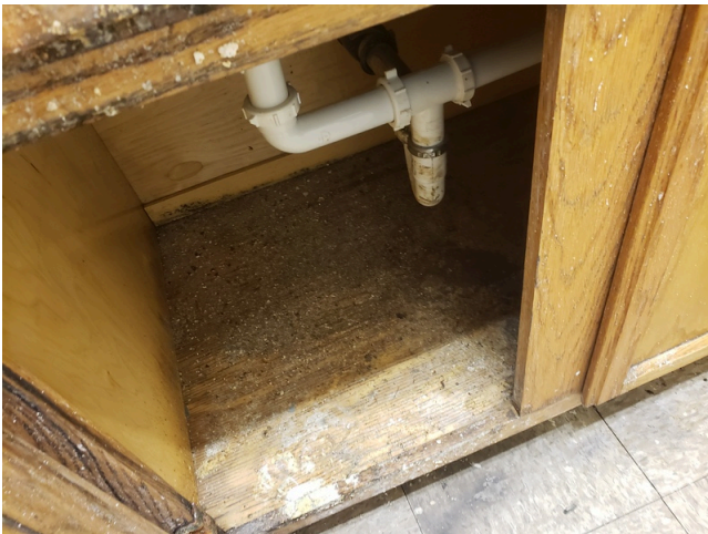
79. Update- Unit D - 1bed/1bath, vacant - Kitchen- Cabinet Older
