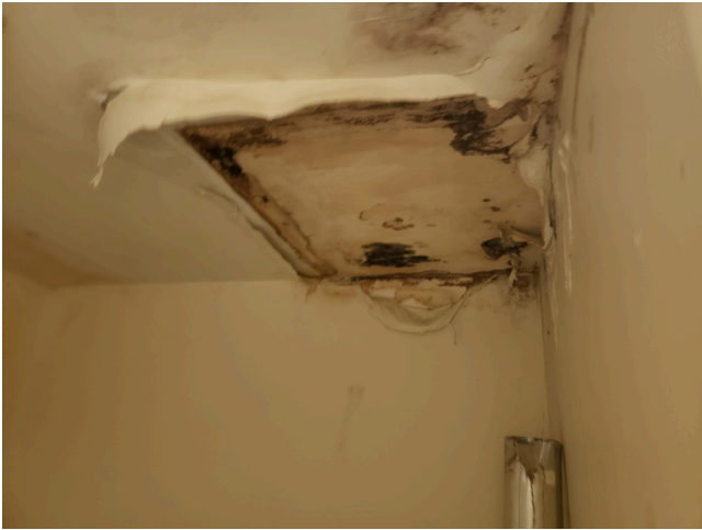
49. Update- Unit A - 1bed/1bath, vacant -Laundry Room- Water damage and mold
