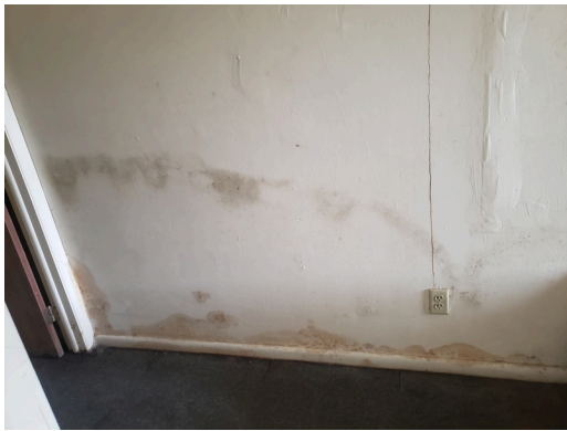
Update- Unit A - 1bed/1bath, vacant - Living Room- Mold/ water damage
