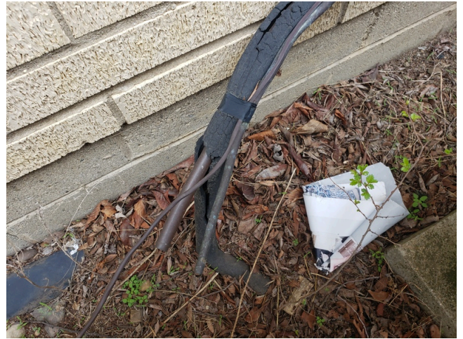
54. A/C units, damaged A/C insulation line
