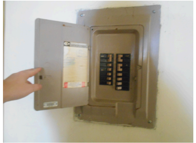
10. Unit D - 1bed/1bath, vacant - Electrical panel, older model
