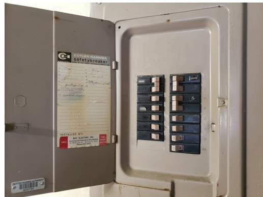
Update- Unit D - 1bed/1bath, vacant - Electrical Panel
