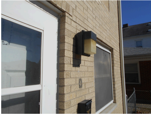
Building mounted exterior lighting
