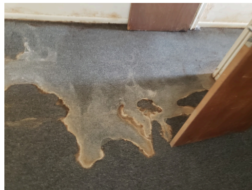
Update- Unit A - 1bed/1bath, vacant -Bedroom- Replace water damaged carpet
