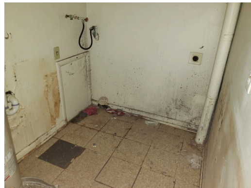
Update- Unit B - 1bed/1bath, vacant - 2nd Floor- Laundry Room- Damaged VCT flooring
