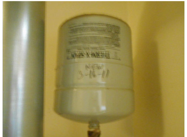
52. Unit F - 1bed/1bath - Mechanical closet water heater expansion tank
