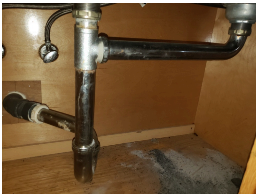
Update- Unit B - 1bed/1bath, vacant - 2nd Floor- Kitchen Pipes
