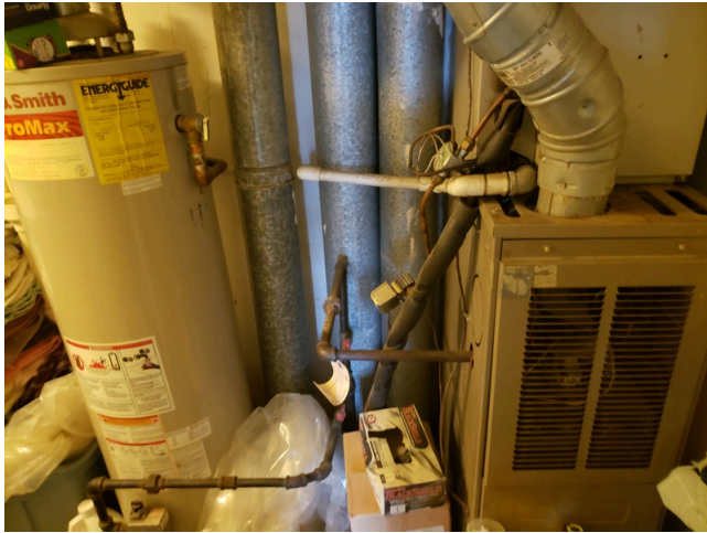
29. Update-Unit C - 1bed/1bath, occupied - 2nd Floor- Furnace and water heater
