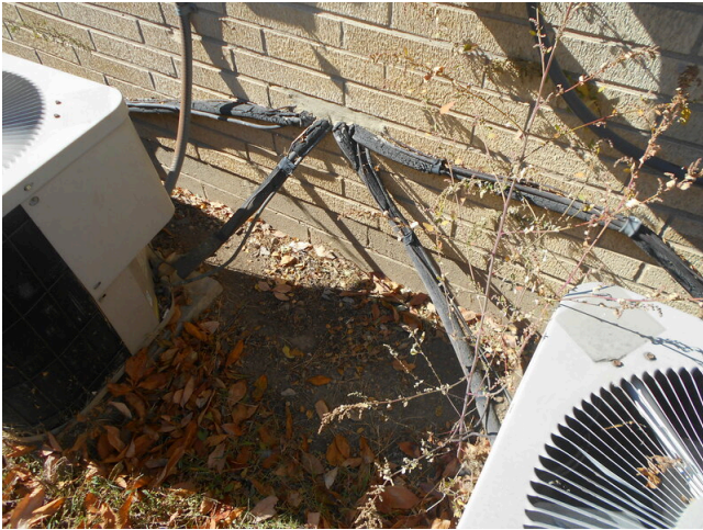
29. A/C units, damaged A/C insulation line
