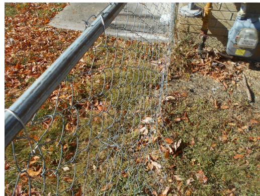
Damaged chain link fencing
