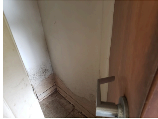
Update- Unit A - 1bed/1bath, vacant - Living Room- Closet- Mold
