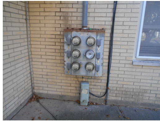
Electrical meters, dated infrastructure
