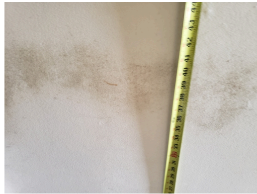
Update- Unit A - 1bed/1bath, vacant - Living Room- Mold/ water damage
