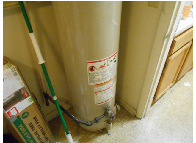
50. Unit F - 1bed/1bath - Mechanical closet water heater
