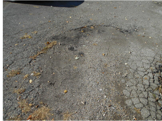
Asphalt parking lot, cracked and faded lines
