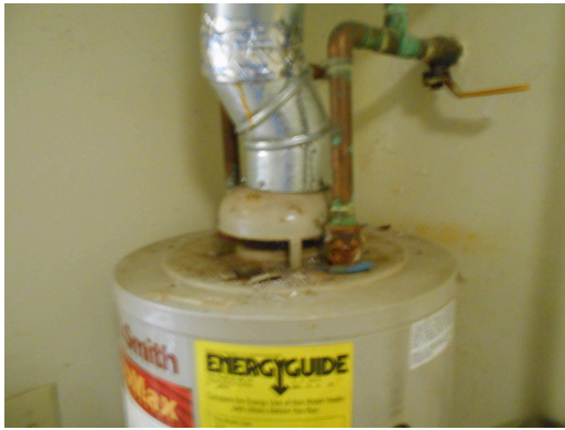
Unit E - 1bed/1bath, vacant - Mechanical closet water heater
