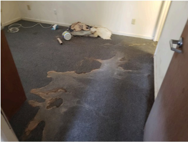
17. Update- Unit A - 1bed/1bath, vacant -Bedroom- Replace water damaged carpet
