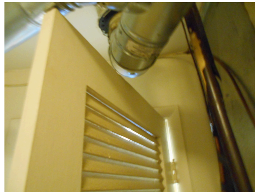
Unit F - 1bed/1bath - Mechanical closet furnace vent, hits with door swing
