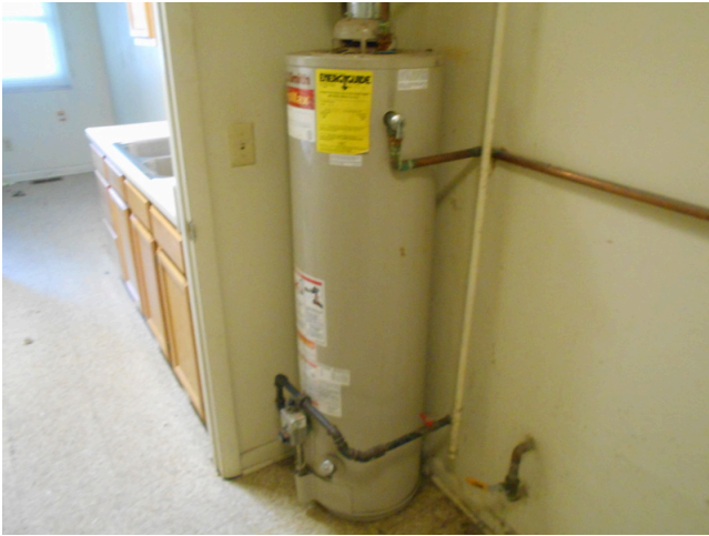
29. Unit E - 1bed/1bath, vacant - Mechanical closet water heater
