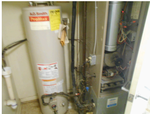
Unit D - 1bed/1bath, vacant - Mechanical closet, older water heater and furnace
