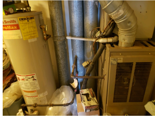
Update-Unit C - 1bed/1bath, occupied - 2nd Floor- Furnace and water heater
