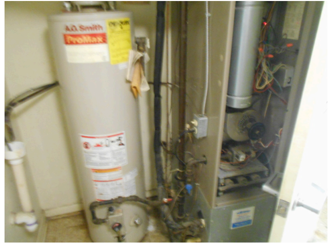
6. Unit D - 1bed/1bath, vacant - Mechanical closet, older water heater and furnace
