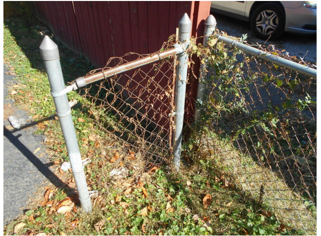
34. Chain link fencing, damaged
