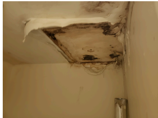
Update- Unit A - 1bed/1bath, vacant -Laundry Room- Water damage and mold
