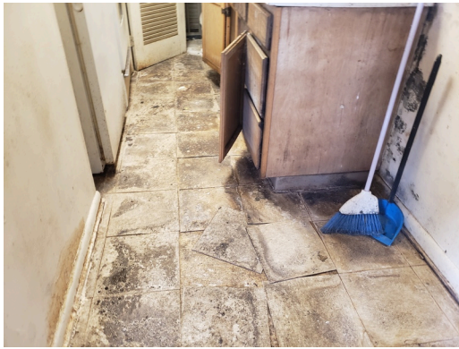
Update- Unit A - 1bed/1bath, vacant - Dining Room- Replace damaged VCT
