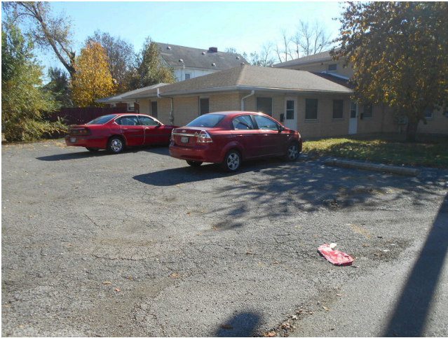
37. Asphalt parking lot, cracked and faded lines
