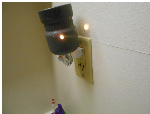
Unit F - 1bed/1bath - Bathroom GFCI
