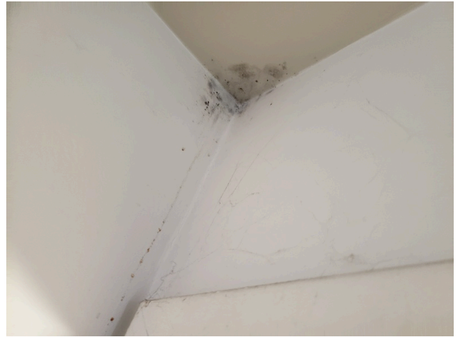
2. Update- Unit A - 1bed/1bath, vacant - Bathroom- Ceiling mold
