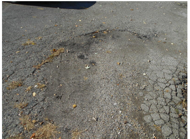
36. Asphalt parking lot, cracked and faded lines
