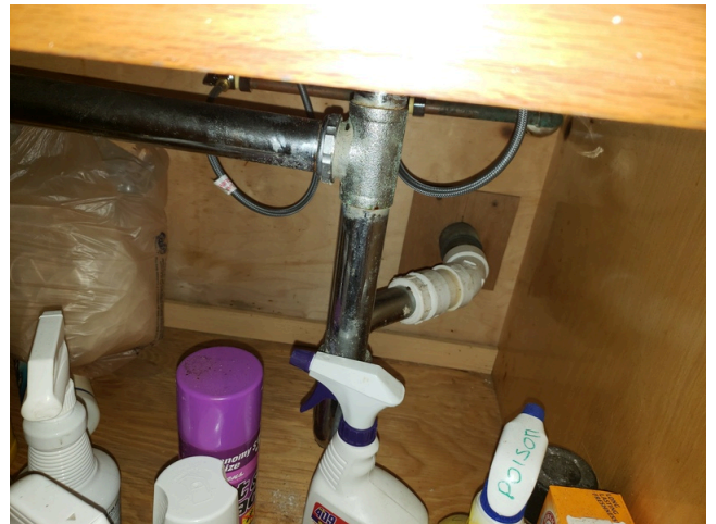
68. Update- Unit C - 1bed/1bath, vacant - 2nd Floor- Bathroom- Vanity
