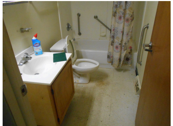
12. Unit D - 1bed/1bath, vacant - Bathroom, older finishes and accessories
