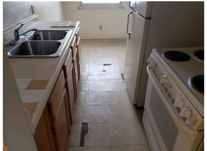
56. Update- Unit B - 1bed/1bath, vacant - 2nd Floor- Kitchen- Damaged Flooring
