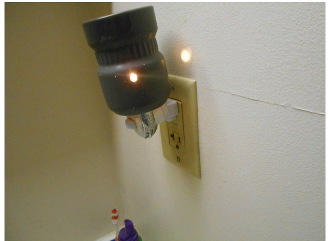
56. Unit F - 1bed/1bath - Bathroom GFCI
