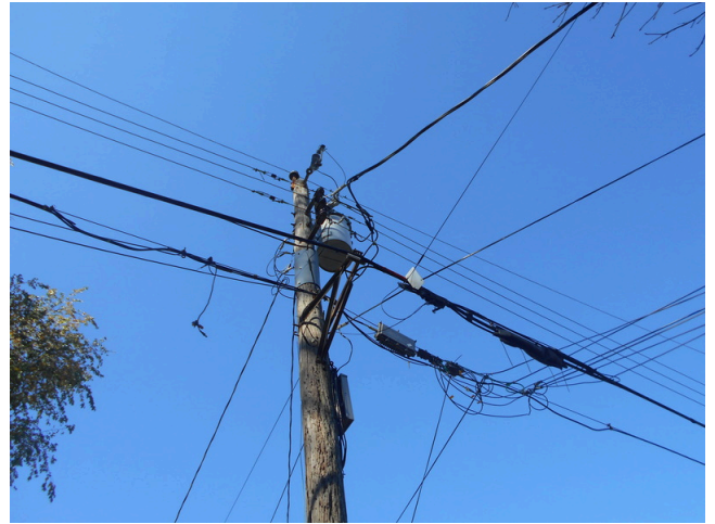
46. Pole mounted electrical transformer
