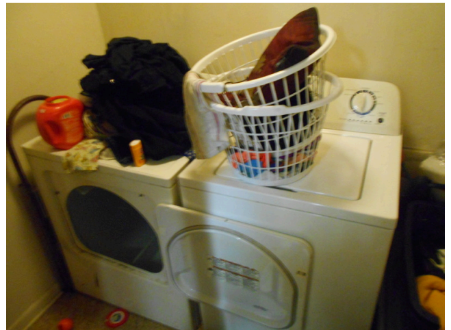
44. Unit F - 1bed/1bath - Mechanical closet
