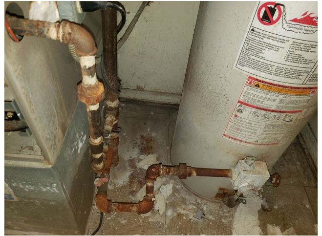
22. Update-Unit A - 1bed/1bath, vacant -Laundry Room- Furnace- Rusty Pipes
