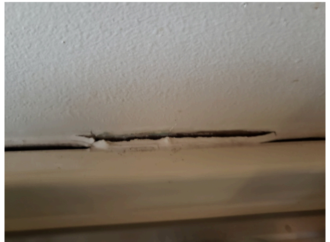
32. Update-Unit C - 1bed/1bath, occupied - 2nd Floor- Kitchen- Drywall cracked
