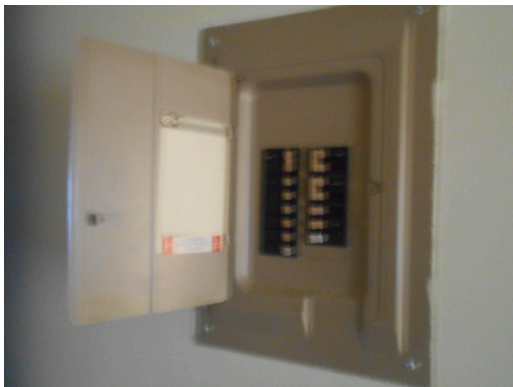
Unit E - 1bed/1bath, vacant - Electrical panel
