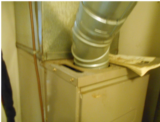
Unit F - 1bed/1bath - Mechanical closet furnace vent
