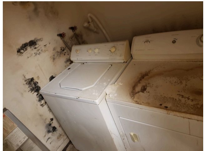
48. Update- Unit A - 1bed/1bath, vacant -Laundry Room- Mold
