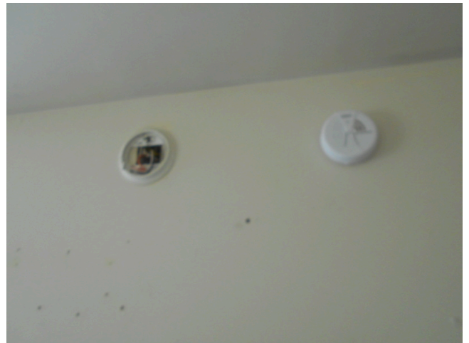
8. Unit D - 1bed/1bath, vacant - Smoke detector and CO detector
