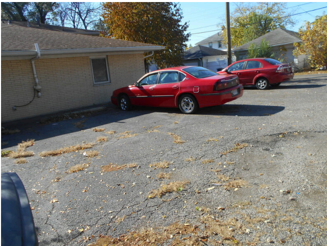
35. Asphalt parking lot, cracked and faded lines
