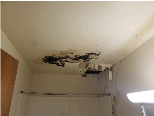
3. Update- Unit A - 1bed/1bath, vacant - Bathroom- Ceiling mold
