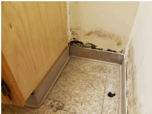
Update- Unit A - 1bed/1bath, vacant - Bathroom- Wall mold
