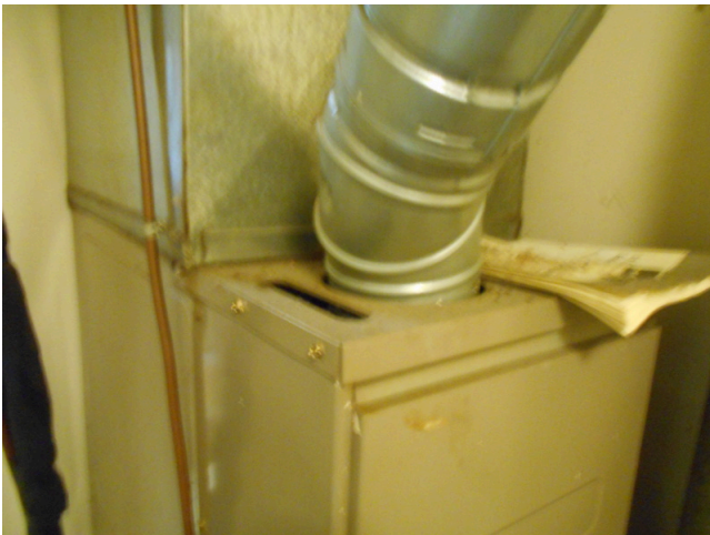
47. Unit F - 1bed/1bath - Mechanical closet furnace vent
