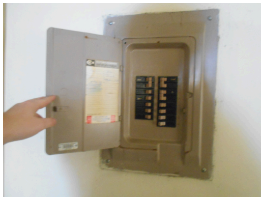
Unit D - 1bed/1bath, vacant - Electrical panel, older model
