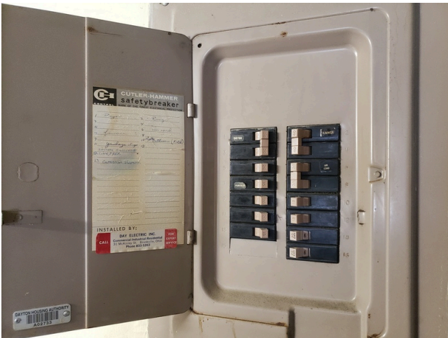
75. Update- Unit D - 1bed/1bath, vacant - Electrical Panel
