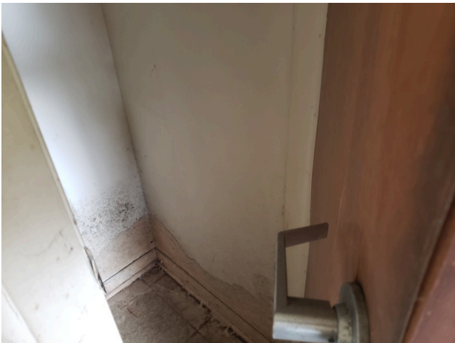
43. Update- Unit A - 1bed/1bath, vacant - Living Room- Closet- Mold
