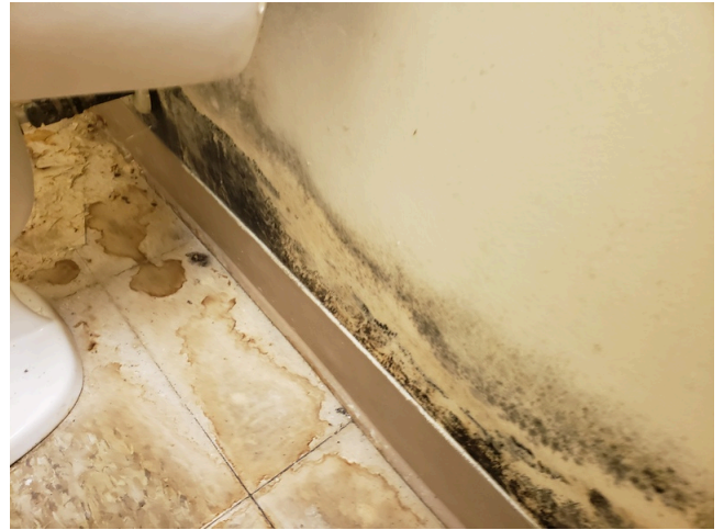
10. Update- Unit A - 1bed/1bath, vacant - Bathroom- Wall mold
