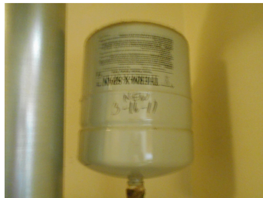
Unit F - 1bed/1bath - Mechanical closet water heater expansion tank
