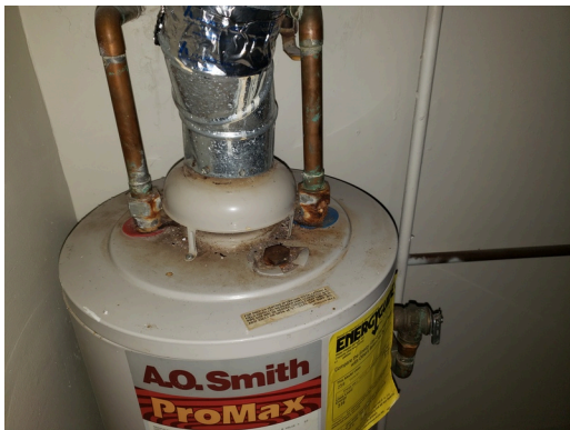
Typical water heater
