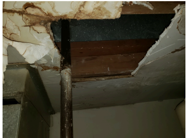
24. Update-Unit A - 1bed/1bath, vacant -Laundry Room- Water damage ceiling
