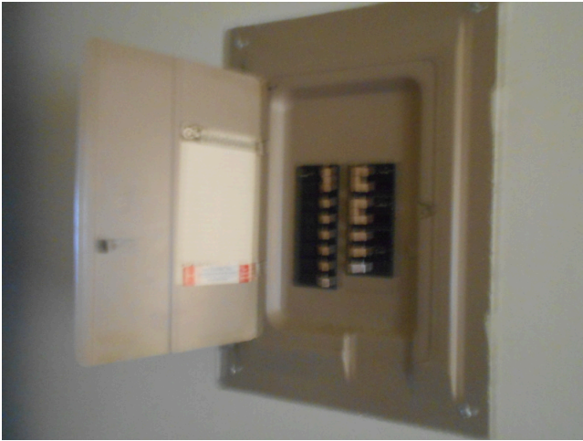
33. Unit E - 1bed/1bath, vacant - Electrical panel
