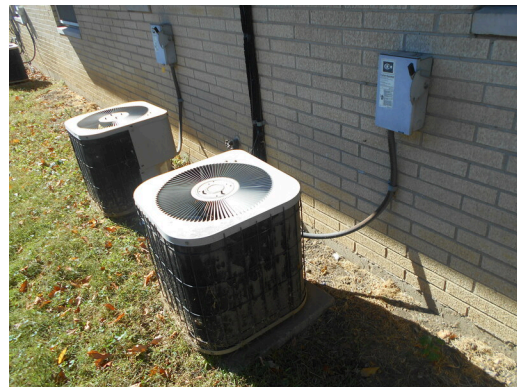
A/C condenser units
