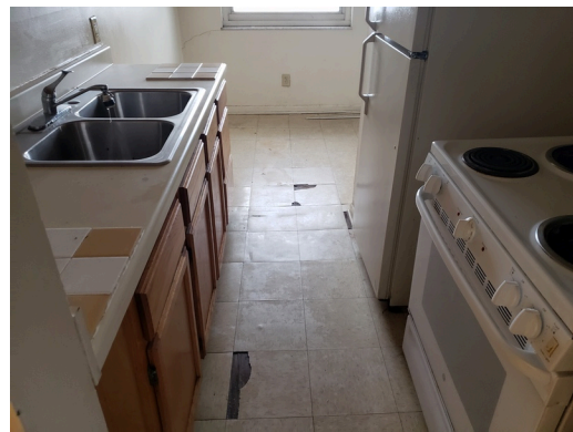
Update- Unit B - 1bed/1bath, vacant - 2nd Floor- Kitchen- Damaged Flooring
