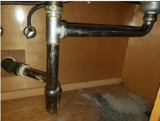
55. Update- Unit B - 1bed/1bath, vacant - 2nd Floor- Kitchen Pipes
