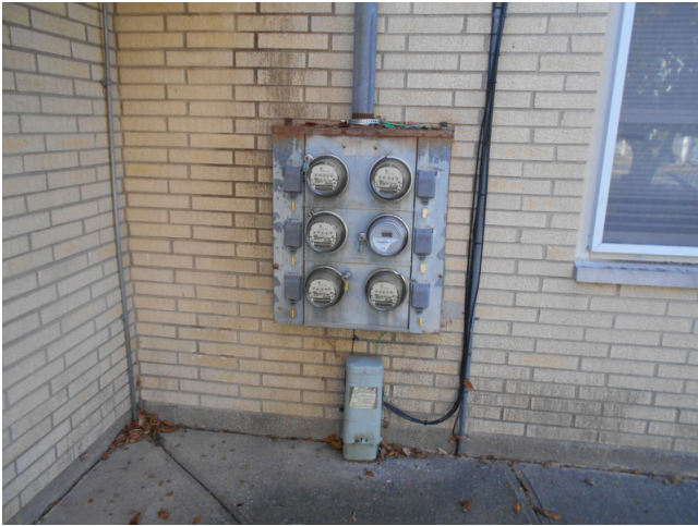
13. Electrical meters, dated infrastructure
