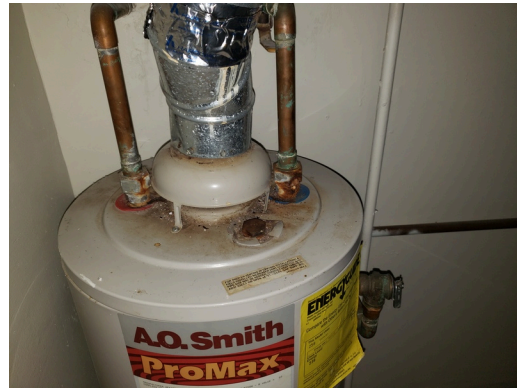
Typical water heater
