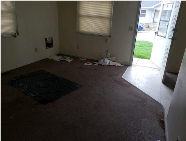
81. Update- Unit D - 1bed/1bath, vacant - Living Room- damaged wall
