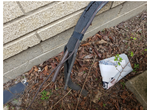
A/C units, damaged A/C condenser line set
