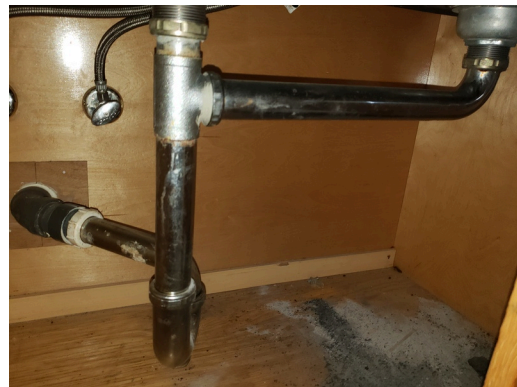
Update- Unit B - 1bed/1bath, vacant - 2nd Floor- Kitchen Pipes
