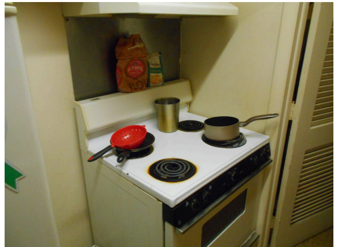
40. Unit F - 1bed/1bath - Kitchen range, no wall shield
