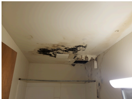
Update- Unit A - 1bed/1bath, vacant - Bathroom- Ceiling mold
