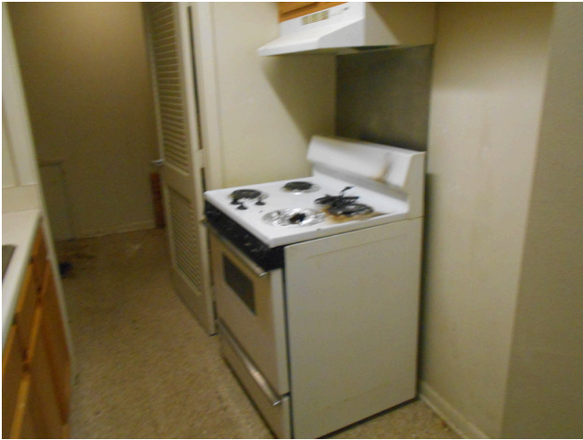
25. Unit E - 1bed/1bath, vacant - Kitchen stove and overhead, no wall shield
