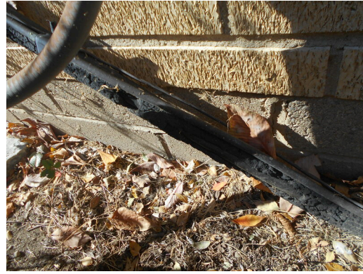
A/C units, damaged A/C insulation line
