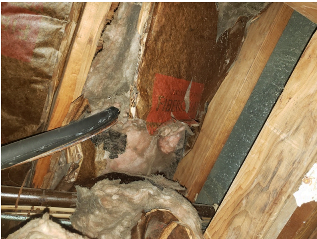
23. Update-Unit A - 1bed/1bath, vacant -Laundry Room- Water damage ceiling
