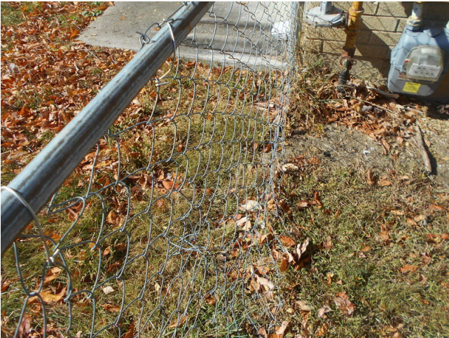
32. Damaged chain link fencing
