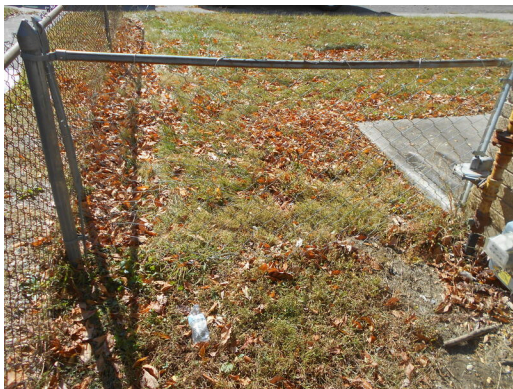
Damaged chain link fencing
