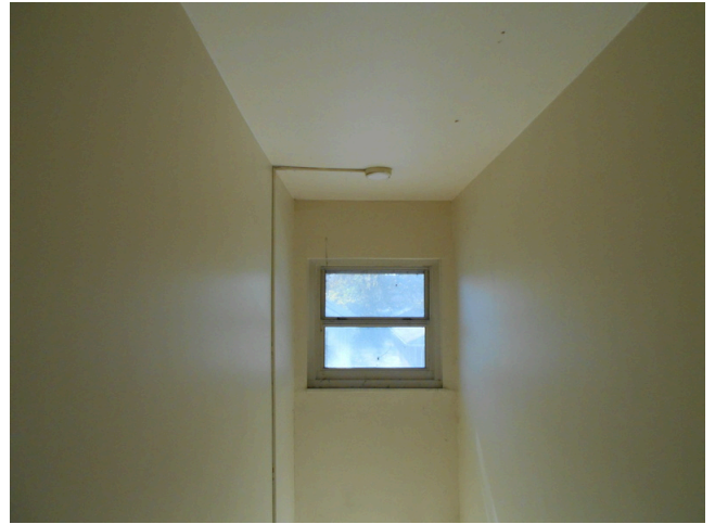
10. Stairwell smoke detector, hard wired
