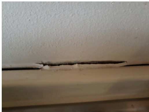
Update-Unit C - 1bed/1bath, occupied - 2nd Floor- Kitchen- Drywall cracked
