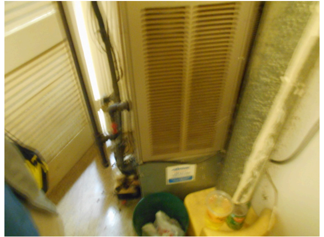
46. Unit F - 1bed/1bath - Mechanical closet furnace
