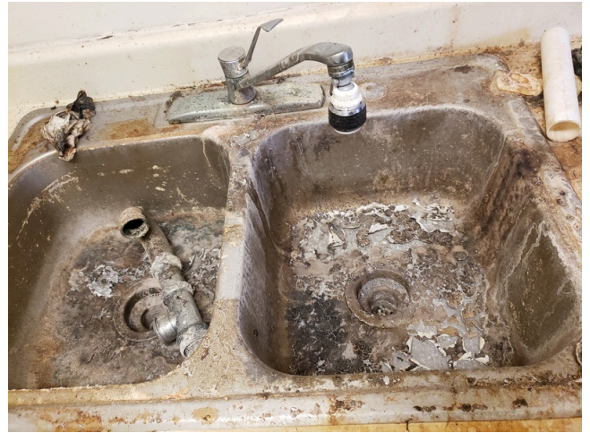
42. Update- Unit A - 1bed/1bath, vacant - Kitchen- Replace older sink
