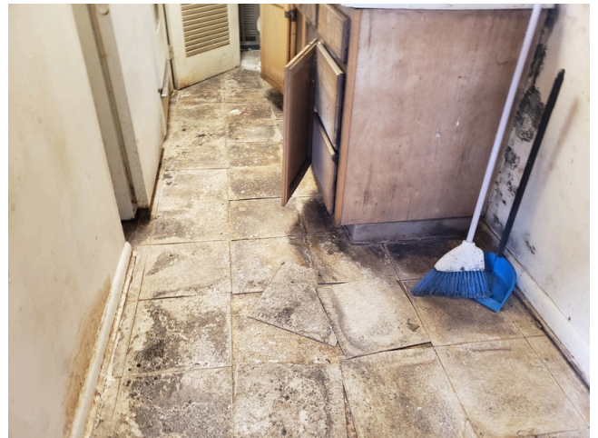
12. Update- Unit A - 1bed/1bath, vacant - Dining Room- Replace damaged VCT
