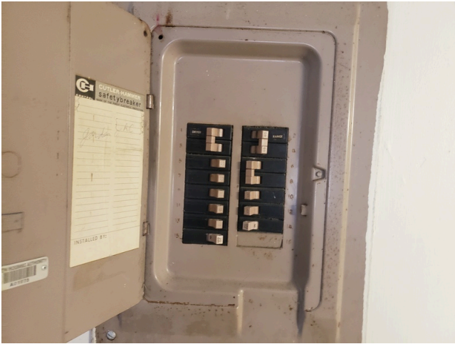
13. Update- Unit A - 1bed/1bath, vacant - electrical panel
