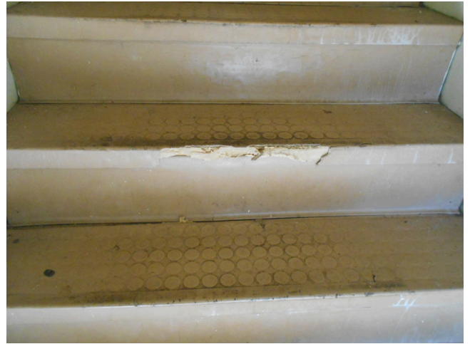
6. Stairwell, damaged stairs
