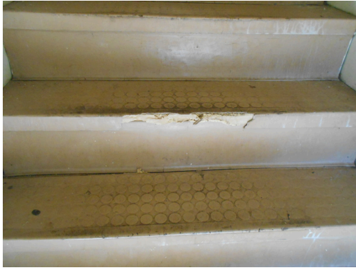
Stairwell, damaged stairs
