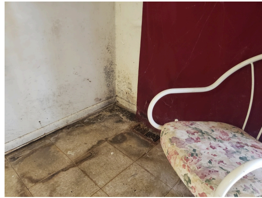
Update- Unit A - 1bed/1bath, vacant - Dining Room- Replace damaged VCT
