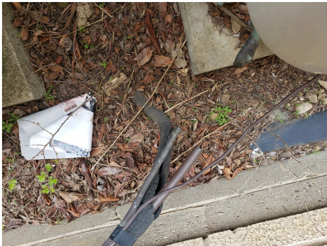
55. A/C units, damaged A/C insulation line
