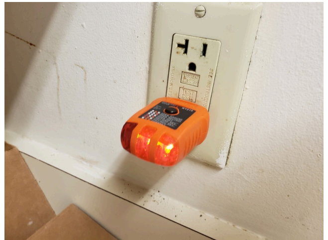
72. Update- Unit D - 1bed/1bath, vacant - Bathroom- GFCI outlet
