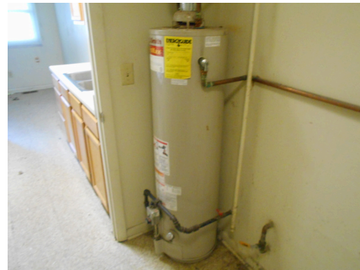
Unit E - 1bed/1bath, vacant - Mechanical closet water heater
