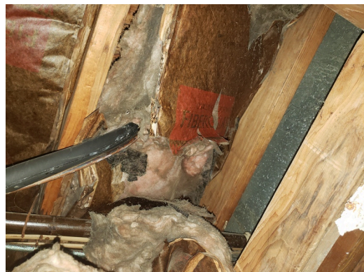
Unit A - 1bed/1bath, Laundry Room- Water damage ceiling
