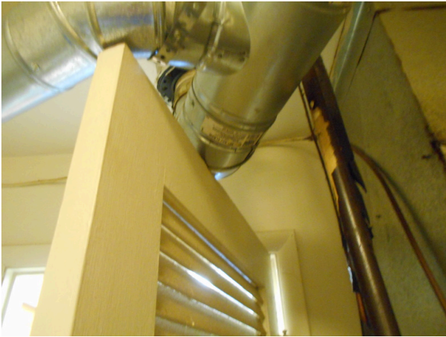
49. Unit F - 1bed/1bath - Mechanical closet furnace vent, hits with door swing
