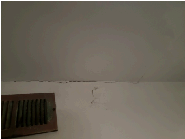
31. Update-Unit C - 1bed/1bath, occupied - 2nd Floor- Kitchen- Drywall cracked
