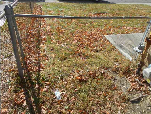
31. Damaged chain link fencing
