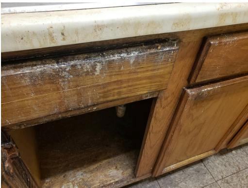
Update- Unit D - 1bed/1bath, vacant - Kitchen- Cabinet Older
