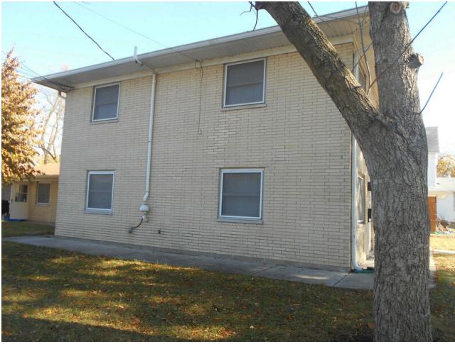
41. Building side facade, deteriorated mortar
