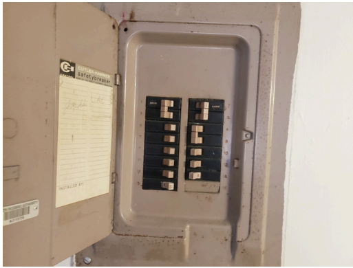
Update- Unit A - 1bed/1bath, vacant - electrical panel
