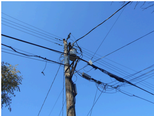
Pole mounted electrical transformer
