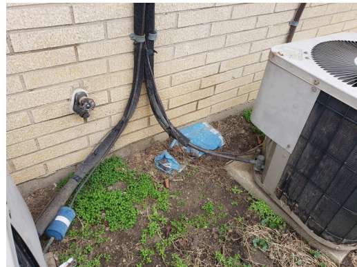
Condenser line sets
