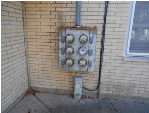
Electrical meters, dated infrastructure
