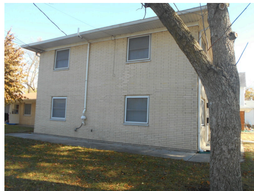
Building side facade, deteriorated mortar
