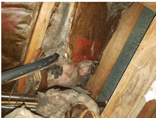
Update-Unit A - 1bed/1bath, vacant -Laundry Room- Hot water heater piping
