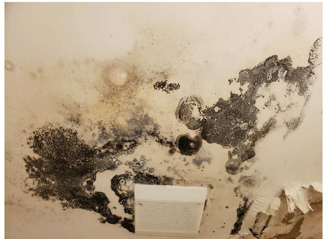
4. Update- Unit A - 1bed/1bath, vacant - Bathroom- Ceiling mold
