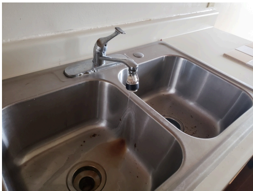
Update- Unit B - 1bed/1bath, vacant - 2nd Floor- Kitchen- Poor Water Flow
