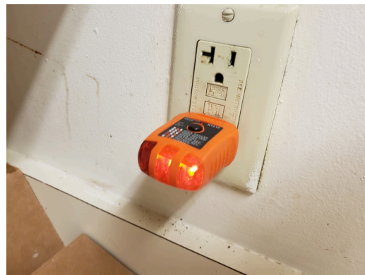
Update- Unit D - 1bed/1bath, vacant - Bathroom- GFCI outlet
