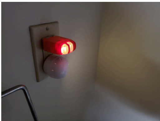
Update-Unit C - 1bed/1bath, occupied - 2nd Floor- Bathroom- GFCI outlet
