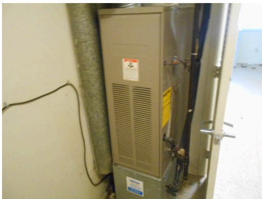
Unit E - 1bed/1bath, vacant - Mechanical closet furnace
