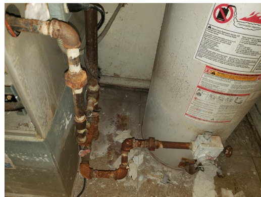
Update-Unit A - 1bed/1bath, vacant -Laundry Room- Furnace- Rusty Pipes
