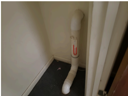
Update- Unit A - 1bed/1bath, vacant- Plumbing
