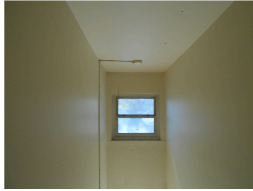
Stairwell smoke detector, hard wired
