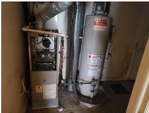
Update- Unit B - 1bed/1bath, vacant - 2nd Floor- Furnace and Water Heater
