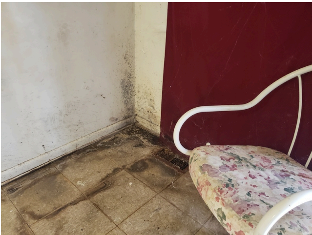
11. Update- Unit A - 1bed/1bath, vacant - Dining Room- Replace damaged VCT
