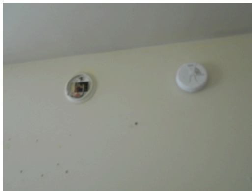
Unit D - 1bed/1bath, vacant - Smoke detector and CO detector
