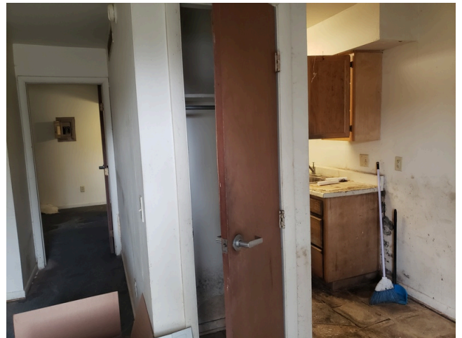
44. Update- Unit A - 1bed/1bath, vacant - Living Room- Closet- Mold
