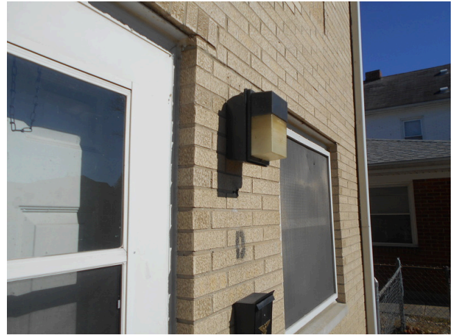
38. Building mounted exterior lighting
