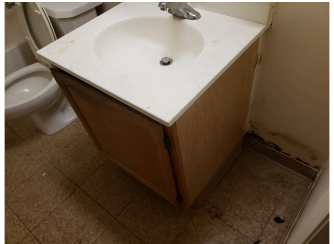
8. Update- Unit A - 1bed/1bath, vacant - Bathroom- Wall mold
