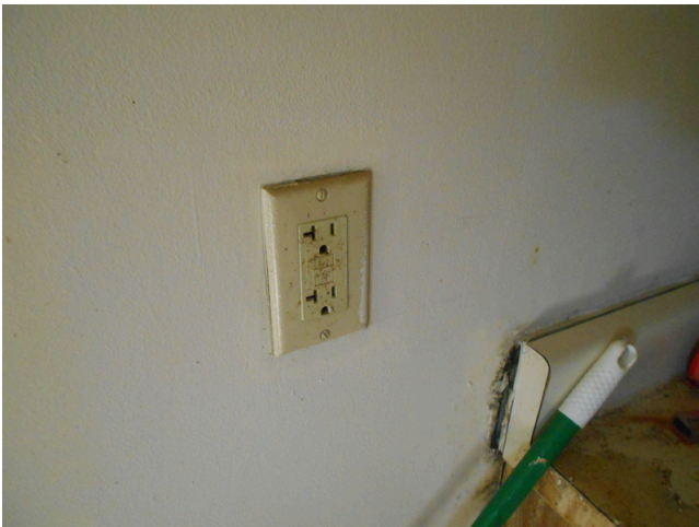
7. Unit D - 1bed/1bath, vacant - Kitchen GFCI
