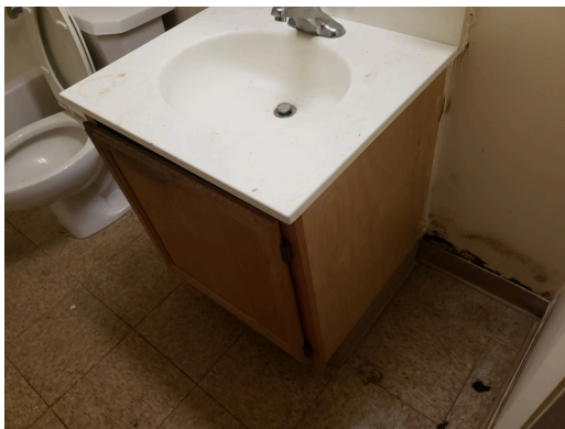
Update- Unit A - 1bed/1bath, vacant - Bathroom- Wall mold
