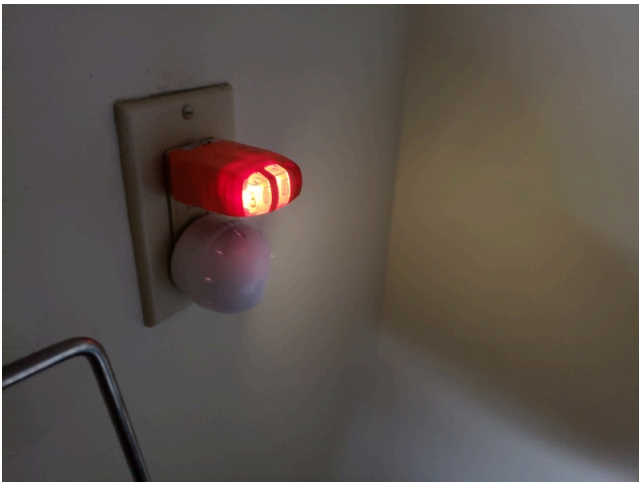
27. Update-Unit C - 1bed/1bath, occupied - 2nd Floor- Bathroom- GFCI outlet
