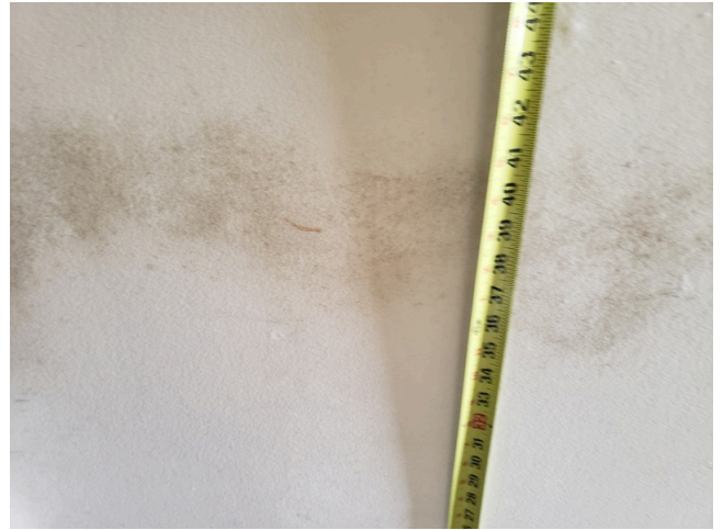
46. Update- Unit A - 1bed/1bath, vacant - Living Room- Mold/ water damage
