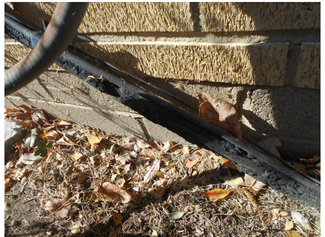
28. A/C units, damaged A/C insulation line
