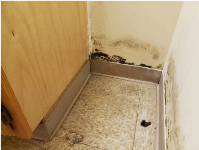
9. Update- Unit A - 1bed/1bath, vacant - Bathroom- Wall mold
