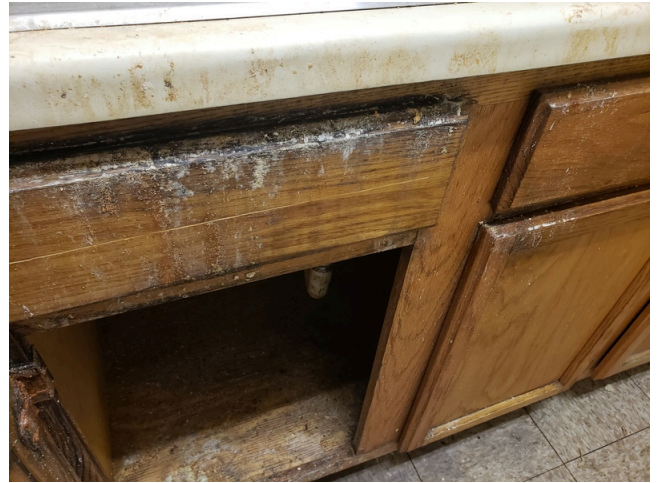
78. Update- Unit D - 1bed/1bath, vacant - Kitchen- Cabinet Older
