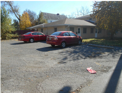
Asphalt parking lot, cracked and faded lines
