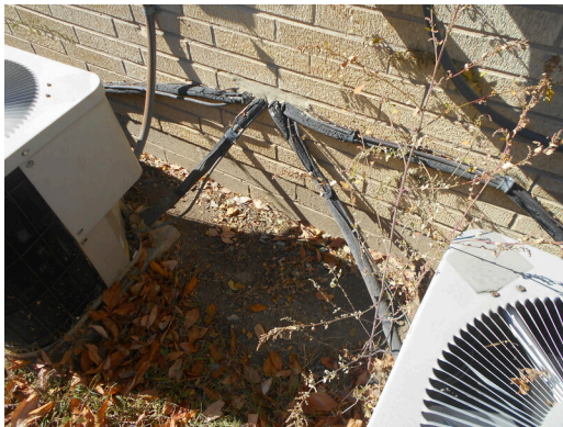
A/C units, damaged A/C insulation line
