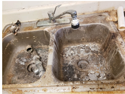
Update- Unit A - 1bed/1bath, vacant - Kitchen- Replace older sink
