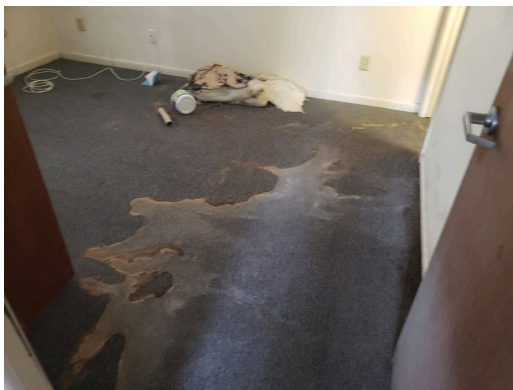
Update- Unit A - 1bed/1bath, vacant -Bedroom- Replace water damaged carpet
