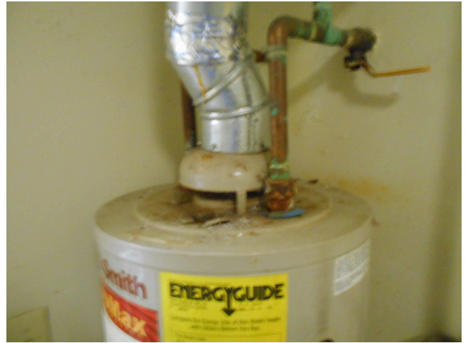
30. Unit E - 1bed/1bath, vacant - Mechanical closet water heater
