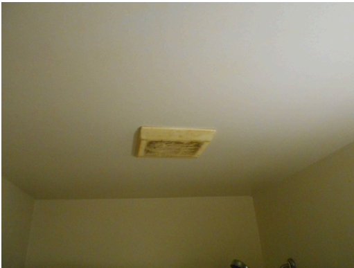
Unit F - 1bed/1bath - Bathroom ceiling
