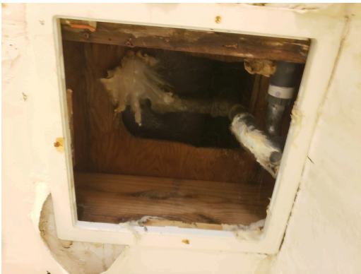
Unit A - 1bed/1bath, Bathroom- plumbing with observed damaged subfloor and joists
