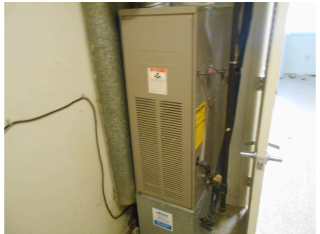
28. Unit E - 1bed/1bath, vacant - Mechanical closet furnace
