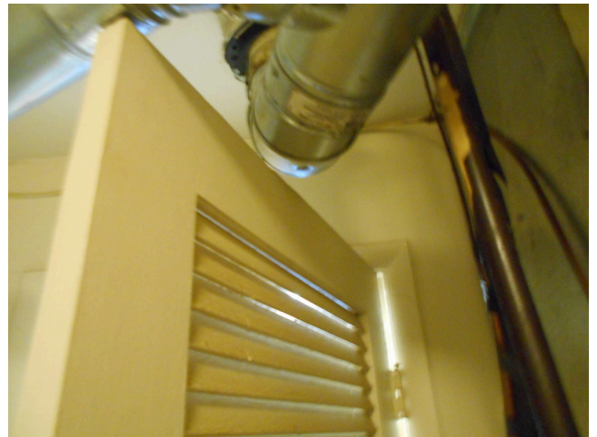
48. Unit F - 1bed/1bath - Mechanical closet furnace vent, hits with door swing
