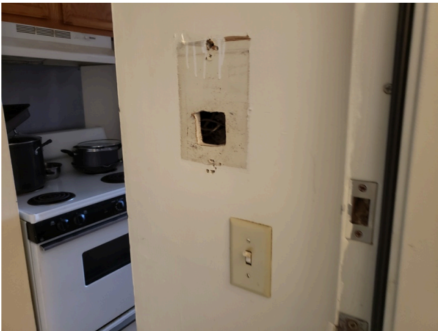
67. Update- Unit C - 1bed/1bath, occupied - 2nd Floor- Whole in drywall
