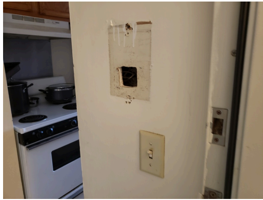
Update- Unit C - 1bed/1bath, occupied - 2nd Floor- Whole in drywall
