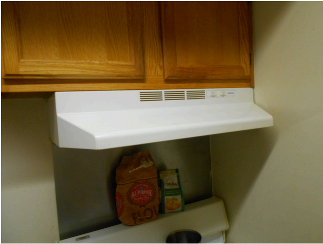
41. Unit F - 1bed/1bath - Kitchen range overhead
