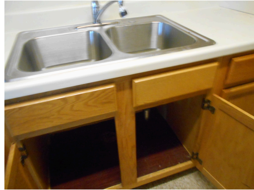
Unit E - 1bed/1bath, vacant - Kitchen sink
