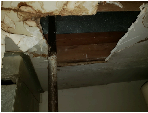
Unit A - 1bed/1bath, Laundry Room- Water damage ceiling
