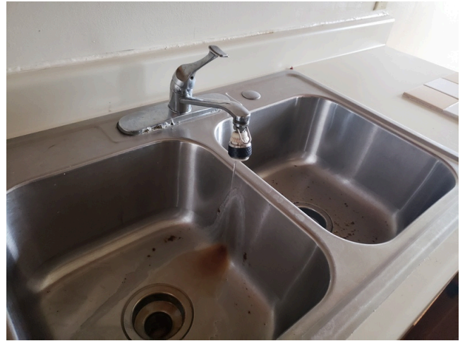
58. Update- Unit B - 1bed/1bath, vacant - 2nd Floor- Kitchen- Poor Water Flow
