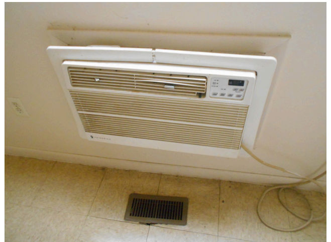
24. Unit 265 - 1bed/1bath, vacant - Thru-wall A/C unit
