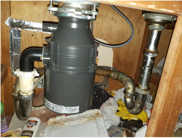
73. Unit 267-C - 1bed/1bath, occupied-(update)- Kitchen- Garbage disposal and pipes
