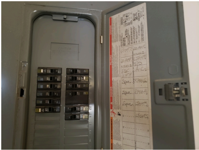
17. Unit 265- D - 1bed/1bath,vacant-(update)- Electrical panel
