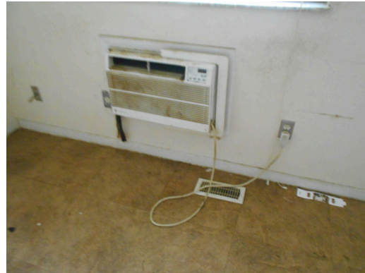
Unit 261 - 1bed/1bath, vacant - Thru-wall A/ C unit
