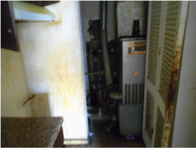
5. Unit 261 - 1bed/1bath, vacant - Mechanical closet
