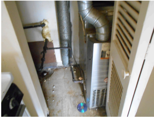
Unit 265 - 1bed/1bath, vacant - Mechanical closet
