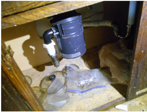
Unit 261 - 1bed/1bath, vacant - Kitchen sink, garbage disposal
