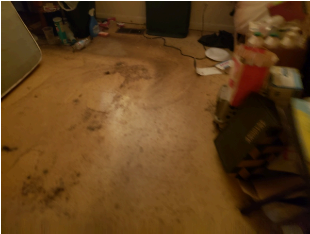
55. Unit 267-B - 1bed/1bath, occupied-(update)- Bedroom- Damaged VCT
