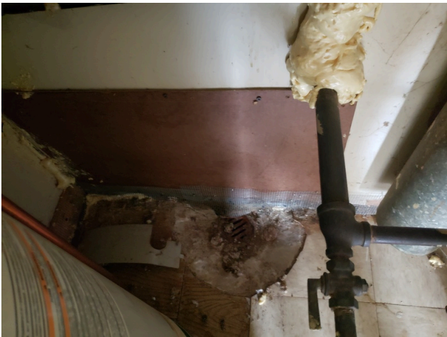
23. Unit 265- D - 1bed/1bath,vacant-(update)- Mechanical room- damaged drywall
