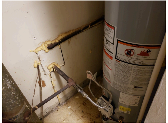
42. Unit 267-A - 1bed/1bath, occupied-(update)- Mechanical room- damaged drywall
