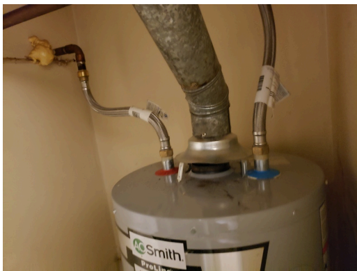
Unit 267-A - 1bed/1bath, occupied-(update)- 30-Gal gas water heater- MFG 2022
