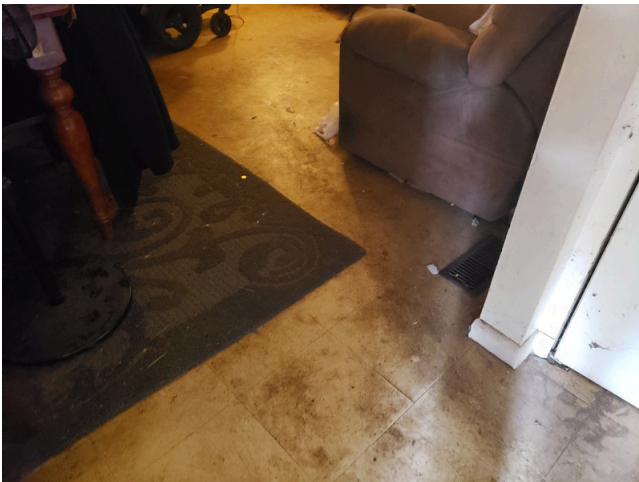
59. Unit 267-B - 1bed/1bath, occupied-(update)- Living room- Damaged VCT
