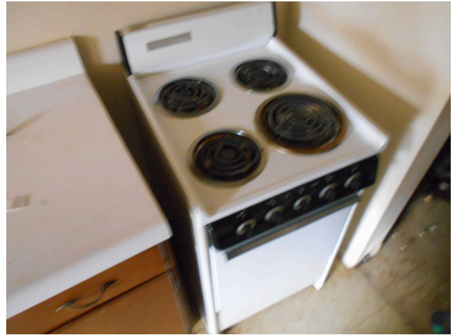
22. Unit 265 - 1bed/1bath, vacant - Kitchen stove, no wall shield
