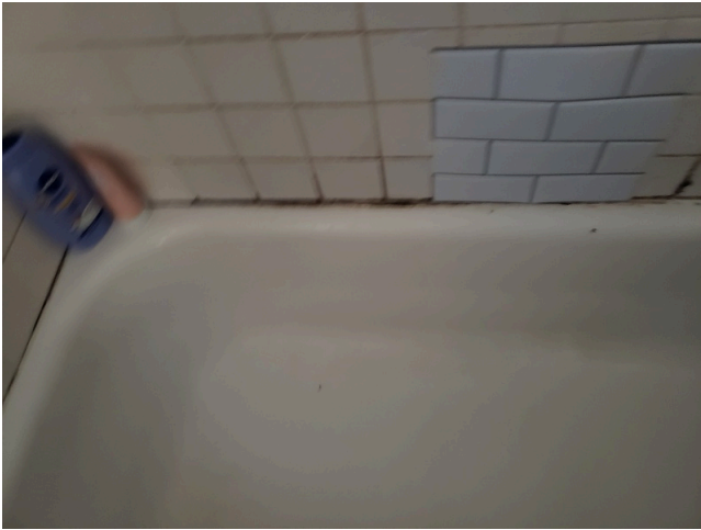
65. Unit 267-C - 1bed/1bath, occupied-(update)- Bathroom- Damaged tile
