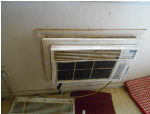
Unit 267-A - 1bed/1bath, vacant - Thru-wall A/C unit
