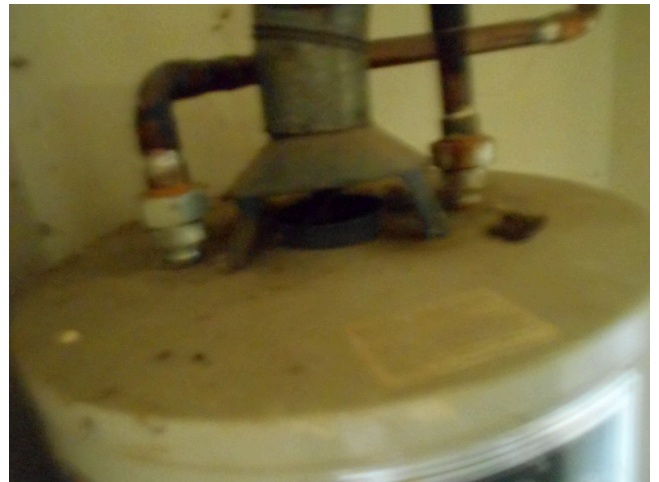
20. Unit 265 - 1bed/1bath, vacant - Water heater
