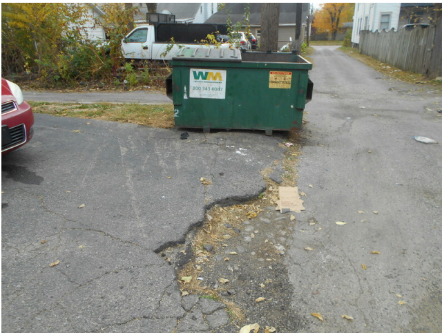
31. Asphalt parking area, damaged
