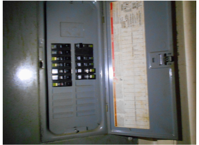
46. Unit 267-A - 1bed/1bath, vacant - Electrical panel
