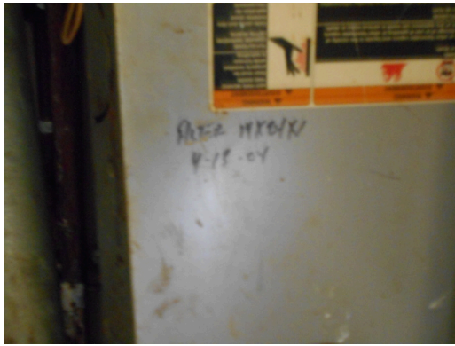
Unit 261 - 1bed/1bath, vacant - Mechanical closet
