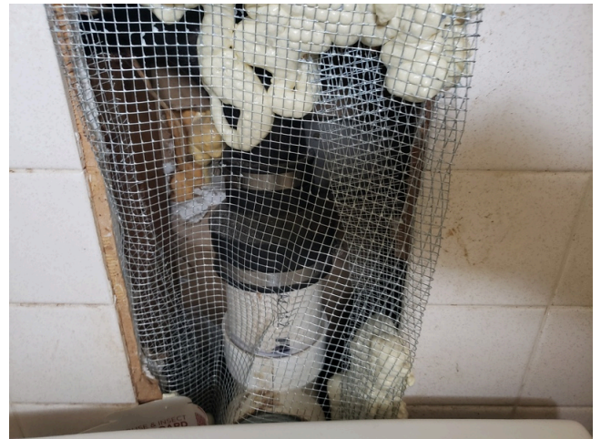
64. Unit 267-C - 1bed/1bath, occupied-(update)- Bathroom- Damaged tile
