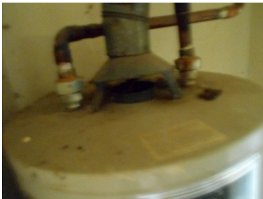
Unit 265 - 1bed/1bath, vacant - Water heater
