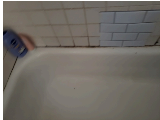
Unit 267-C - 1bed/1bath, occupied-(update)- Bathroom- Damaged tile
