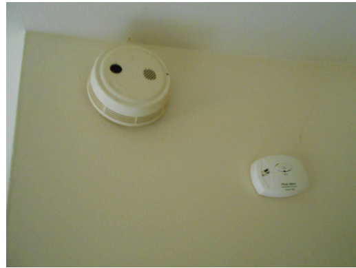
Unit 265 - 1bed/1bath, vacant - Smoke detector and CO detector
