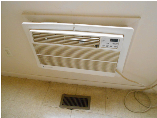
Unit 265 - 1bed/1bath, vacant - Thru-wall A/C unit
