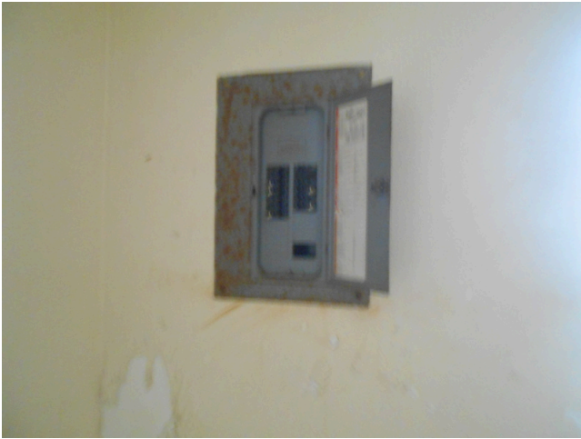
9. Unit 261 - 1bed/1bath, vacant - electrical panel
