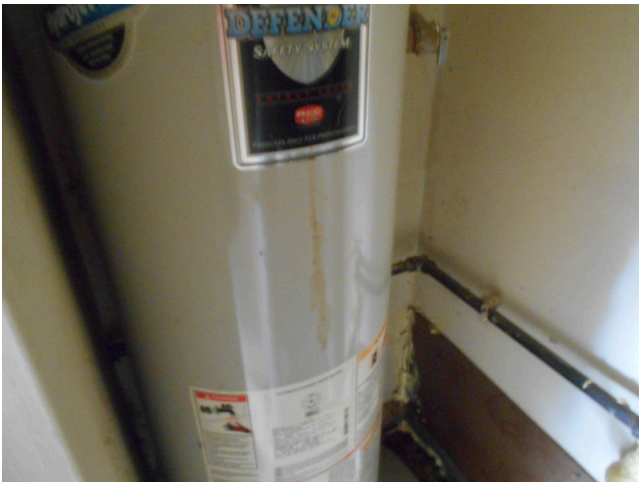
19. Unit 265 - 1bed/1bath, vacant - Water heater
