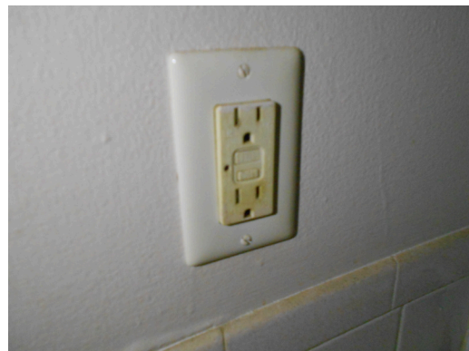
Unit 265 - 1bed/1bath, vacant - Bathroom GFCI
