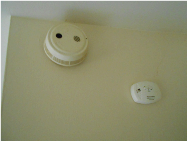
25. Unit 265 - 1bed/1bath, vacant - Smoke detector and CO detector
