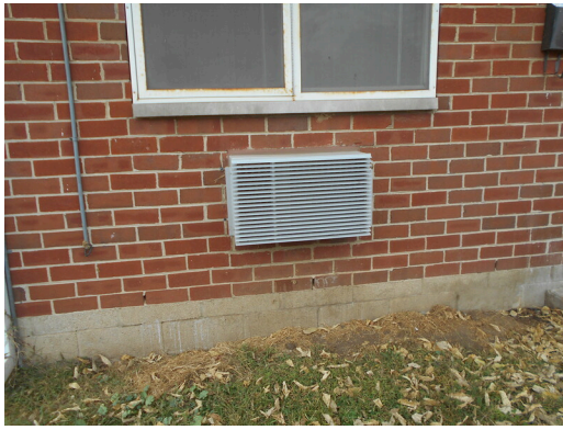
Thru-wall A/C units
