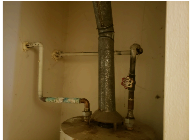
68. Unit 267-C - 1bed/1bath, occupied-(update)- Corroded pipes
