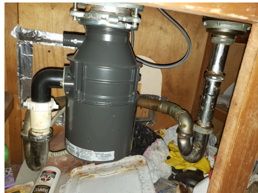
Unit 267-C - 1bed/1bath, occupied-(update)-Kitchen- Garbage disposal and pipes
