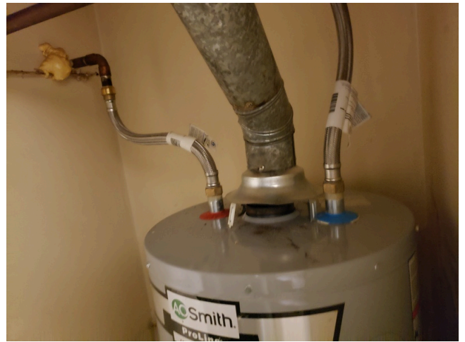
30. Unit 267-A - 1bed/1bath, occupied-(update)- 30-Gal gas water heater- MFG 2022
