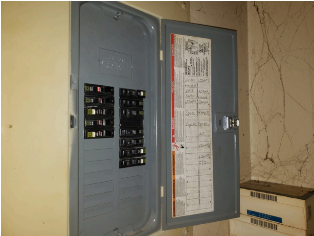
56. Unit 267-B - 1bed/1bath, occupied-(update)- Electrical panel
