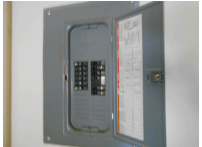
28. Unit 265 - 1bed/1bath, vacant - Electrical panel
