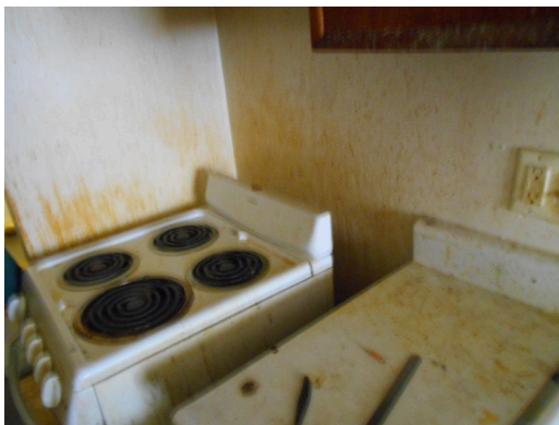
Unit 267-A - 1bed/1bath, vacant - Kitchen stove, no wall shield
