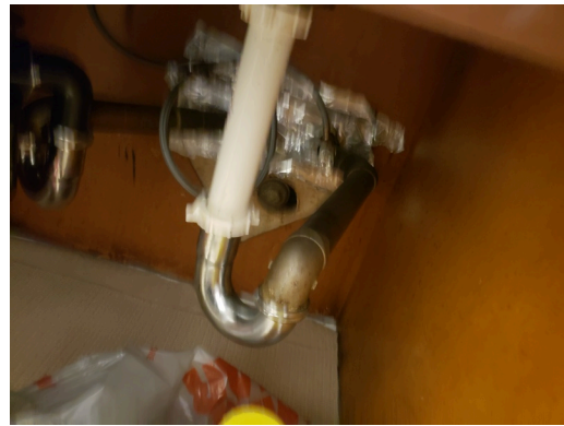
Unit 267-A - 1bed/1bath, occupied-(update)- Kitchen- plumbing
