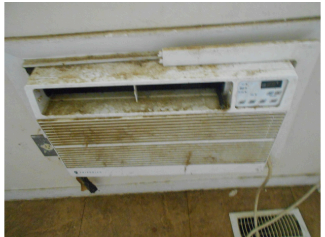
12. Unit 261 - 1bed/1bath, vacant - Thru-wall A/C unit
