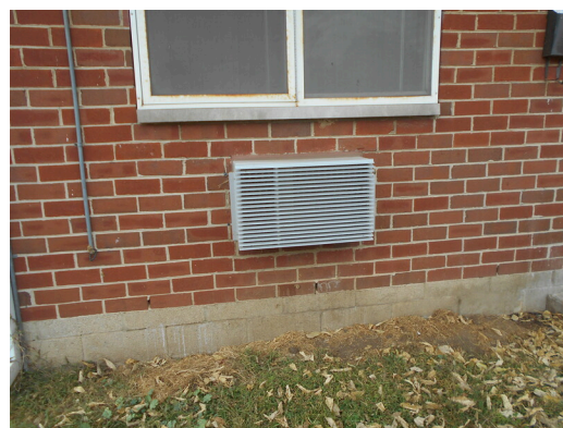
Thru-wall A/C units
