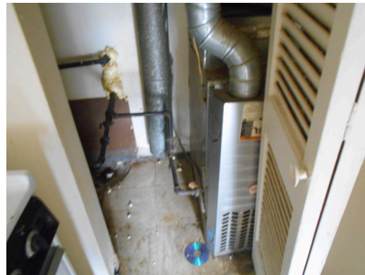
Unit 265 - 1bed/1bath, vacant - Mechanical closet
