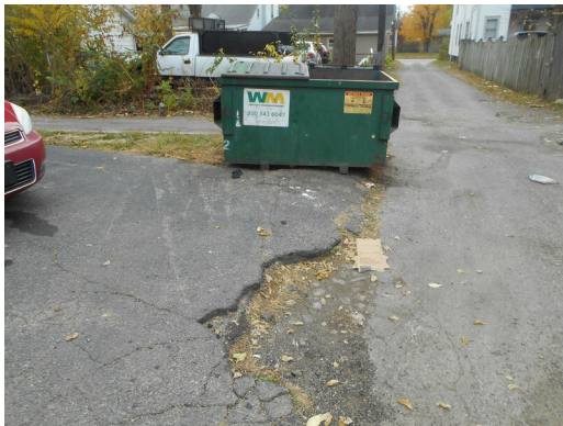
Asphalt parking area, damaged
