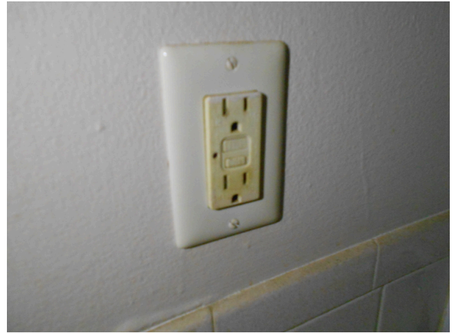
30. Unit 265 - 1bed/1bath, vacant - Bathroom GFCI
