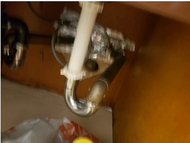
39. Unit 267-A - 1bed/1bath, occupied-(update)- Kitchen- plumbing
