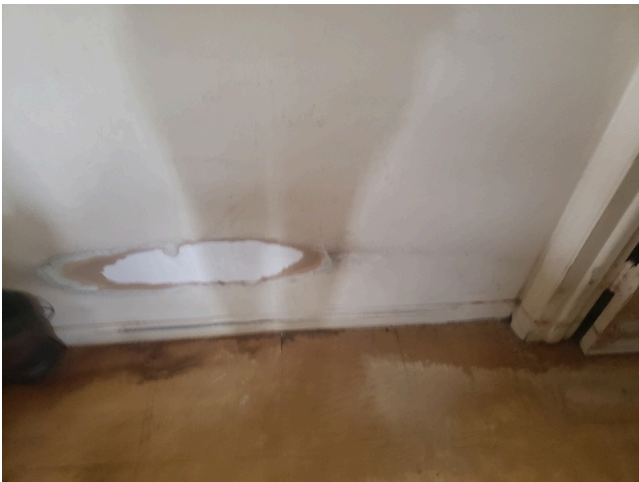
7. Unit 263-E - 1bed/1bath, occupied-(update)- Bedroom- Damaged drywall
