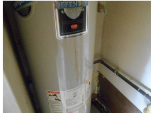
Unit 265 - 1bed/1bath, vacant - Water heater
