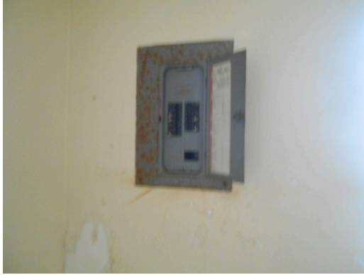
Unit 261 - 1bed/1bath, vacant - electrical panel
