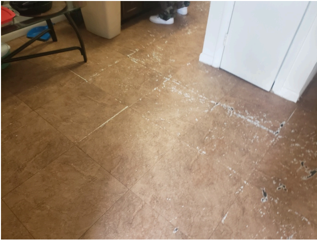
1. Unit 261-F - 1bed/1bath, occupied-(update)- Damaged VCT
