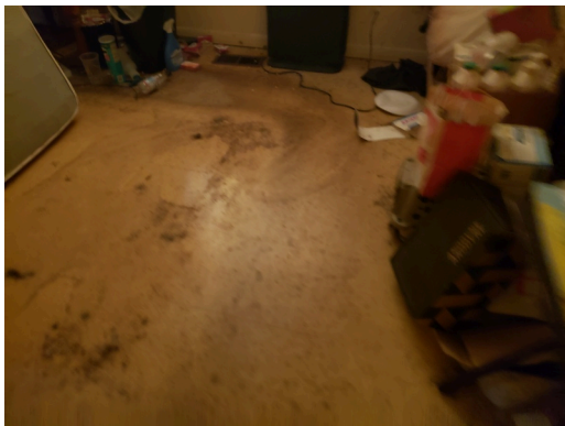
Unit 267-B - 1bed/1bath, occupied-(update)- Bedroom- Damaged VCT
