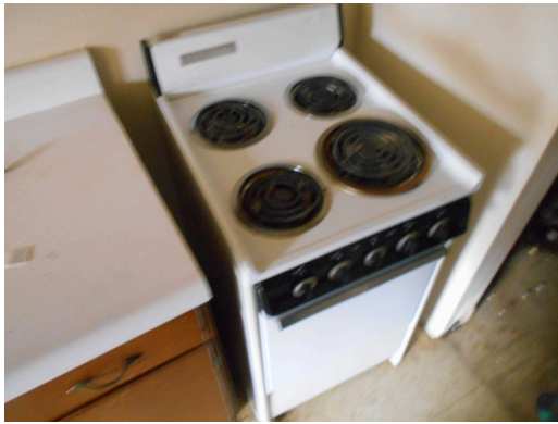
Unit 265 - 1bed/1bath, vacant - Kitchen stove, no wall shield
