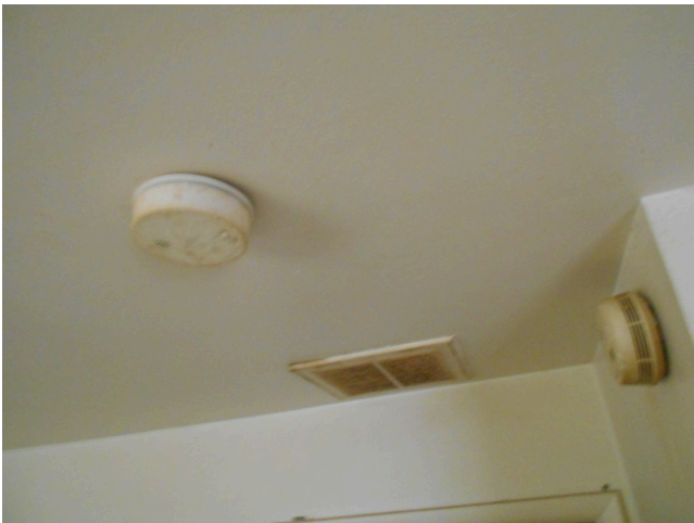
51. Unit 267-A - 1bed/1bath, vacant - Living area smoke detectors
