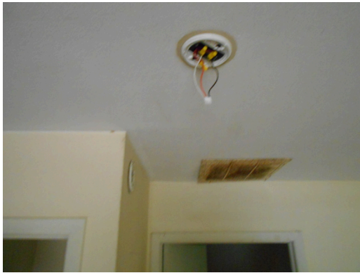
Unit 261 - 1bed/1bath, vacant - Smoke detector
