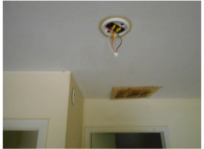
14. Unit 261 - 1bed/1bath, vacant - Smoke detector
