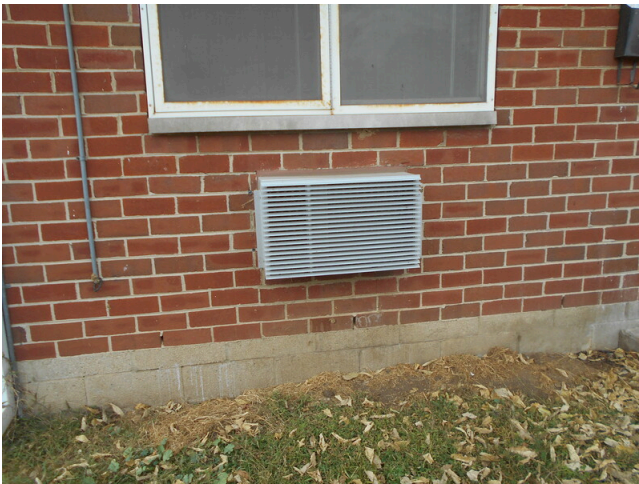
15. Thru-wall A/C units
