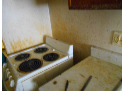
Unit 267-A - 1bed/1bath, vacant - Kitchen stove, no wall shield
