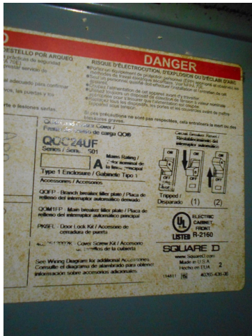
47. Unit 267-A - 1bed/1bath, vacant - Electrical panel
