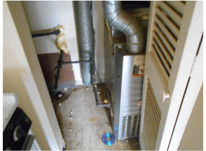
18. Unit 265 - 1bed/1bath, vacant - Mechanical closet
