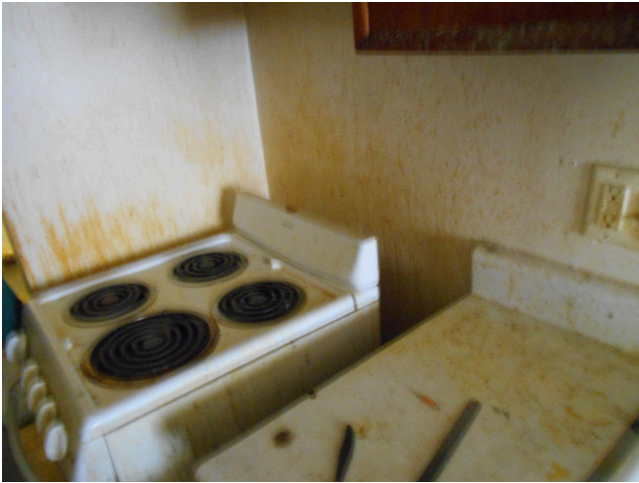
49. Unit 267-A - 1bed/1bath, vacant - Kitchen stove, no wall shield
