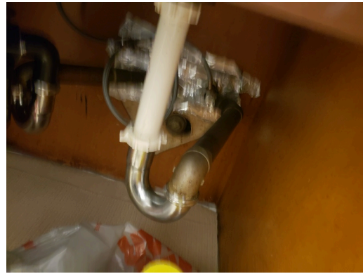
Unit 267-A - 1bed/1bath, occupied-(update)- Kitchen- plumbing
