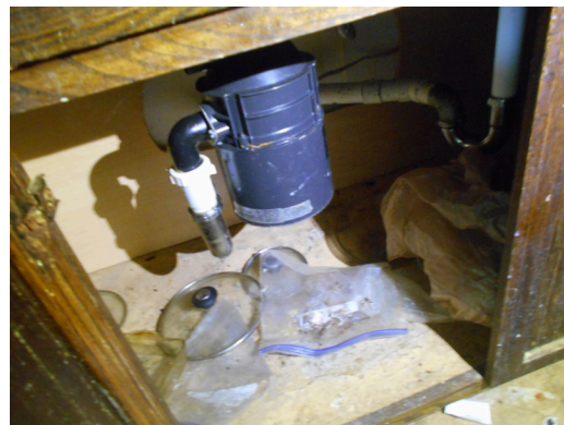
Unit 261 - 1bed/1bath, vacant - Kitchen sink, garbage disposal
