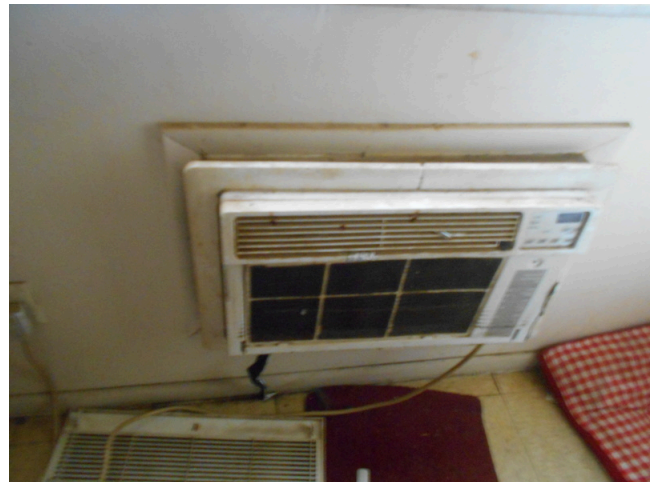
52. Unit 267-A - 1bed/1bath, vacant - Thru-wall A/C unit
