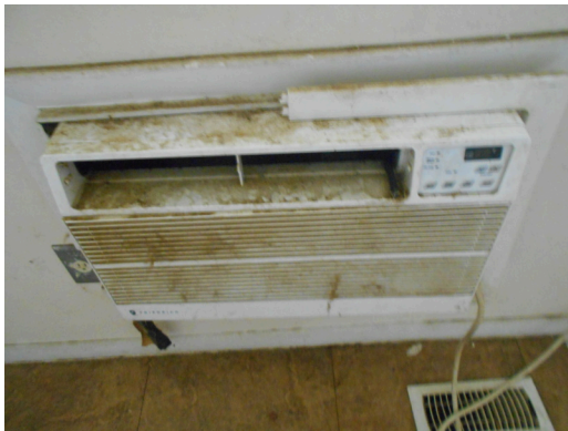
Unit 261 - 1bed/1bath, vacant - Thru-wall A/C unit
