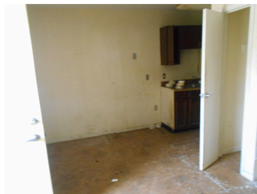
Unit 261 - 1bed/1bath, vacant - Living area
