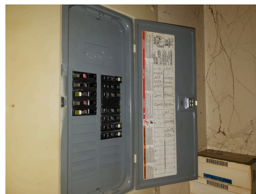
Unit 267-B - 1bed/1bath, occupied-(update)- Electrical panel
