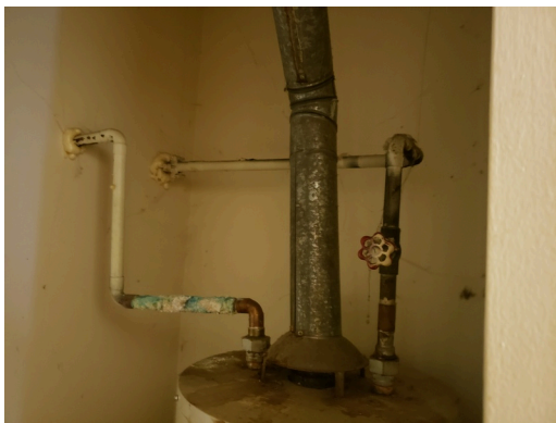
Unit 267-C - 1bed/1bath, occupied-(update)- Corroded pipes
