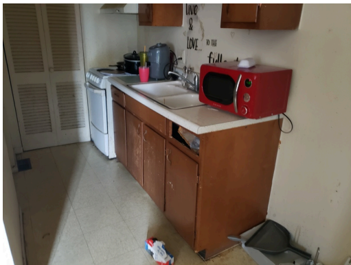
Unit 267-C - 1bed/1bath, occupied-(update)- Kitchen- Damaged cabinet
