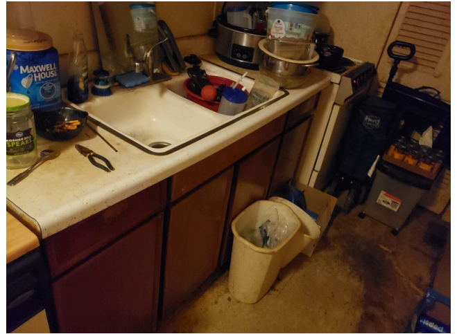
58. Unit 267-B - 1bed/1bath, occupied-(update)- Kitchen- Damaged VCT
