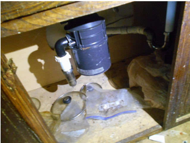
7. Unit 261 - 1bed/1bath, vacant - Kitchen sink, garbage disposal
