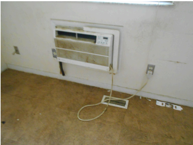
11. Unit 261 - 1bed/1bath, vacant - Thru-wall A/C unit
