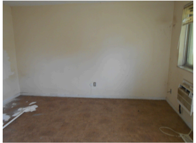
2. Unit 261 - 1bed/1bath, vacant - Living area
