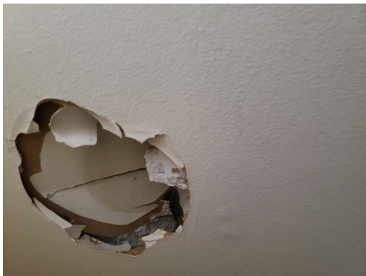
Unit 267-C - 1bed/1bath, occupied-(update)- Bedroom- Damaged drywall
