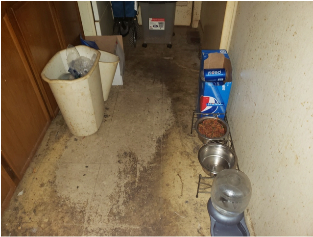
61. Unit 267-B - 1bed/1bath, occupied-(update)- Damaged VCT
