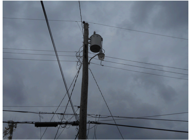
26. Pole mounted transformer
