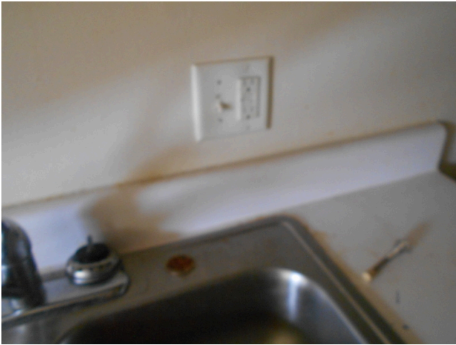
21. Unit 265 - 1bed/1bath, vacant - Kitchen GFCI
