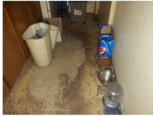
Unit 267-B - 1bed/1bath, occupied-(update)- Damaged VCT
