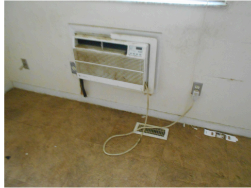
Unit 261 - 1bed/1bath, vacant - Thru-wall A/C unit
