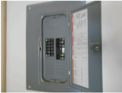
Unit 265 - 1bed/1bath, vacant - Electrical panel
