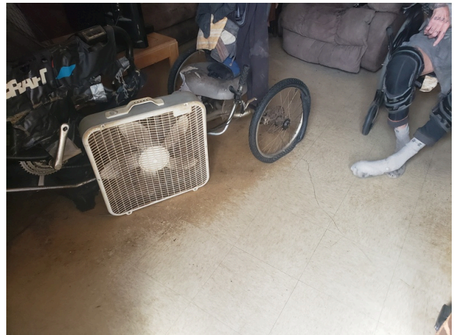
12. Unit 263-E - 1bed/1bath, occupied-(update)- Living room- damaged VCT
