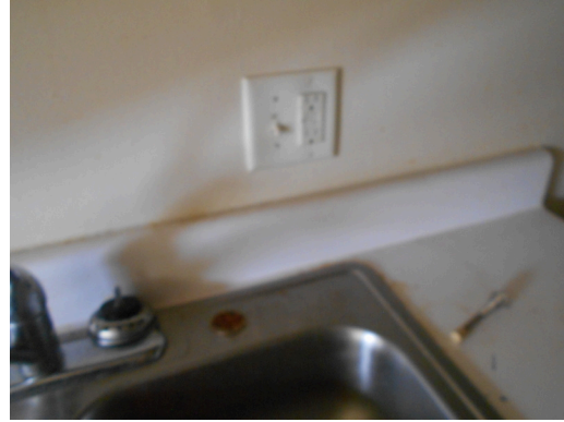
Unit 265 - 1bed/1bath, vacant - Kitchen GFCI
