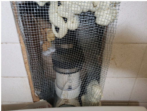
Unit 267-C - 1bed/1bath, occupied-(update)- Bathroom- Damaged tile
