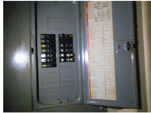
Unit 267-A - 1bed/1bath, vacant - Electrical panel
