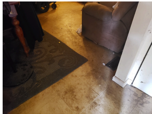
Unit 267-B - 1bed/1bath, occupied-(update)- Living room- Damaged VCT
