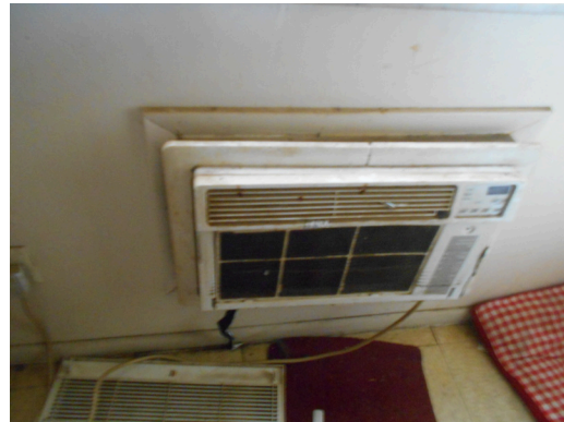
Unit 267-A - 1bed/1bath, vacant - Thru-wall A/C unit
