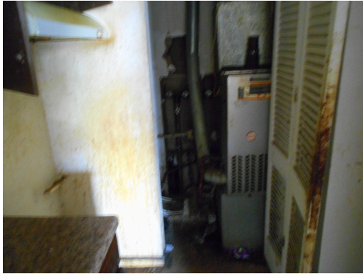
Unit 261 - 1bed/1bath, vacant - Mechanical closet
