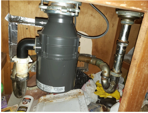
Unit 267-C - 1bed/1bath, occupied-(update)-Kitchen- Garbage disposal and pipes
