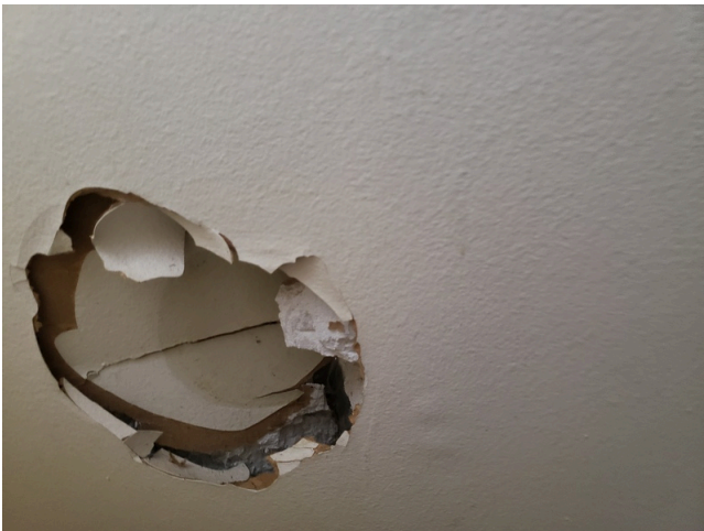
67. Unit 267-C - 1bed/1bath, occupied-(update)- Bedroom- Damaged drywall
