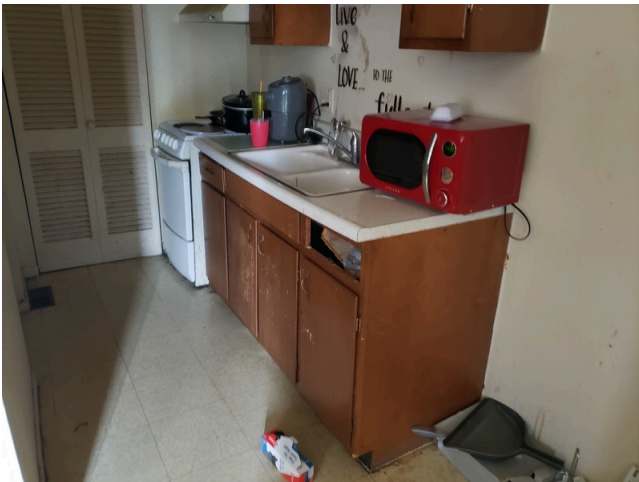
71. Unit 267-C - 1bed/1bath, occupied-(update)- Kitchen- Damaged cabinet
