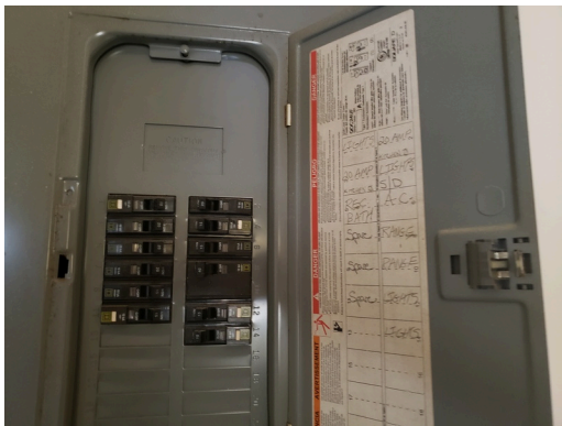
Unit 265- D - 1bed/1bath,vacant-(update)- Electrical panel
