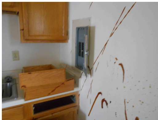
Unit A, 2 bedroom/1 bathroom, vacant - Kitchen electrical panel
