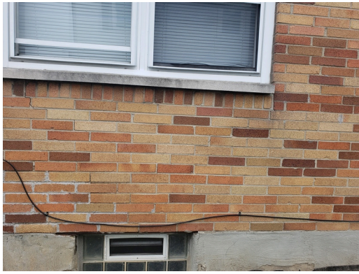
Update- North elevation minor cracking
