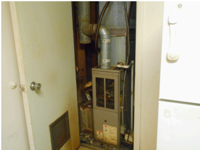
11. Unit E, 2 bedroom/1 bathroom - Furnace, older unit
