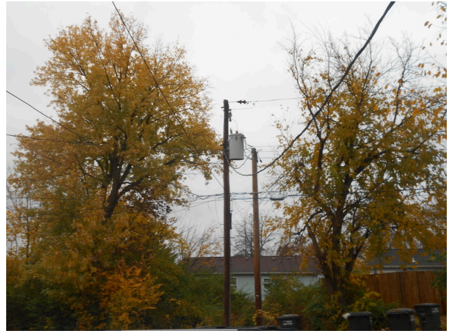
38. Pole mounted transformer
