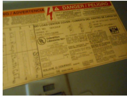
Unit E, 2 bedroom/1 bathroom - Kitchen electrical breaker
