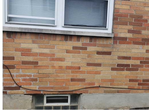
Update- North elevation minor cracking
