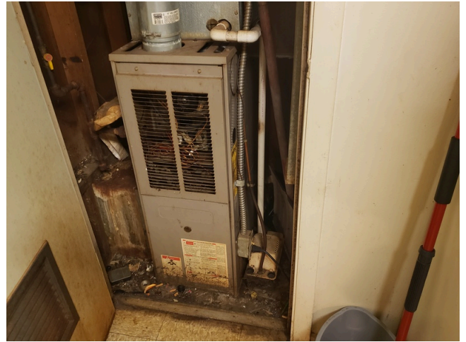
46. Update- Unit E, 2 bedroom/1 bathroom- Furnace
