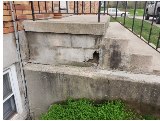
Update- Main entry stair- damaged concrete stair
