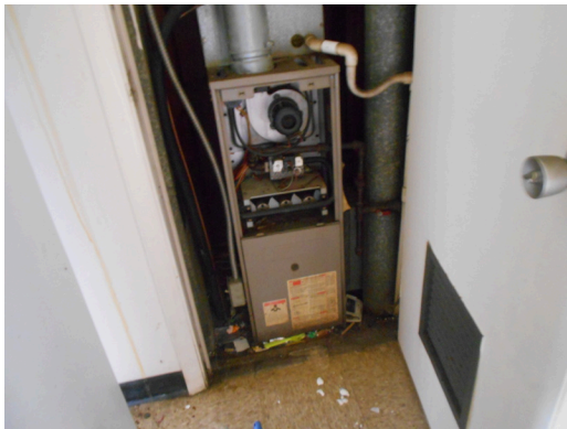
Unit A, 2 bedroom/1 bathroom, vacant - Furnace
