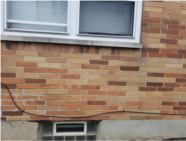
25. Update- North elevation minor cracking
