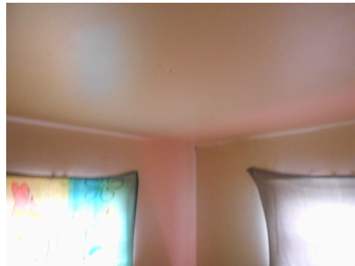
Unit E, 2 bedroom/1 bathroom - Bedroom 2 ceiling, no smoke detector
