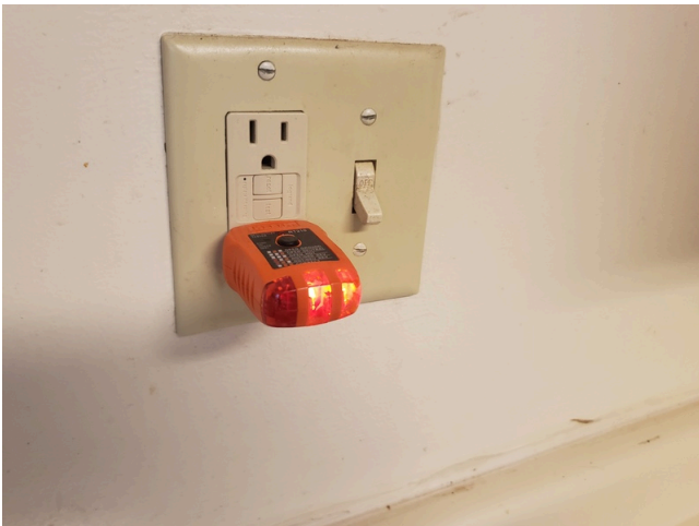
39. Update- Unit C, 2 bedroom/1 bathroom- GFCI outlet
