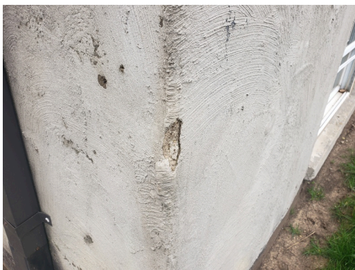
Update- West elevation cracking concrete
