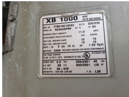
Update- HVAC 1.5 Ton- MFR- 2006
