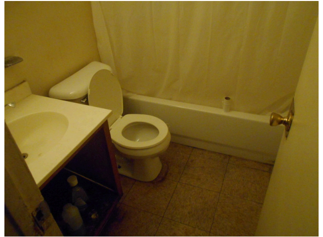
18. Unit E, 2 bedroom/1 bathroom - Bathroom, poor quality finishes
