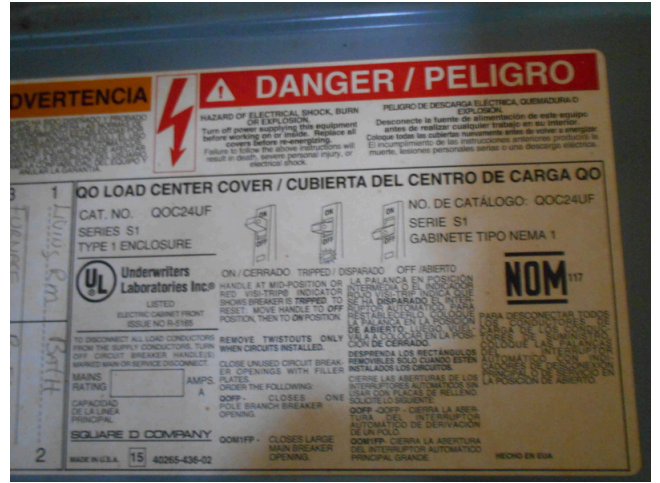
38. Unit A, 2 bedroom/1 bathroom, vacant - Kitchen electrical panel
