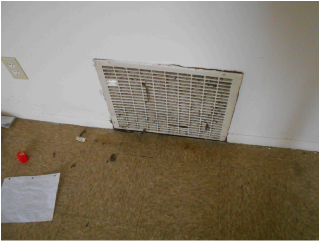
41. Unit A, 2 bedroom/1 bathroom, vacant - Vent
