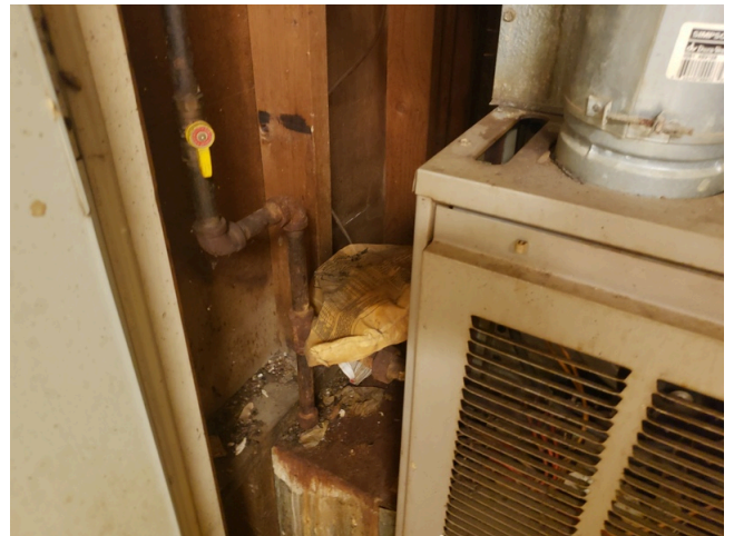
44. Update- Unit E, 2 bedroom/1 bathroom- Furnace- Rusty plumbing
