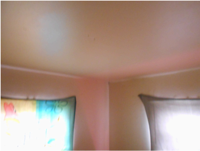
25. Unit E, 2 bedroom/1 bathroom - Bedroom 2 ceiling, no smoke detector
