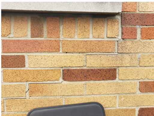
Update- North elevation minor cracking
