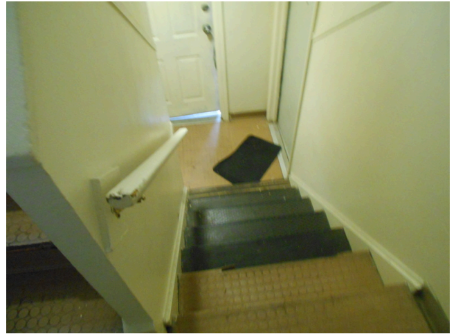
14. Common area stairwell, deteriorated
