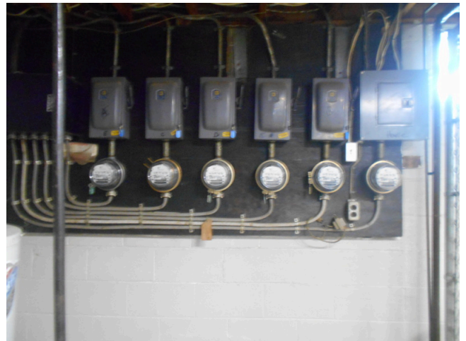
8. Tenant electrical breakers, old equipment
