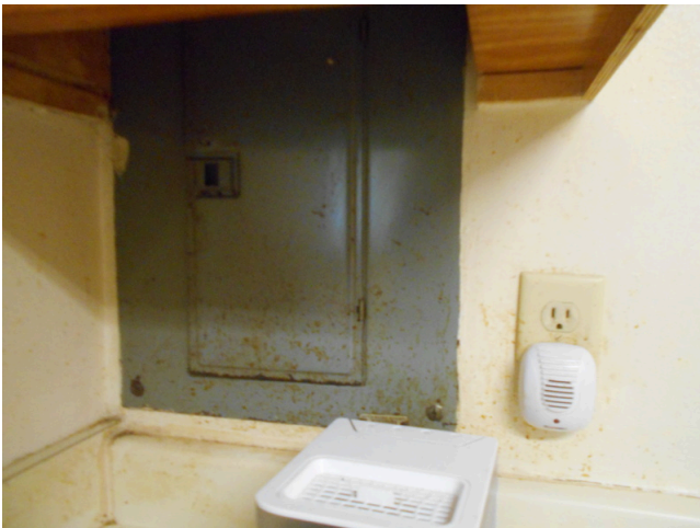
7. Unit E, 2 bedroom/1 bathroom - Kitchen electrical breaker, older/rusted
