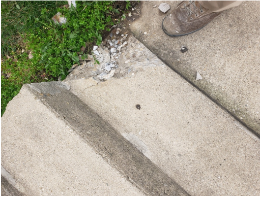
Update- Main entry stair- damaged concrete stair
