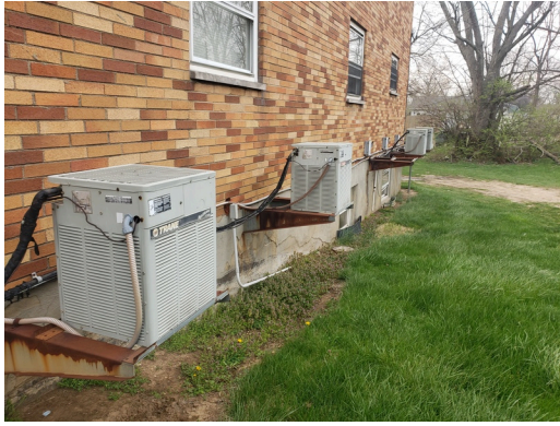
Update- HVAC Units Older
