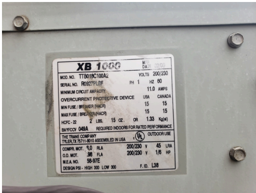
Update- HVAC 1.5 Ton- MFR- 2002
