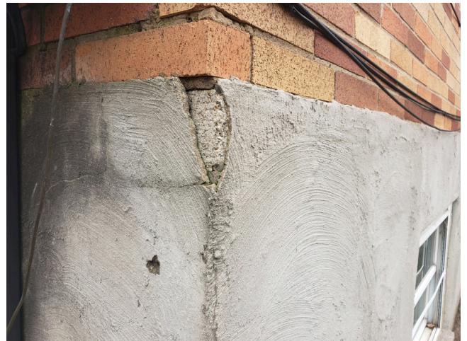
20. Update- West elevation cracking concrete
