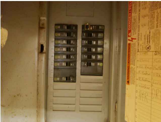
43. Update- Unit E, 2 bedroom/1 bathroom- Electrical Panel
