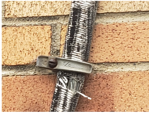
Update- Replace electrical service wire
