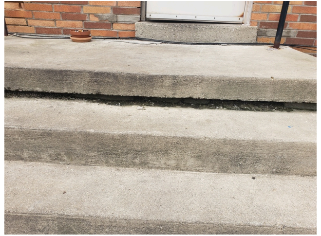
22. Update- Main entry stair- damaged concrete stair
