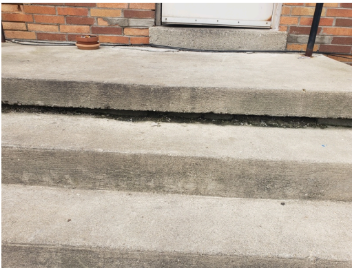
Update- Main entry stair- damaged concrete stair
