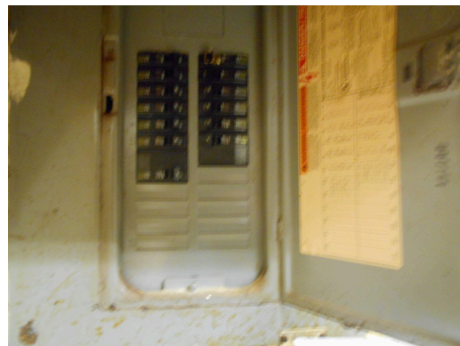
Unit E, 2 bedroom/1 bathroom - Kitchen electrical breaker
