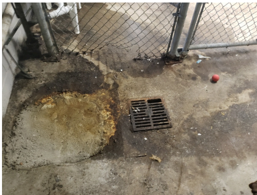
Deteriorated concrete slab at basement floor
