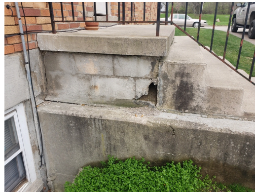
Update- Main entry stair- damaged concrete stair
