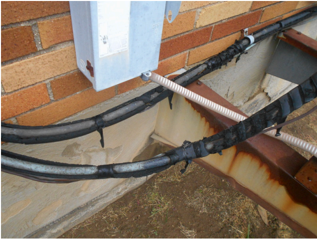
33. A/C units, deteriorated insulation line
