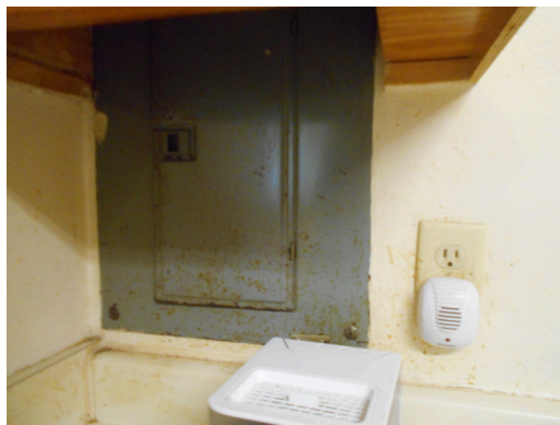
Unit E, 2 bedroom/1 bathroom - Kitchen electrical breaker, older/rusted
