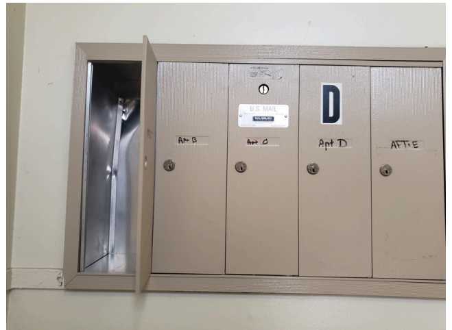
36. Update- Building interior damaged mailbox
