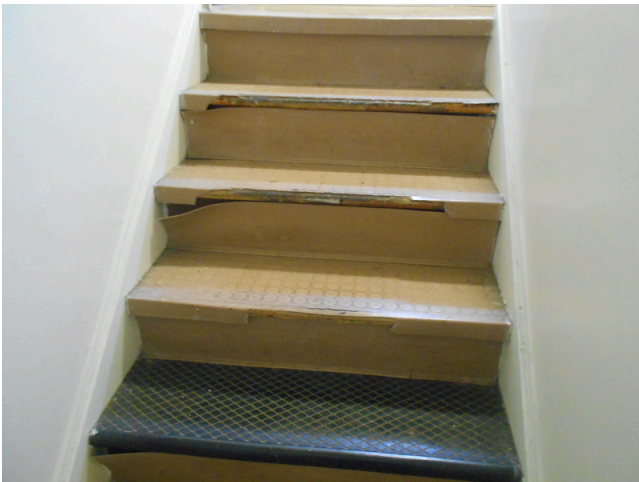
15. Common area stairwell, deteriorated
