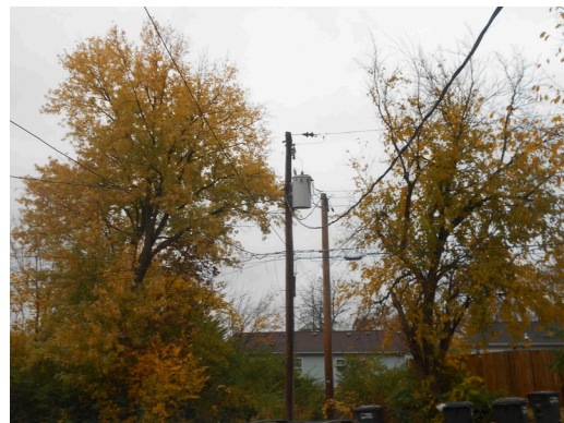
Pole mounted transformer
