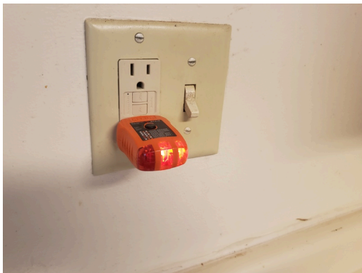
Update- Unit C, 2 bedroom/1 bathroom- GFCI outlet
