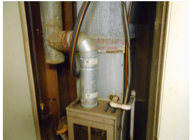
12. Unit E, 2 bedroom/1 bathroom - Furnace
