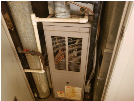
Update- Unit C, 2 bedroom/1 bathroom- Furnace
