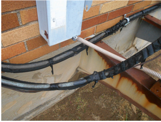
A/C units, deteriorated insulation line
