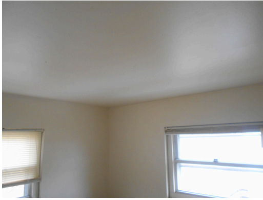
Unit A, 2 bedroom/1 bathroom, vacant - Bedroom 1 ceiling, no smoke detector
