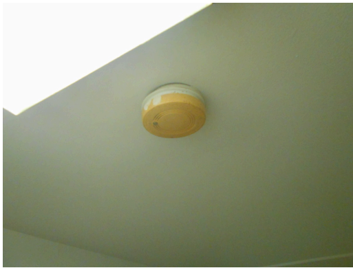
Common area stairwell smoke detector
