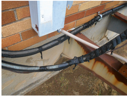
Areas of missing parging
