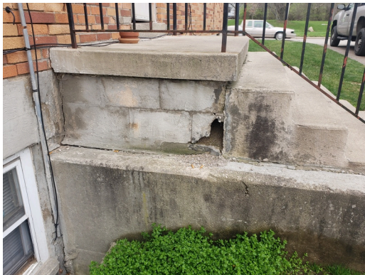
Update- Main entry stair- damaged concrete stair
