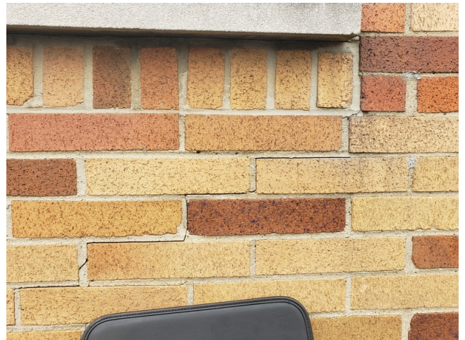
16. Update- North elevation minor cracking
