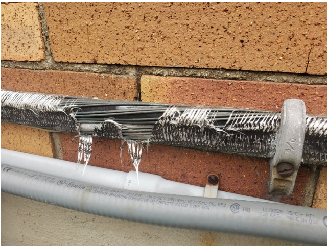
43. Update- Replace electrical service wire
