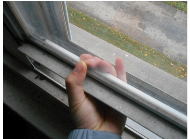
32. Unit A, 2 bedroom/1 bathroom, vacant - Vinyl window, single pane
