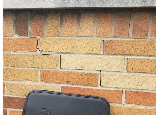
Update- North elevation minor cracking
