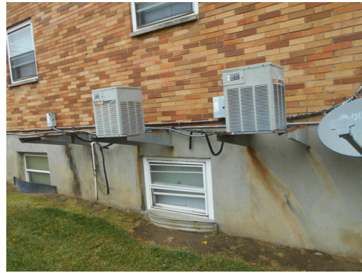
Areas of missing and cracking parging
