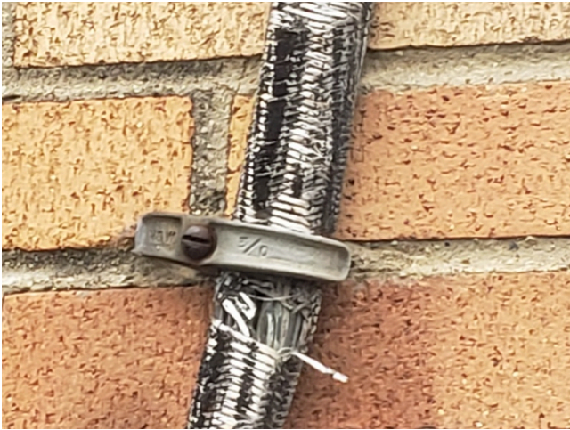
41. Update- Replace electrical service wire
