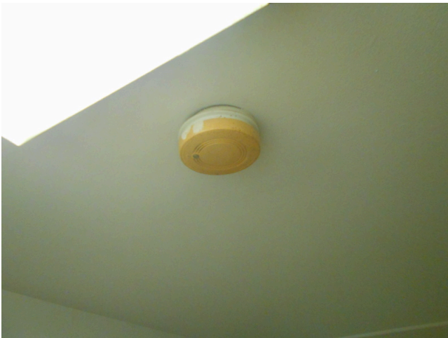
19. Common area stairwell smoke detector
