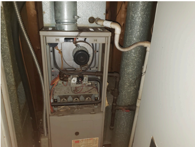
31. Update- Unit A, 2 bedroom/1 bathroom- Furnace
