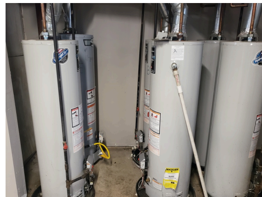
Update-Basement- Dwelling unit water heaters
