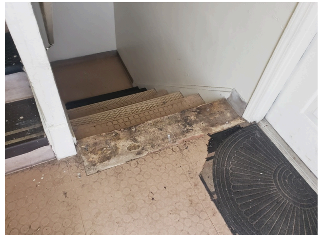
28. Update- Interior stair damaged thread
