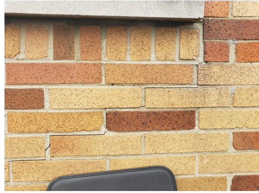
Update- North elevation minor cracking
