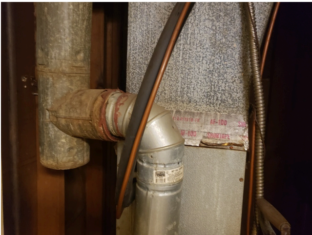
51. Update- Unit E, 2 bedroom/1 bathroom- Furnace- Vent
