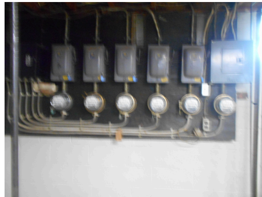
Tenant electrical meters & disconnects
