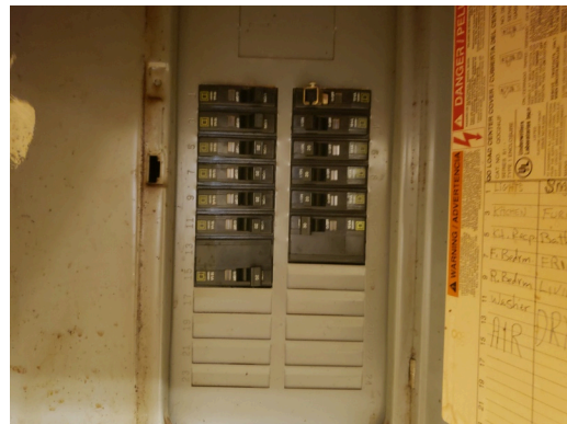
Update- Unit E, 2 bedroom/1 bathroom- Electrical Panel
