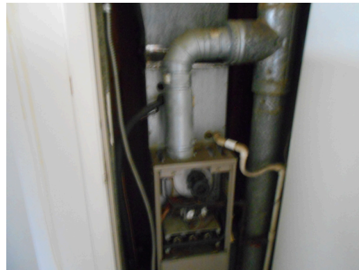
Unit A, 2 bedroom/1 bathroom, vacant - Furnace
