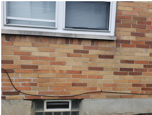
Update- North elevation minor cracking
