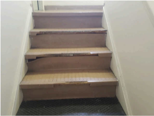
9. Update- Interior stair damaged threads
