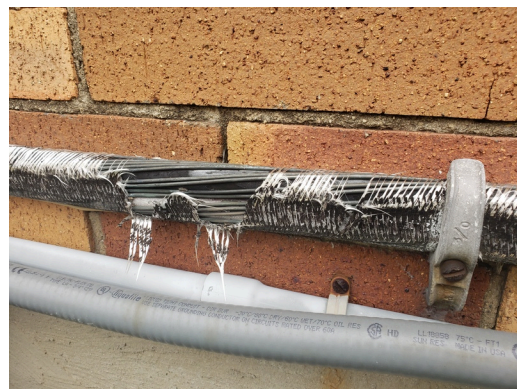
Update- Replace electrical service wire
