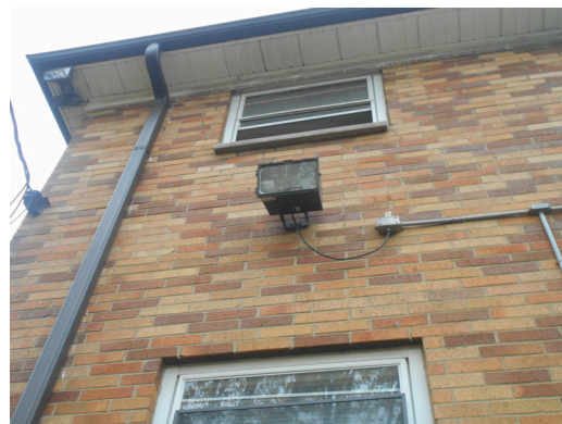
Building mounted lighting
