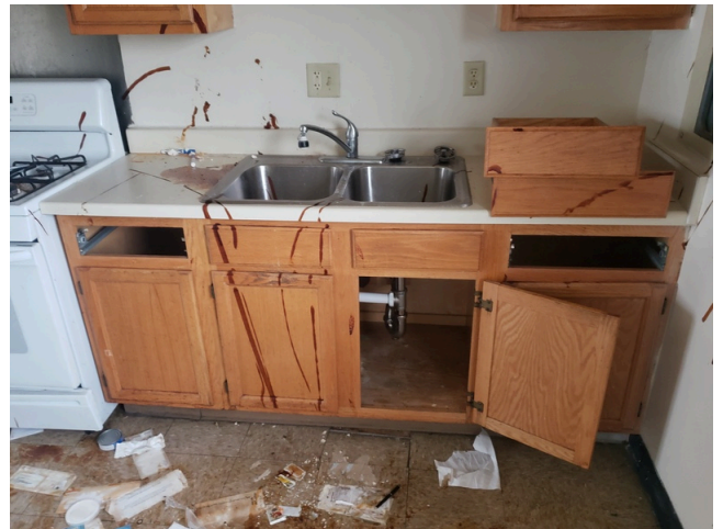
24. Update- Unit A, 2 bedroom/1 bathroom- Kitchen- Damaged cabinets
