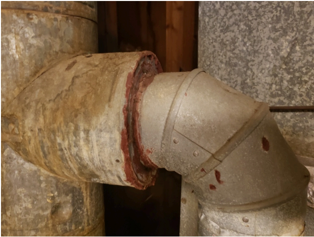
41. Update- Unit C, 2 bedroom/1 bathroom- Furnace
