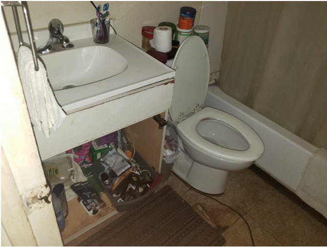
29. Update- Unit B, 2 bedroom/1 bathroom- Bathroom- Damaged vanity
