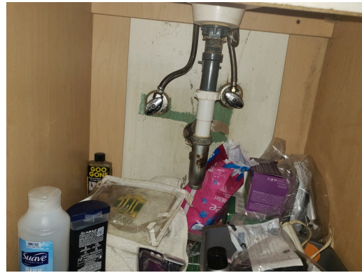
Update- Unit B, 2 bedroom/1 bathroom- Bathroom- Damaged vanity
