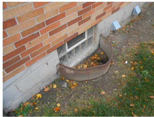
Basement window well
