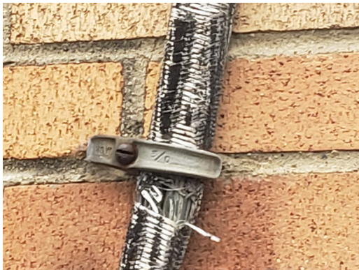
Update- Replace electrical service wire
