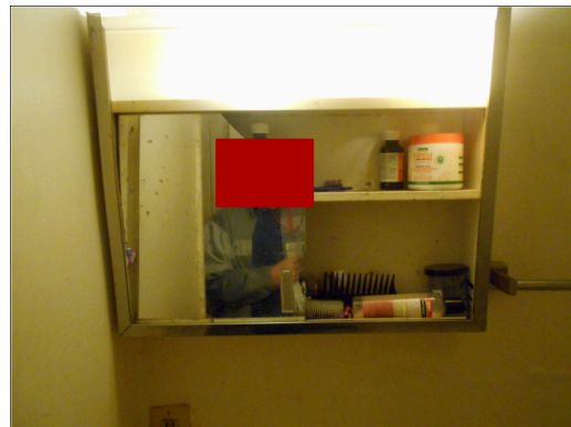
Unit E, 2 bedroom/1 bathroom - Bathroom medicine cabinet, damaged glass, poor quality finishes
