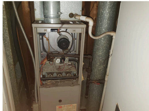
Update- Unit A, 2 bedroom/1 bathroom- Furnace
