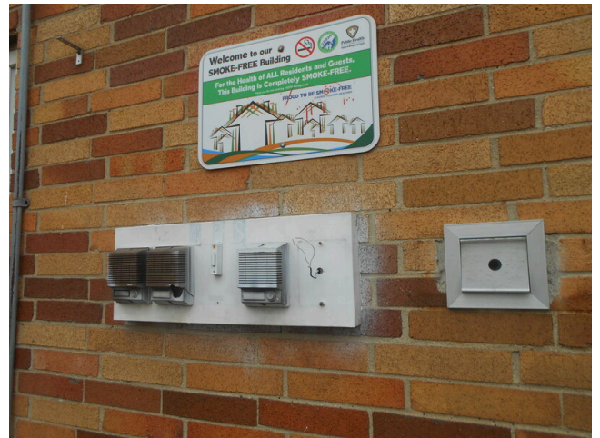
44. Building intercom, reported inoperable
