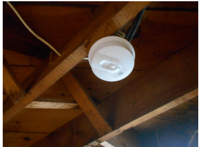
4. Common area laundry room smoke detector
