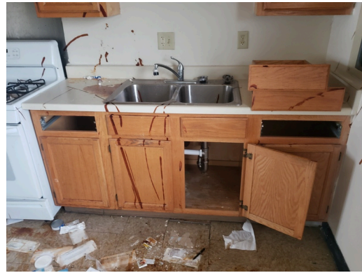
Update- Unit A, 2 bedroom/1 bathroom- Kitchen- Damaged cabinets
