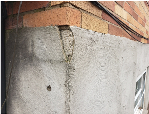
Update- West elevation cracking concrete
