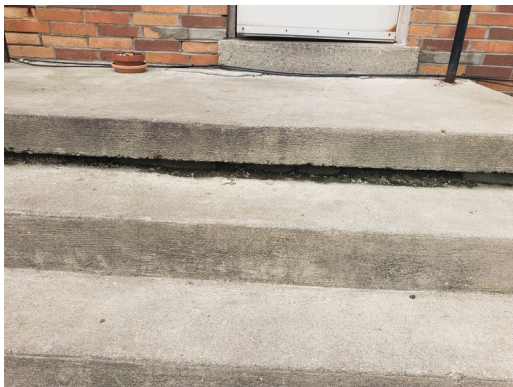
Update- Main entry stair- damaged concrete stair
