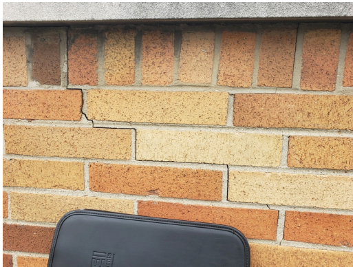
Update- North elevation minor cracking
