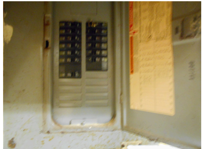
8. Unit E, 2 bedroom/1 bathroom - Kitchen electrical breaker
