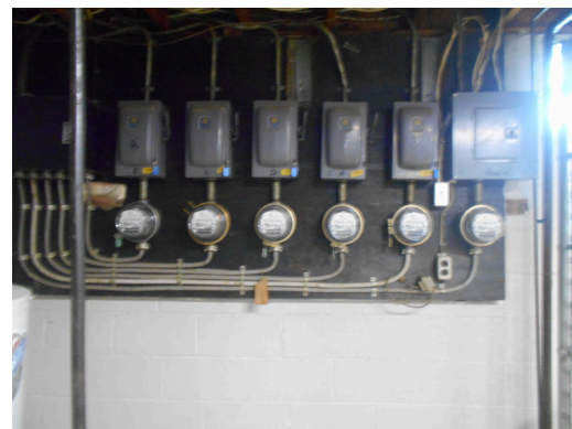
Tenant electrical breakers, old equipment
