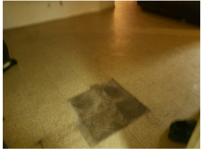
42. Update- Unit E, 2 bedroom/1 bathroom- Living room- damaged VCT
