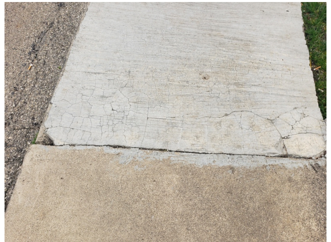
12. Update- Repair cracking concrete sidewalk
