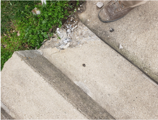
Update- Main entry stair- damaged concrete stair
