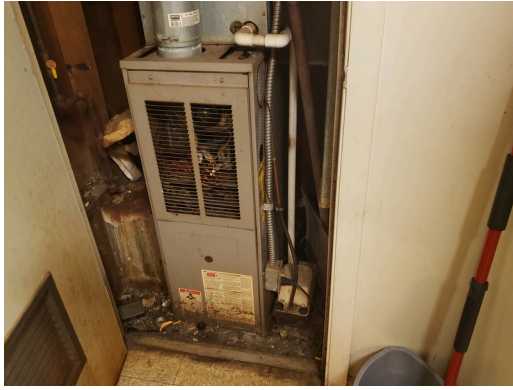
Update- Unit E, 2 bedroom/1 bathroom- Furnace
