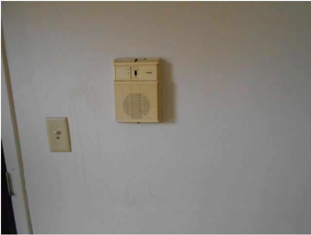
33. Unit A, 2 bedroom/1 bathroom, vacant - Intercom, disconnected from previous door intercom system
