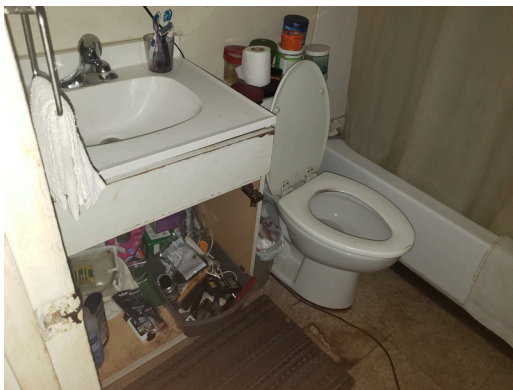
Update- Unit B, 2 bedroom/1 bathroom- Bathroom- Damaged vanity
