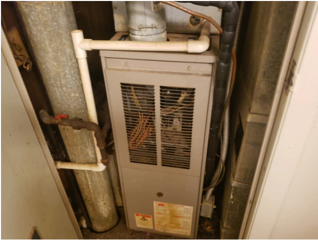
9. Update- Unit C, 2 bedroom/1 bathroom- Furnace
