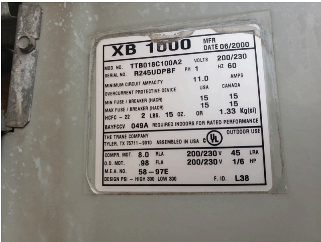
31. Update- HVAC 1.5 Ton- MFR- 2006
