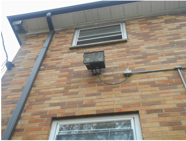
37. Building mounted lighting
