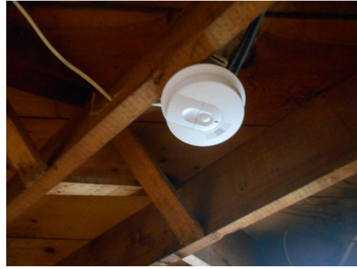
Common area laundry room smoke detector
