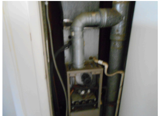
40. Unit A, 2 bedroom/1 bathroom, vacant - Furnace
