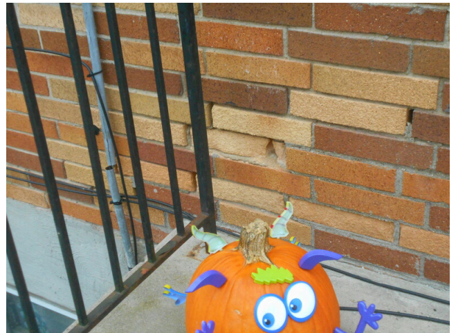
48. Brick facade, requires repointing
