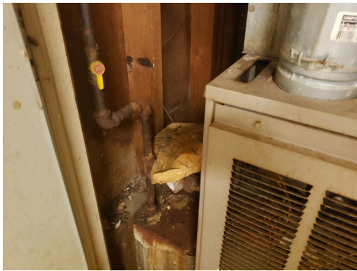
Update- Unit E, 2 bedroom/1 bathroom- Furnace- Rusty plumbing
