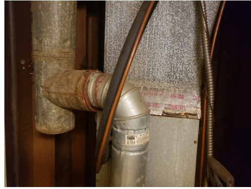
Update- Unit E, 2 bedroom/1 bathroom- Furnace- Vent
