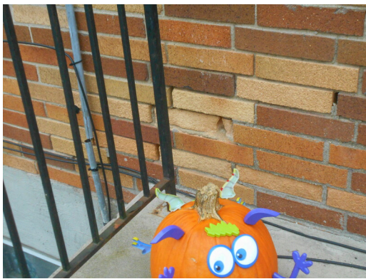
Brick facade, requires repointing
