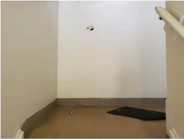
33. Update- Interior stair damaged drywall
