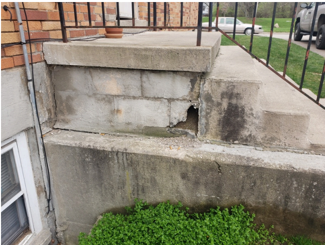
27. Update- Main entry stair- damaged concrete stair
