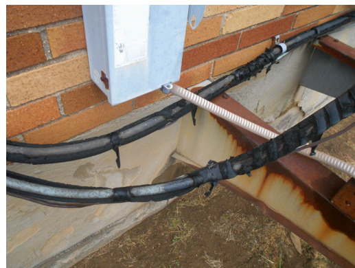
A/C units, deteriorated insulation line
