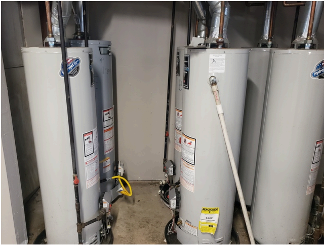
1. Update-Basement- Dwelling unit water heaters
