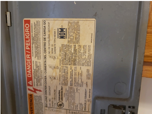
35. Update- Unit C, 2 bedroom/1 bathroom- Electrical panel
