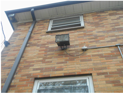
Building mounted lighting
