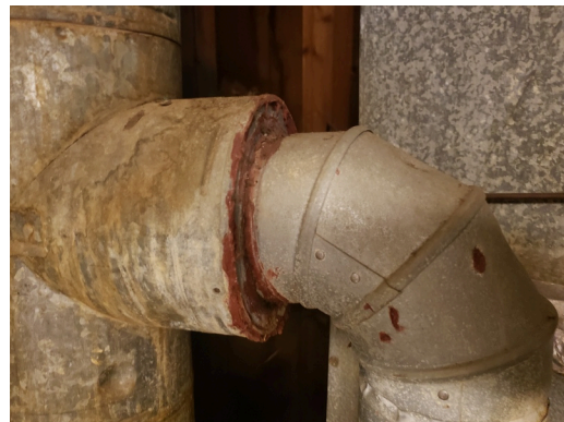
Update- Unit C, 2 bedroom/1 bathroom- Furnace
