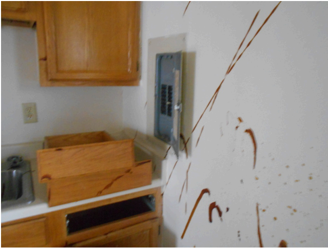
37. Unit A, 2 bedroom/1 bathroom, vacant - Kitchen electrical panel
