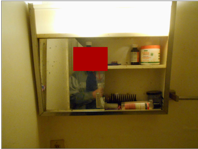
21. Unit E, 2 bedroom/1 bathroom - Bathroom medicine cabinet, damaged glass, poor quality finishes
