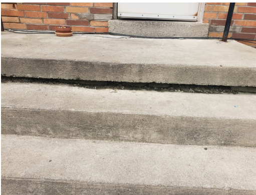
Update- Main entry stair- damaged concrete stair
