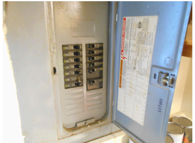
56. Unit C, 2 bedroom/1 bathroom - Electrical breaker
