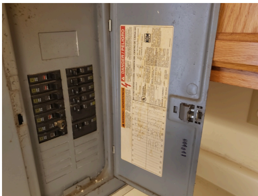
Update- Unit C, 2 bedroom/1 bathroom- Electrical panel
