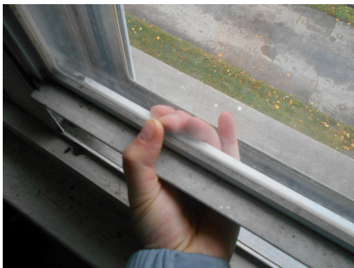
Unit A, 2 bedroom/1 bathroom, vacant - Vinyl window, single pane
