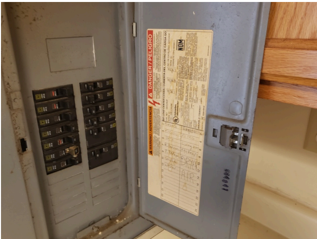
3. Update- Unit C, 2 bedroom/1 bathroom- Electrical panel
