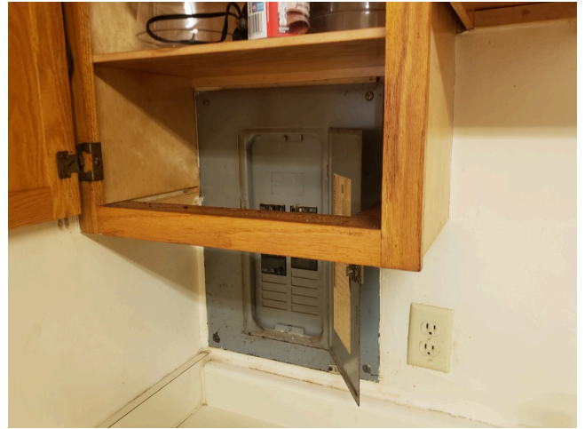
50. Update- Unit E, 2 bedroom/1 bathroom- Electrical Panel
