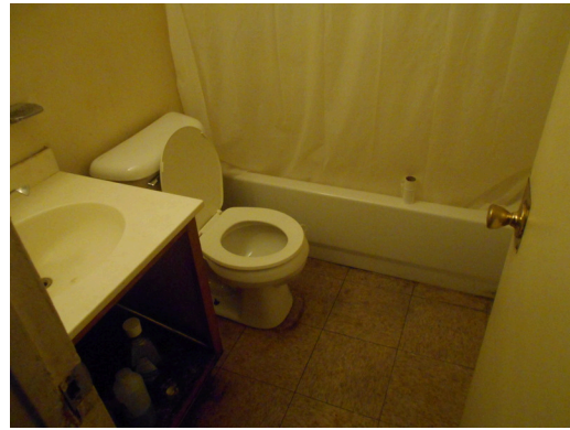
Unit E, 2 bedroom/1 bathroom - Bathroom, poor quality finishes
