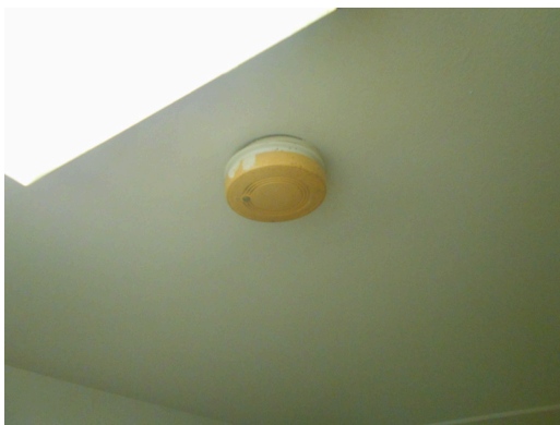
Common area stairwell smoke detector
