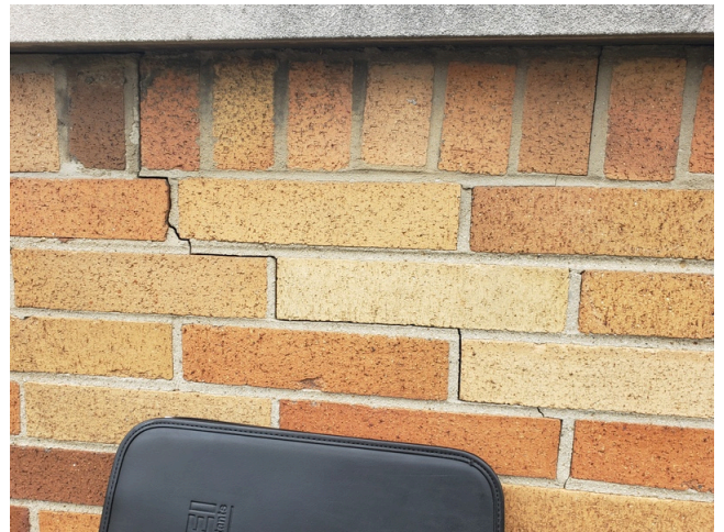
24. Update- North elevation minor cracking
