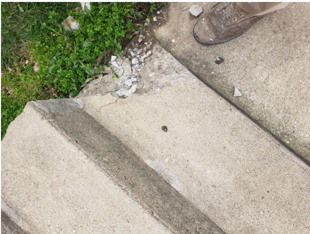
11. Update- Main entry stair- damaged concrete stair
