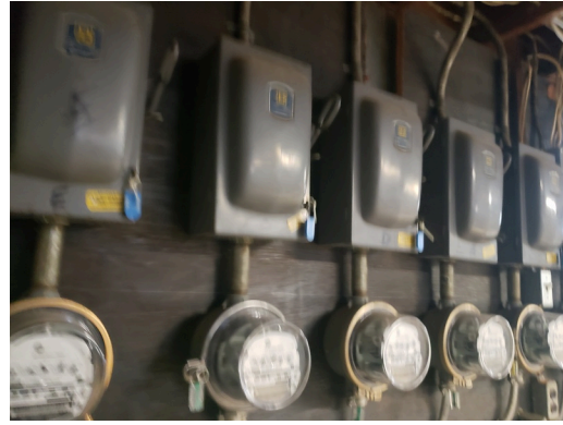
Unit meters & disconnects
