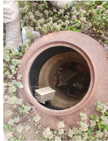
14. Update- Sump pump not in use
