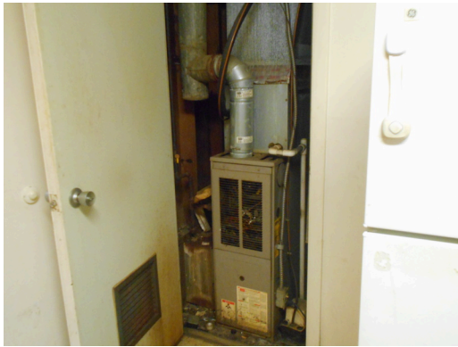
Unit E, 2 bedroom/1 bathroom - Furnace, older unit
