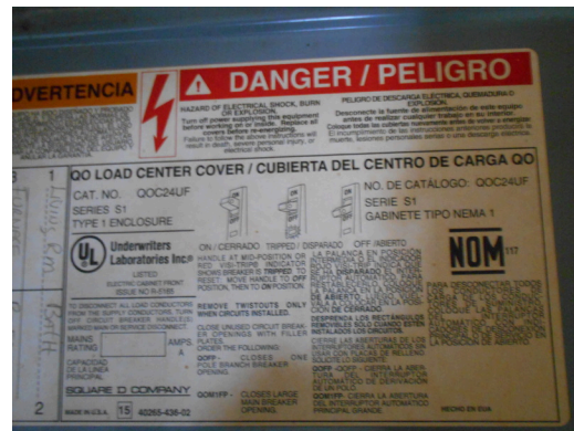
Unit A, 2 bedroom/1 bathroom, vacant - Kitchen electrical panel
