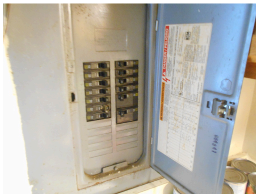
Unit C, 2 bedroom/1 bathroom - Electrical breaker
