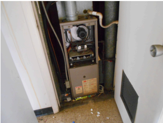
39. Unit A, 2 bedroom/1 bathroom, vacant - Furnace
