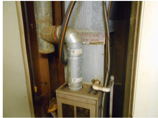
Unit E, 2 bedroom/1 bathroom - Furnace
