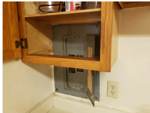
Update- Unit E, 2 bedroom/1 bathroom- Electrical Panel
