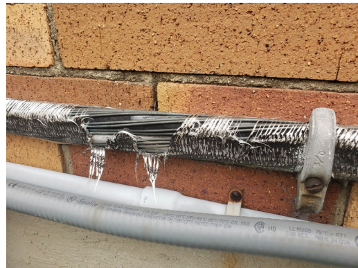
Update- Replace electrical service wire
