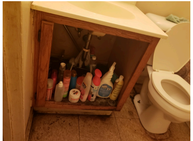
48. Update- Unit E, 2 bedroom/1 bathroom- Bathroom- Damaged vanity
