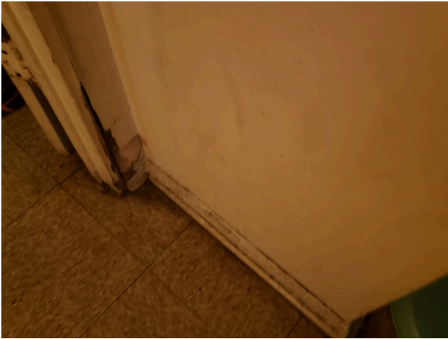
1. Update- Unit E, 2 bedroom/1 bathroom- Bedroom- Damaged drywall
