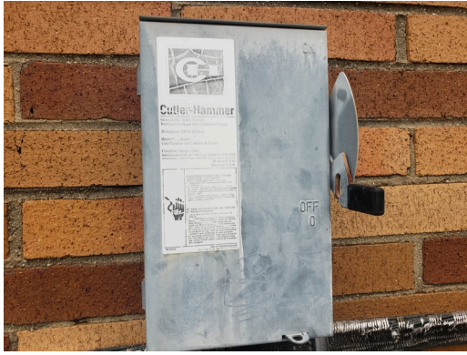
Main service disconnect
