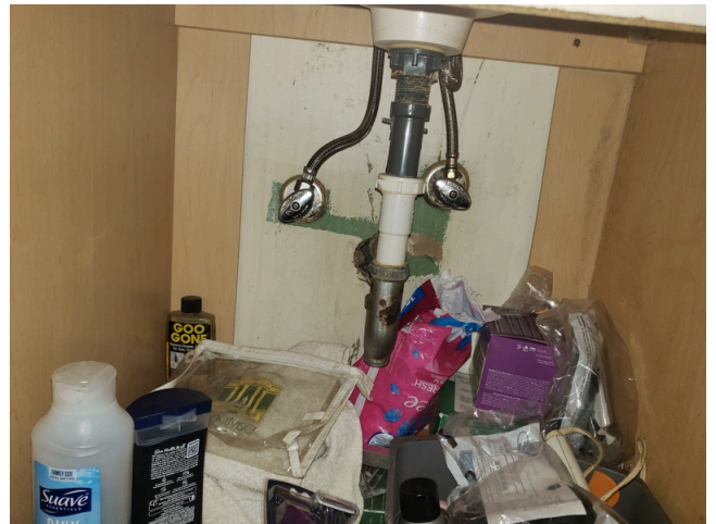
16. Update- Unit B, 2 bedroom/1 bathroom- Bathroom- Damaged vanity
