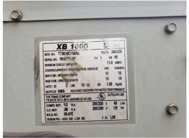
38. Update- HVAC 1.5 Ton- MFR- 2002
