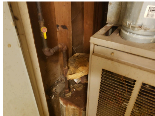
Update- Unit E, 2 bedroom/1 bathroom- Furnace- Rusty plumbing
