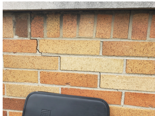
Update- North elevation minor cracking
