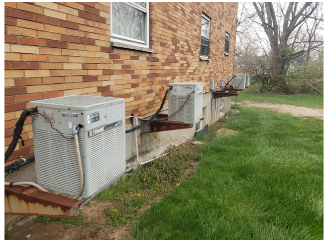
32. Update- HVAC Units Older
