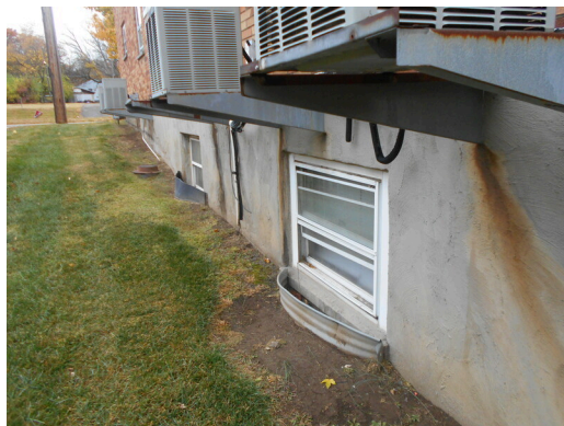
Areas of missing and cracking parging
