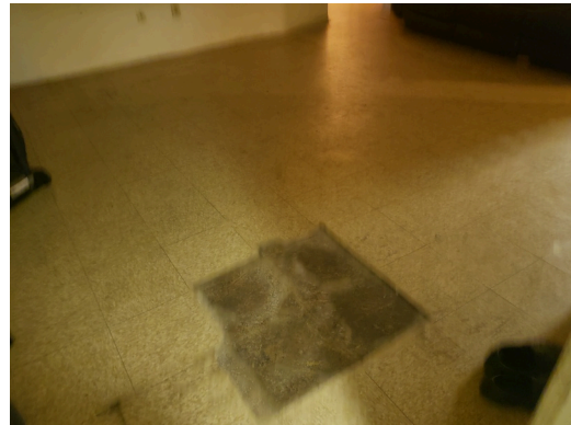
Update- Unit E, 2 bedroom/1 bathroom- Living room- damaged VCT
