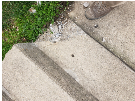
Update- Main entry stair- damaged concrete stair
