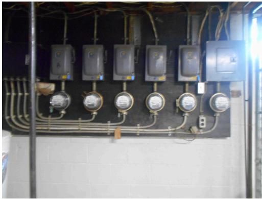
Tenant electrical breakers, old equipment
