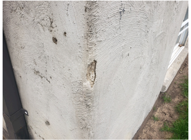
10. Update- West elevation cracking concrete
