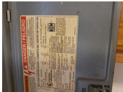
Update- Unit C, 2 bedroom/1 bathroom- Electrical panel
