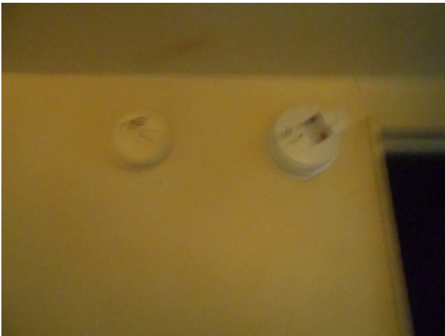
15. Unit E, 2 bedroom/1 bathroom - Living area smoke detectors
