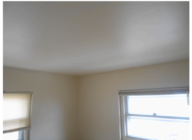
44. Unit A, 2 bedroom/1 bathroom, vacant - Bedroom 1 ceiling, no smoke detector
