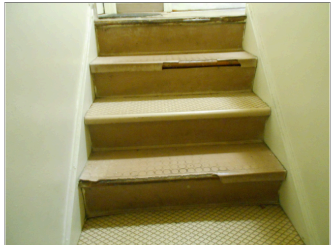
12. Common area stairwell, deteriorated
