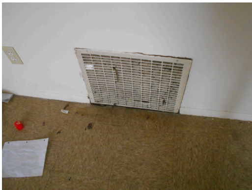
Unit A, 2 bedroom/1 bathroom, vacant - Vent
