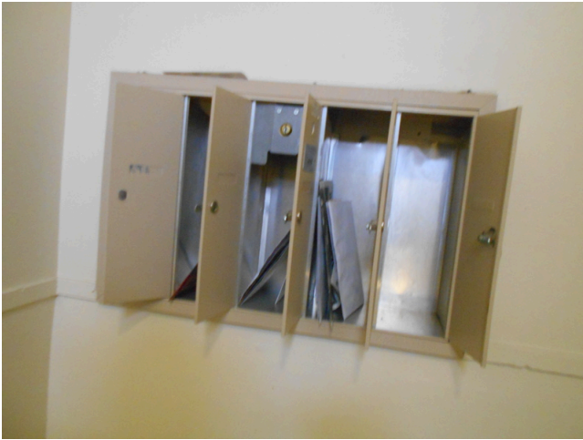
13. Common area stairwell mailboxes
